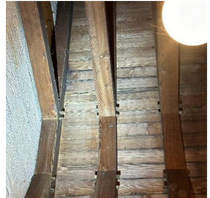
Figure 16 – Porch ceiling – rotten board
