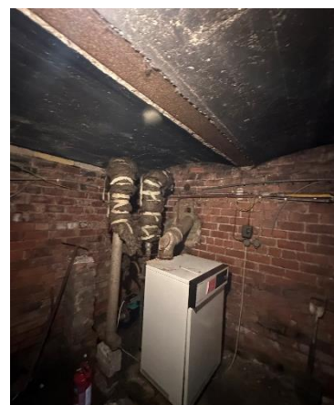
Figure 15- Boiler room – rusted beam
