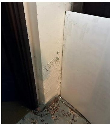
Figure 24- Damp near lobby door
