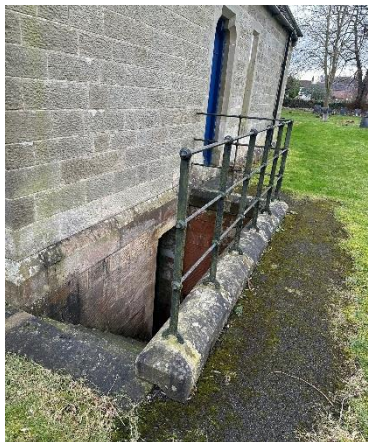
Figure 14- Boiler Rm Guarding
