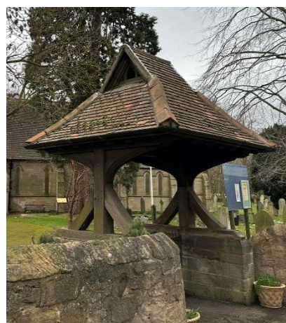
Figure 29 – Collapsed wall to W
