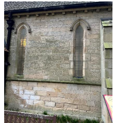
Figure 8 – S Nave erosion and lancets with cracks above
