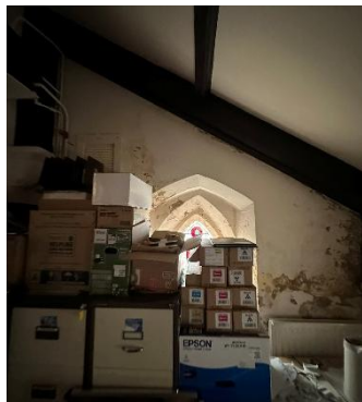
Figure 60 – damp to E wall
