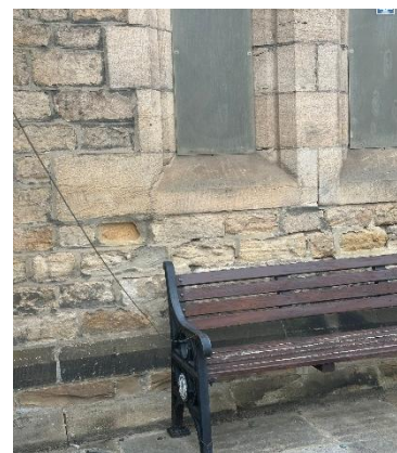
Figure 19 – second bay erosion
