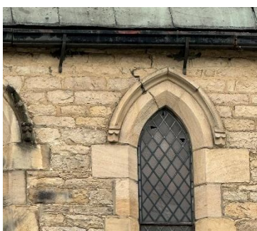
Figure 18 – Crack above lancet
