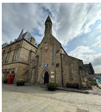
Figure 37 – cracking to W wall
