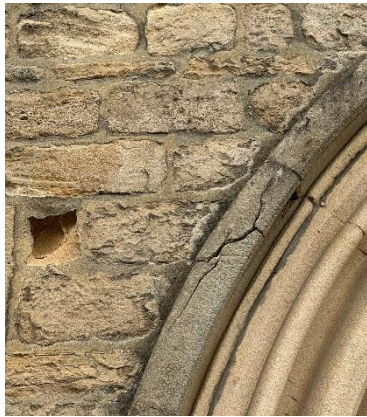
Figure 21 – Hoodmould and erosion
