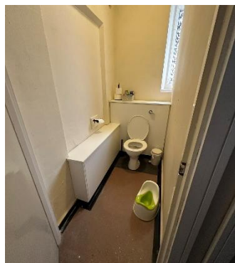
Figure 57 – WC area where floor had temp repairs
