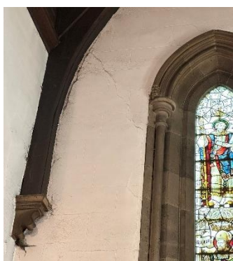
Figure 48 – crack to LHS of E and rafter closest to E wall
