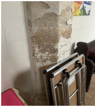
Figure 56 – Columns with damp issues
