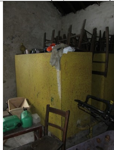
Rusty oil tanks (8.1)
