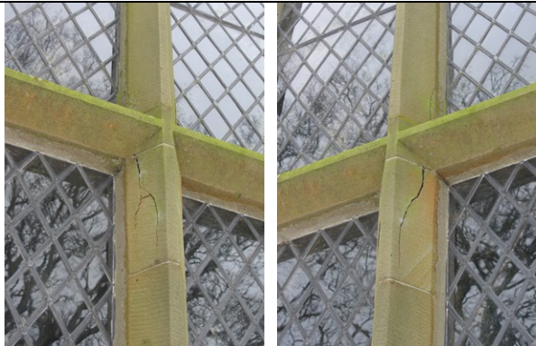
Nave north window n(v) – cracks to mullions (6.7)
