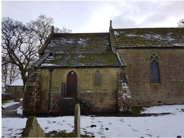
Moss on roofs/ slipped slates (6.1)
