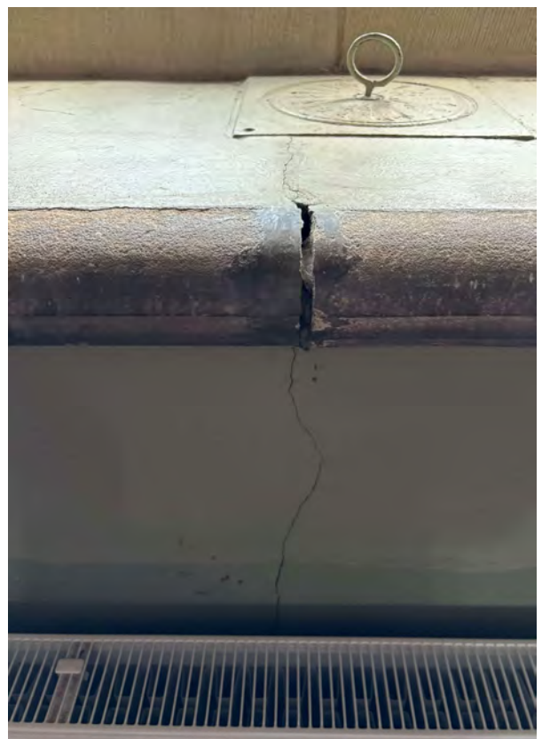
Evident crack to window cill.
