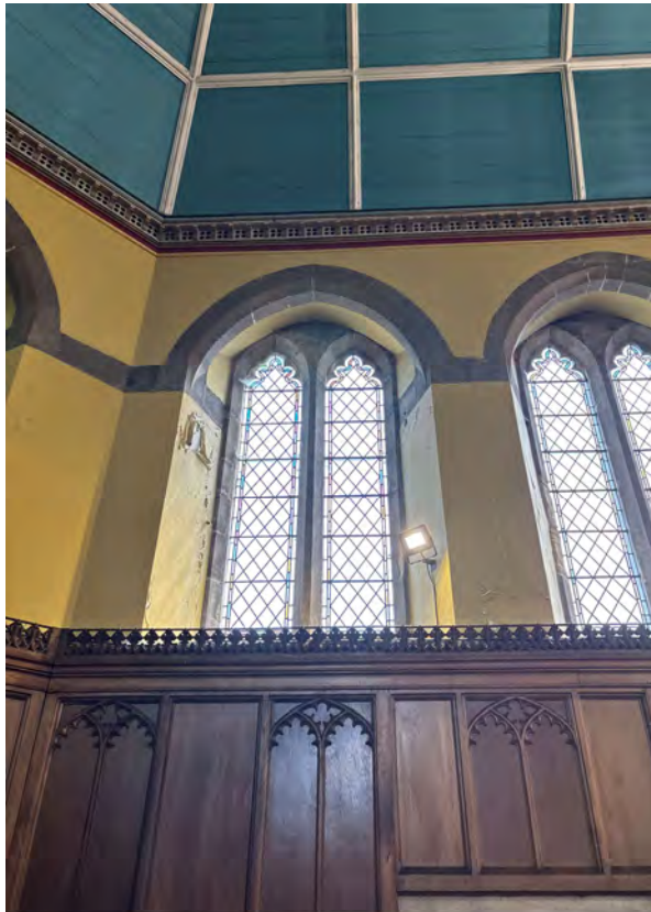
Some flaking and blistering of paint to some window surrounds.
