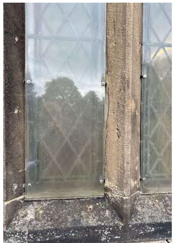
W17 – Deterioration to mullion.
