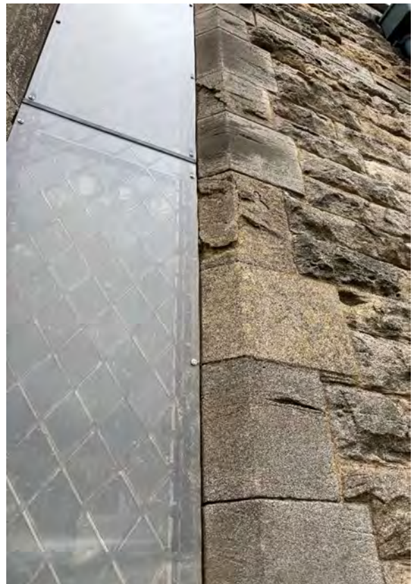
W9 – Significant deterioration of stone surround.
