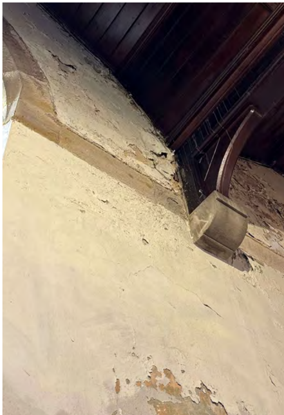
Significant flaking of paint also visible at high level to W8/W9 of North Transept.
