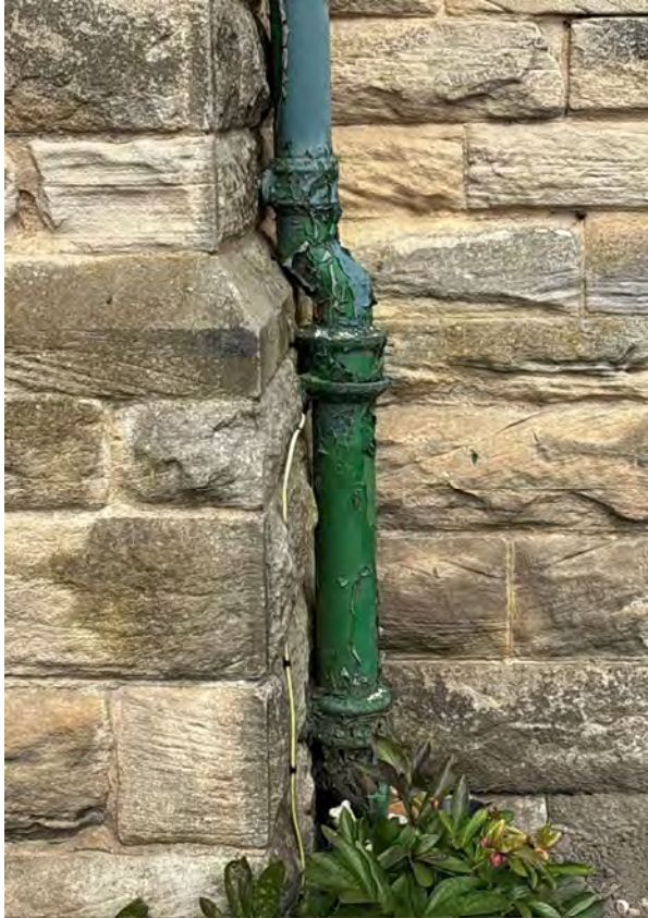
Evidence of paint failure to downpipes.
