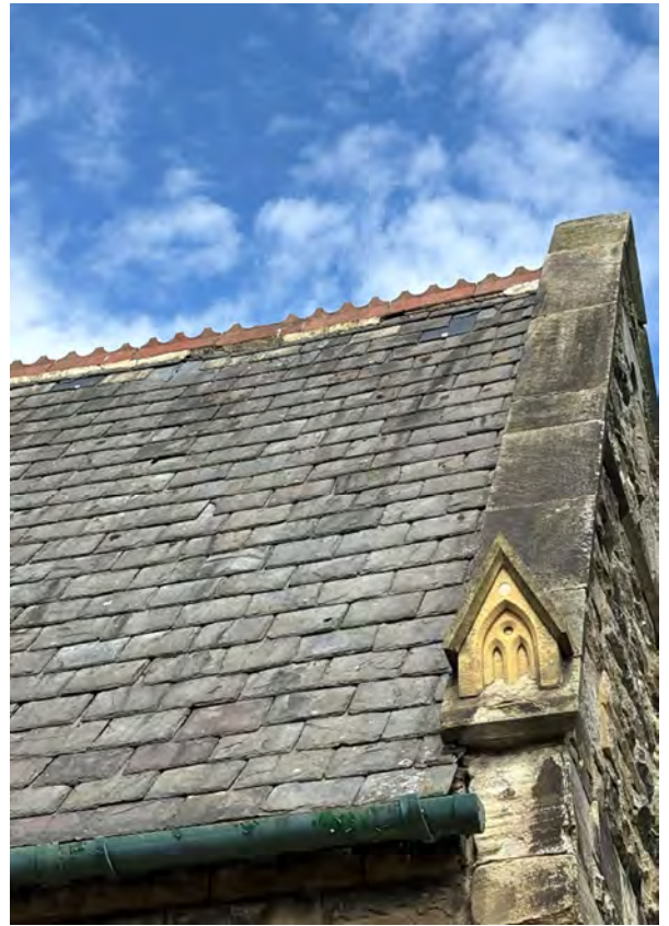
Loss of mortar bedding to ridge tiles.
