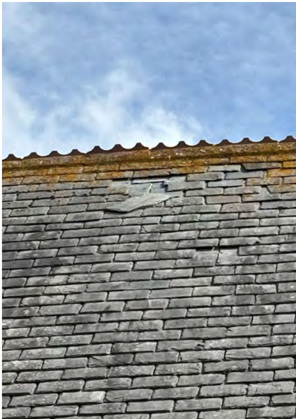
Example areas of damage to North Roof
