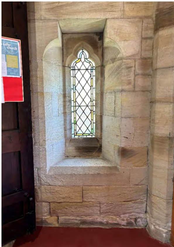
Deterioration to lower two courses.
