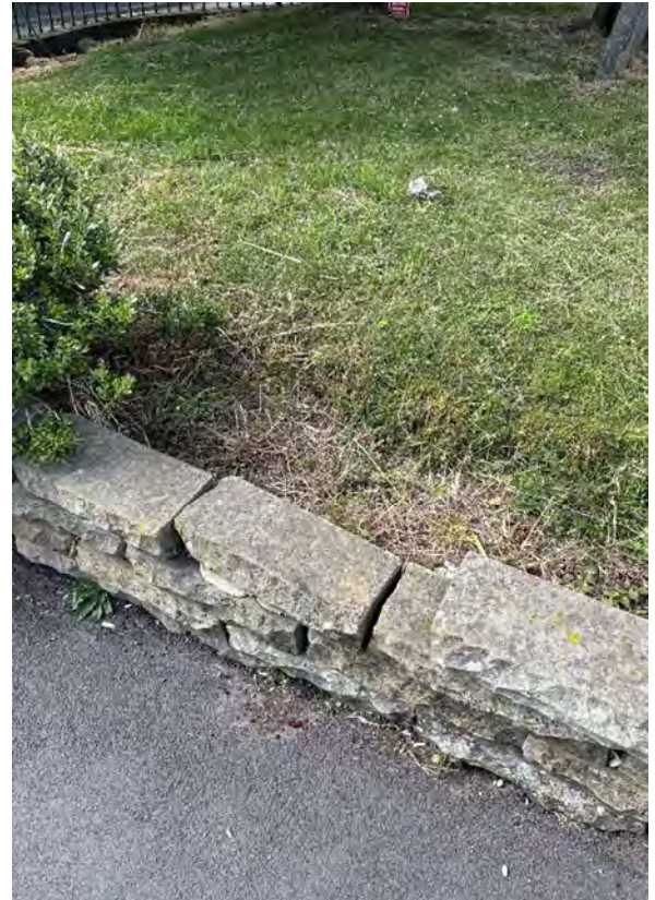
Some loss of pointing to low level kerb to path towards church.
