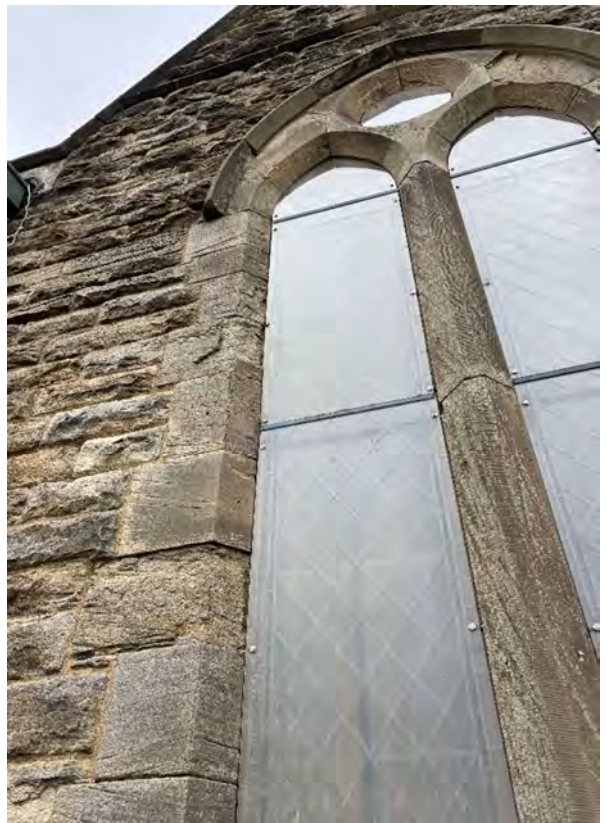
W8 – Various locations of deterioration to stone surround.
