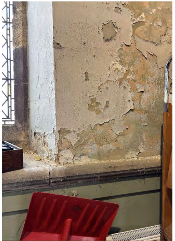
Significant flaking of paint and damage to plaster to walls of W8 & W9 North Transept
