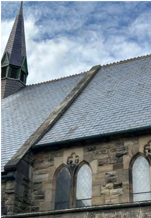
South roof in better condition however still some slipped / missing / broken tiles
