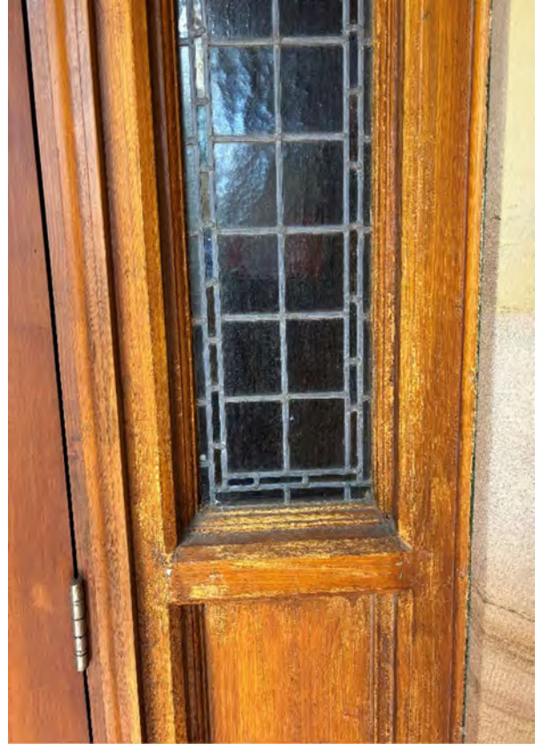
Minor flaking of paint to entrance doors.
