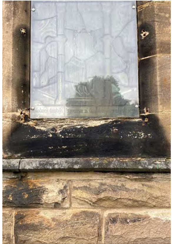
W21 – Significant deterioration of cills.
