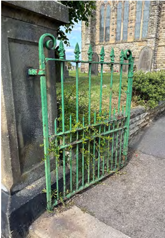
Flaking paint to entrance gates.
