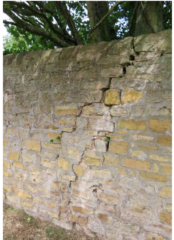
Area of wall cracking due to tree behind.
