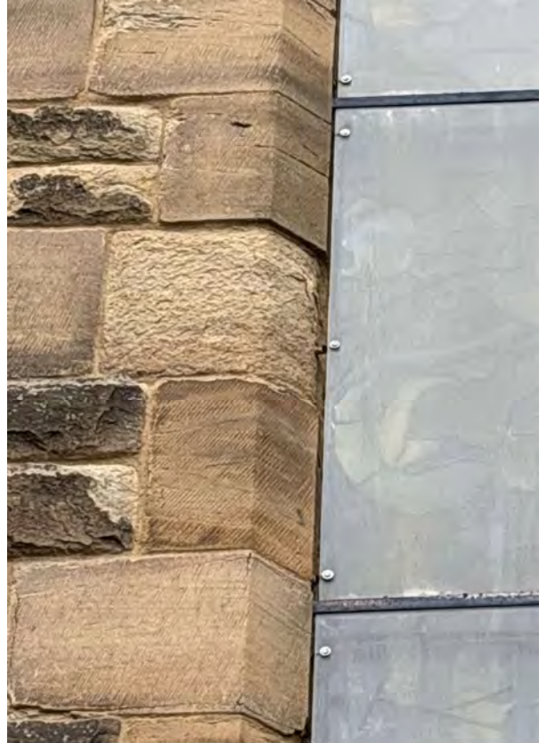
W1 – Deterioration of stone face.
