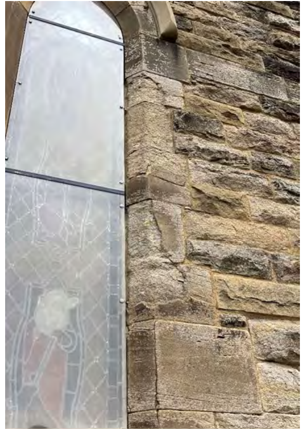
W18 – Significant deterioration of stone surround.
