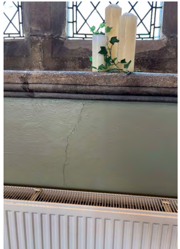
Example cracks to plaster work above radiators within the nave.
