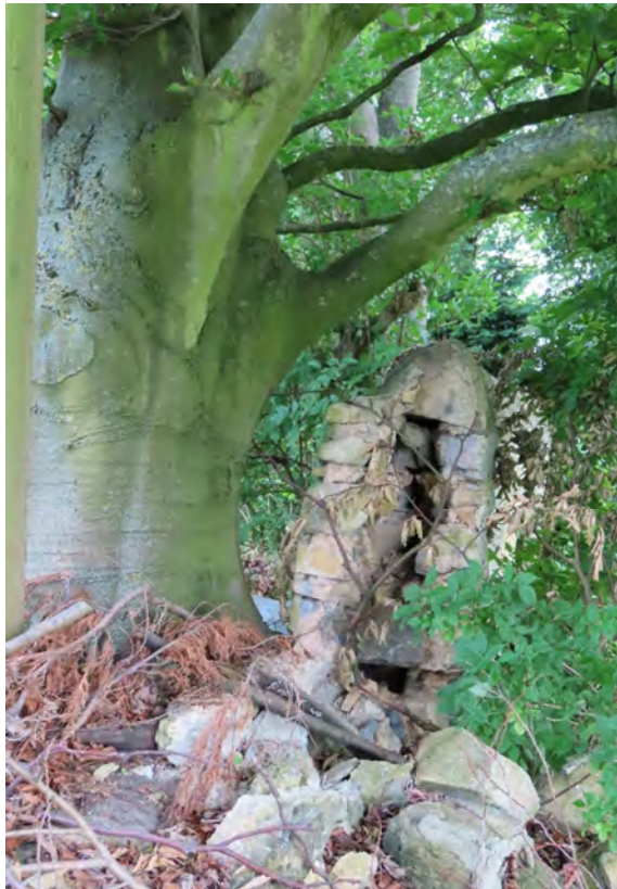
Proximity of tree behind fallen wall.
