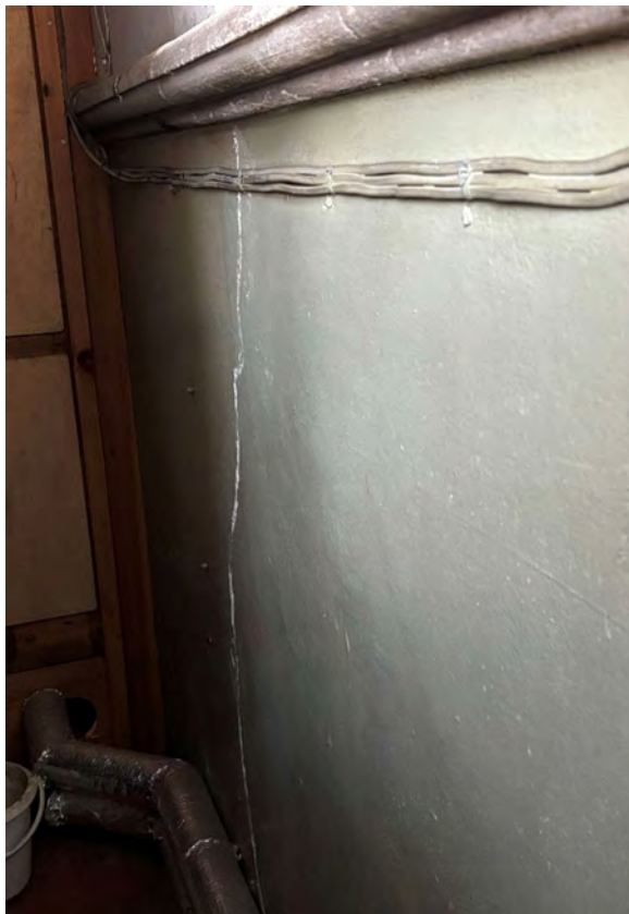
Crack below window cill of W7.
