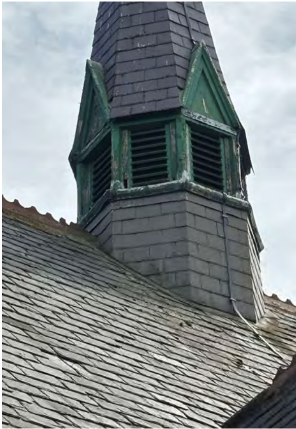
Fleche appears to be deteriorating with flaking paint / timber rot visible.
