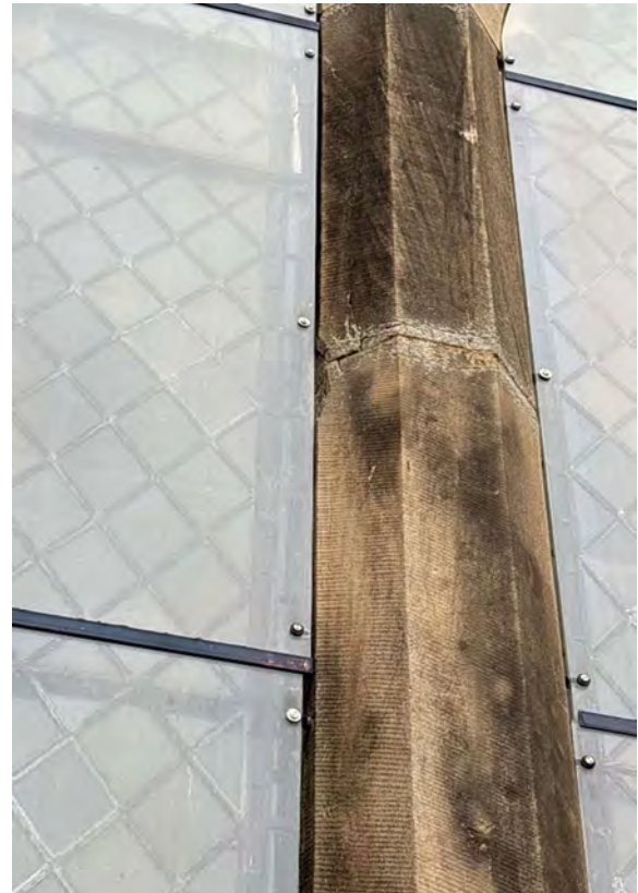
W22 – Some deterioration to mullion.
