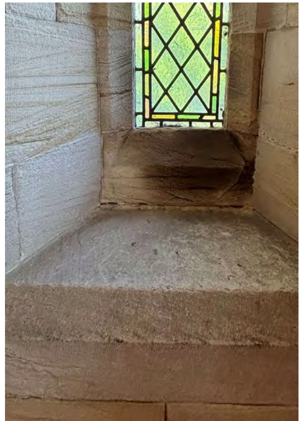
Evidence of cracking to stone cills.
