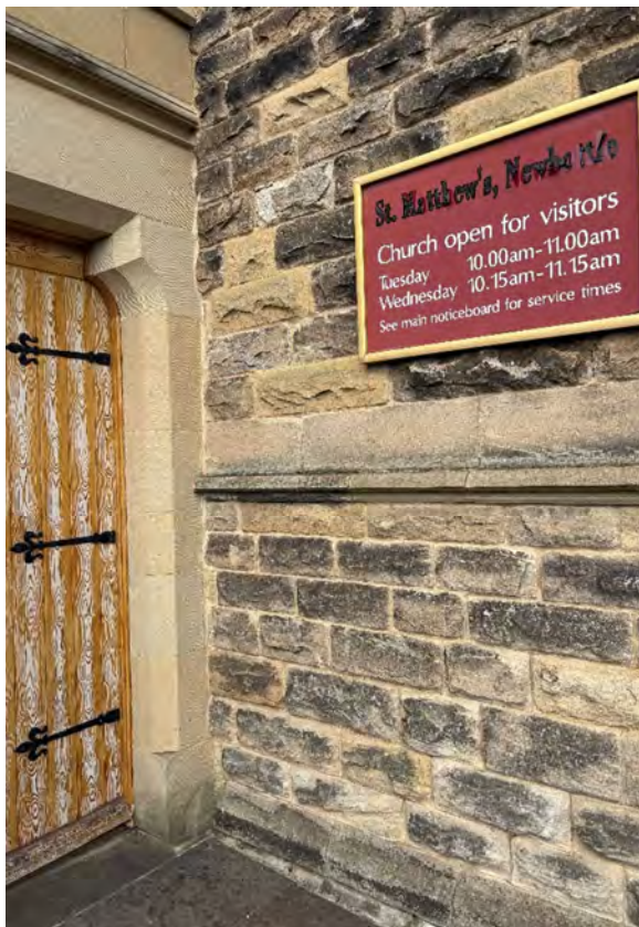
Signage within proximity of entrance showing failed lettering.
