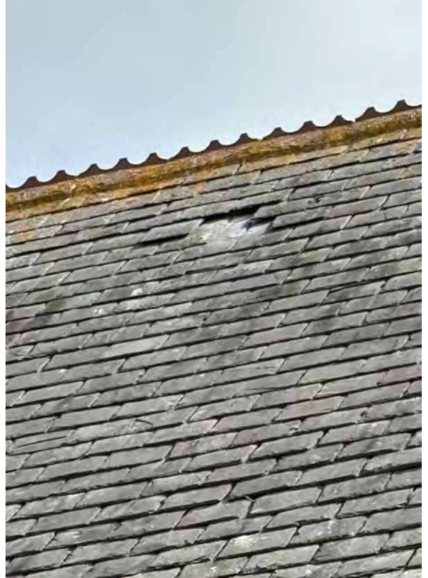
Example areas of damage to North Roof
