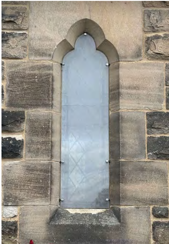
W25 – General overview of window. Some significant deterioration to cill.
