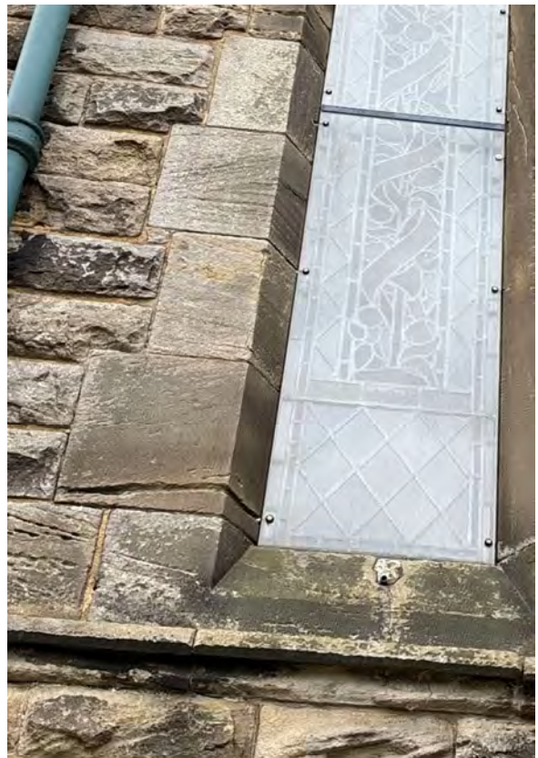
W12a – Deterioration visible at lower and upper areas of stone surround.
