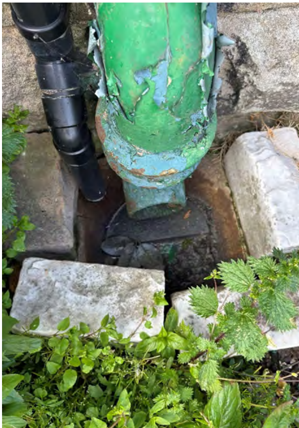
Evidence of blockage to drains.
