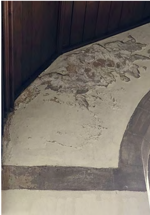
Significant flaking and blistering of paint to South wall with damage to plaster behind.
