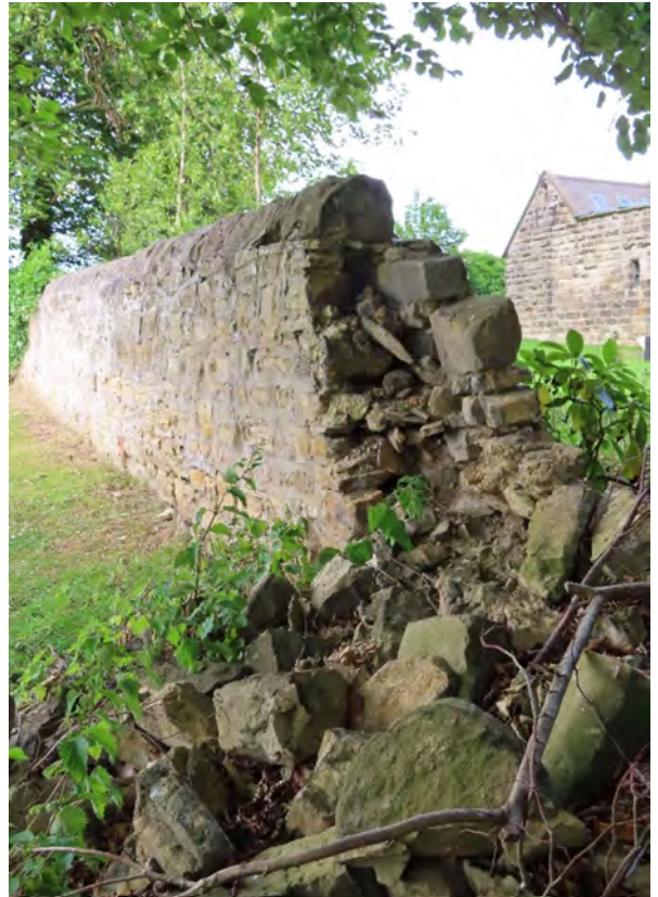
Area of fallen boundary wall to East.
