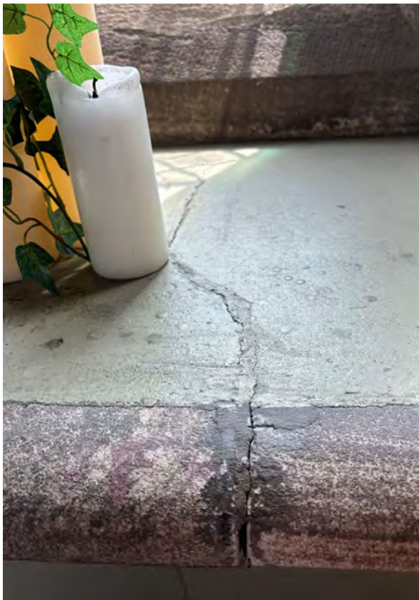
Example of historic cracking to cill in Nave
