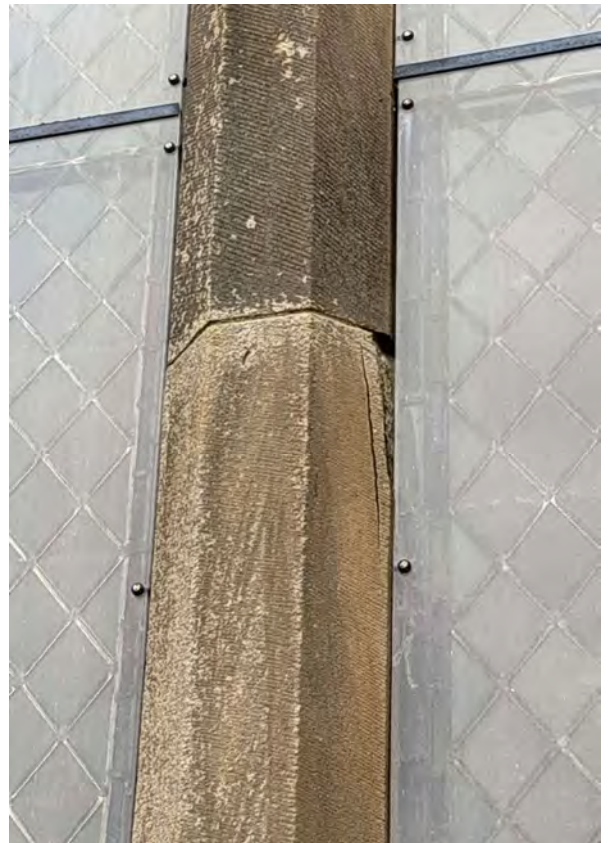
W4 – Weathering of stone to right side of mullion.
