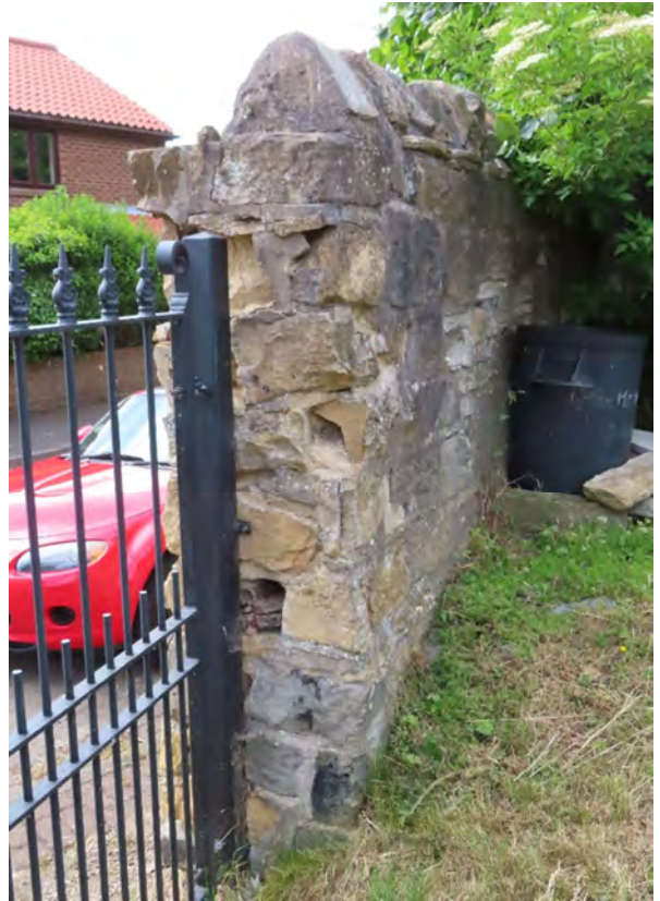
Loss of pointing & weathering to stone wall of entrance gates.
