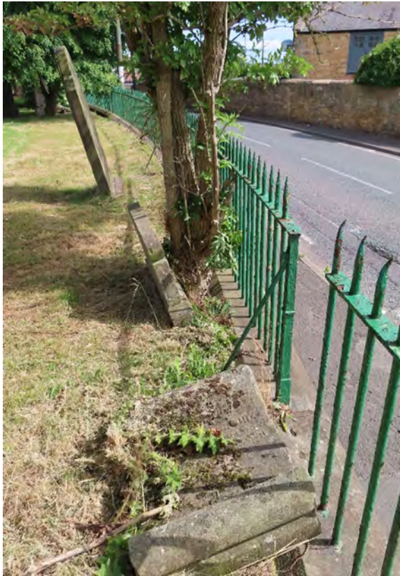
Low height of metal railings evident and sharp spikes.
