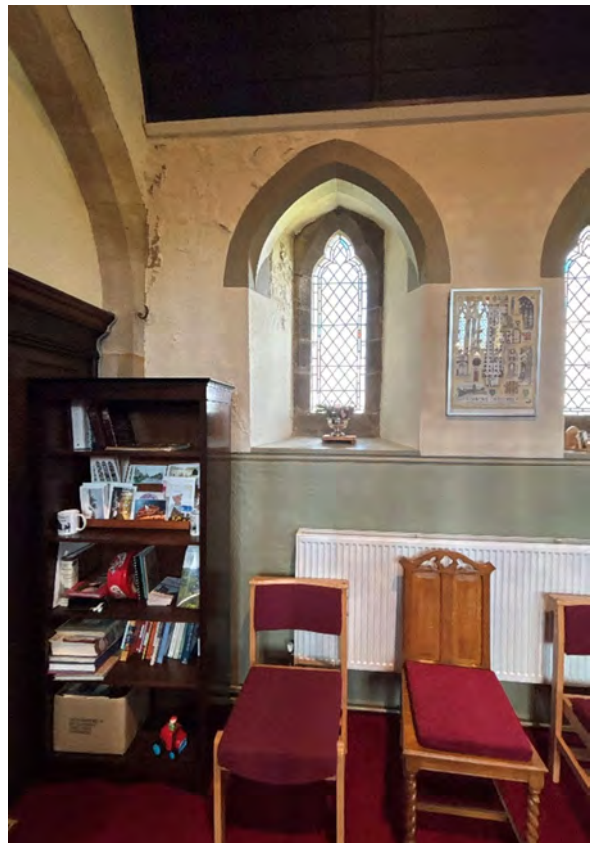
Deterioration of finishes due to issues with dampness to entrance and W10.
