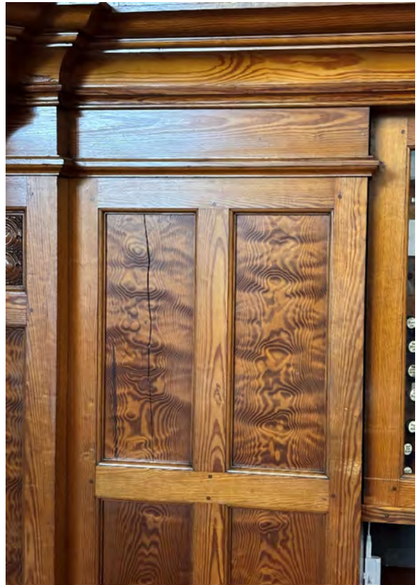
Minor crack to timber panel of Organ
