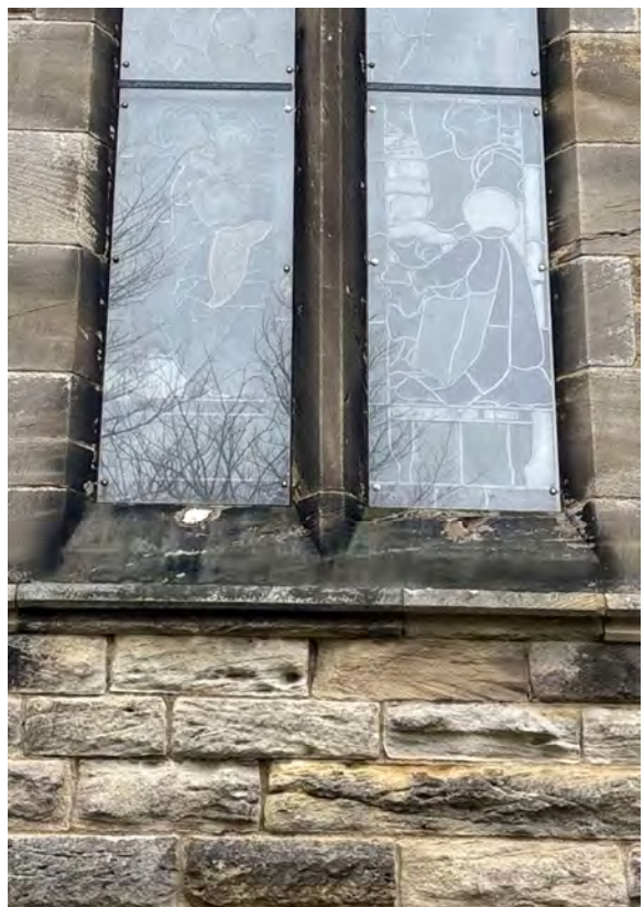
W13 – Deterioration to cill around metal fixing
