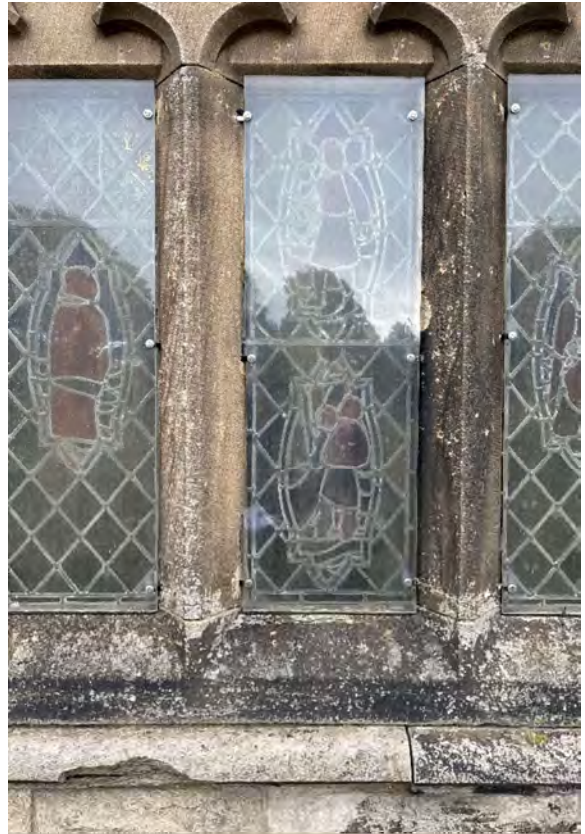
W16 – Some deterioration and cracking to stone surround.
