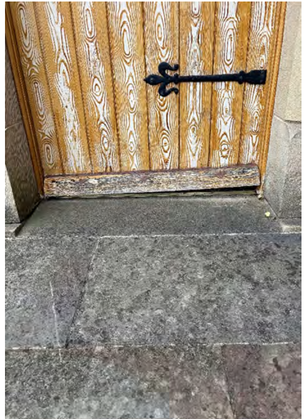
Evidence of detachment of bottom rail and loss of protective finish.
