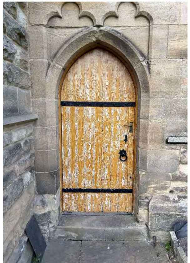
Flaking of paint/finish to Vestry entrance door.
