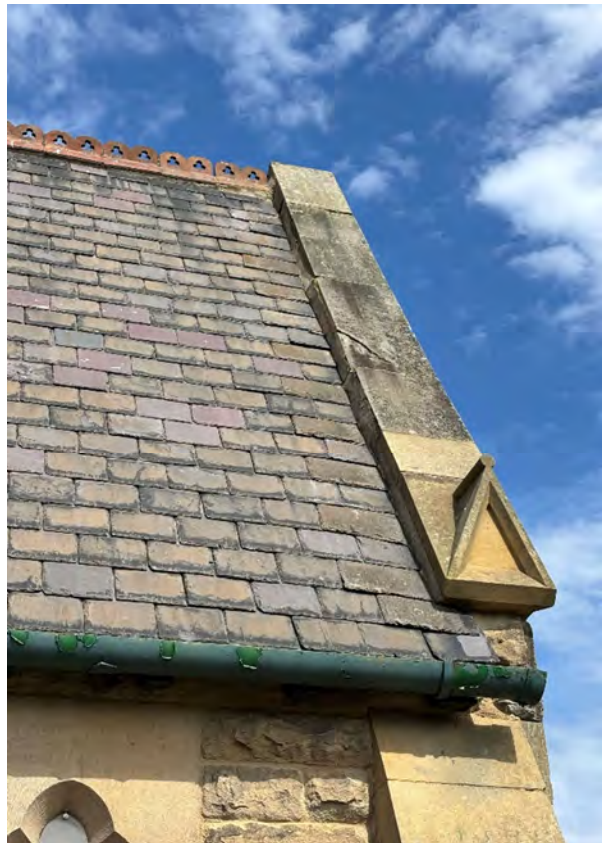
Some delamination / loss of pointing to stone.
