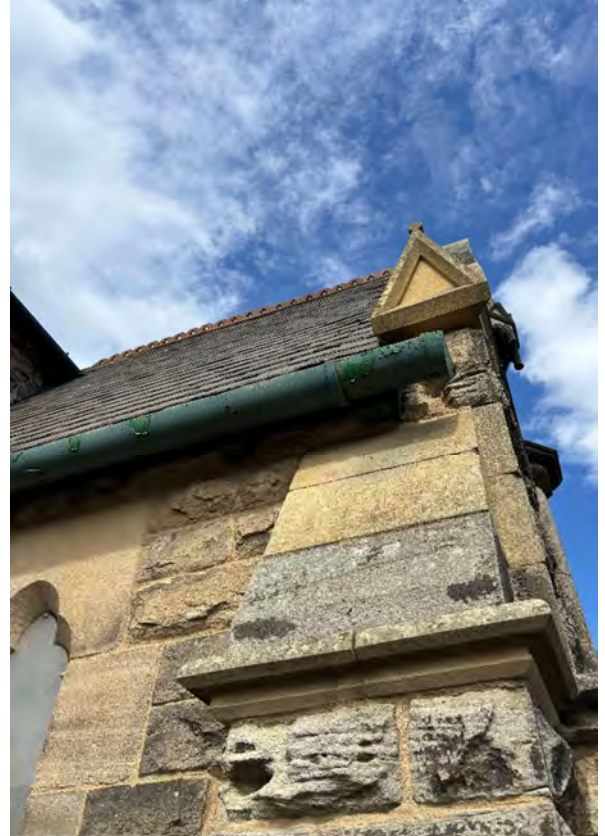
Evidence of paint failure to gutters.
