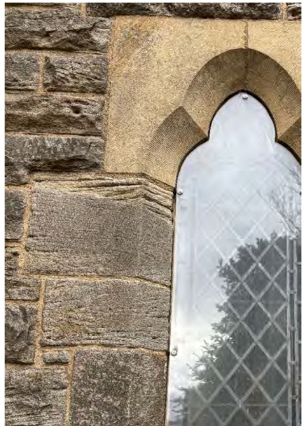
W12 – Some weathering of stone surround.
