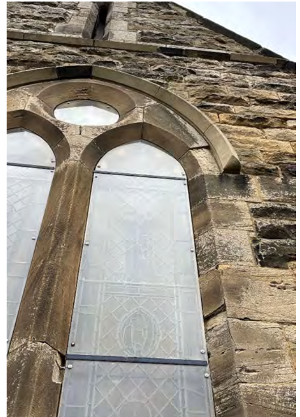
W19 – Significant deterioration of stone surround and parts of mullion.
