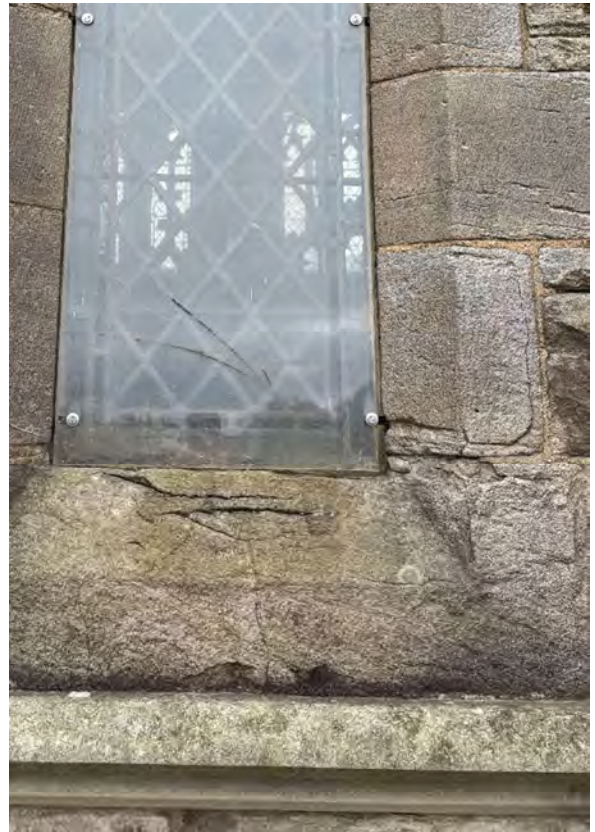
W11 – Delamination visible to cill and right side of stone tracery.
