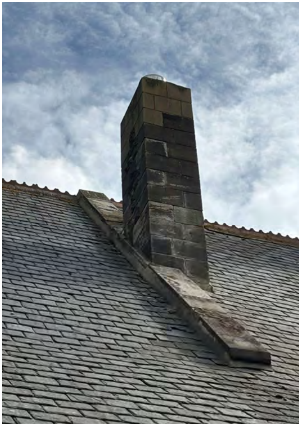
Area of Chimney which may be allowing water ingress internally. Failing mortar fillet to water table.
