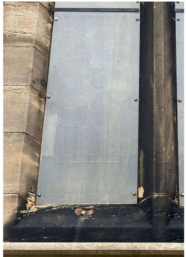
W15 – Deterioration to cill around metal fixing
