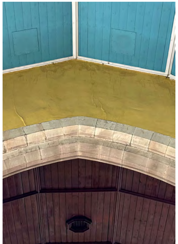
Blistering plasterwork to Chancel Return
