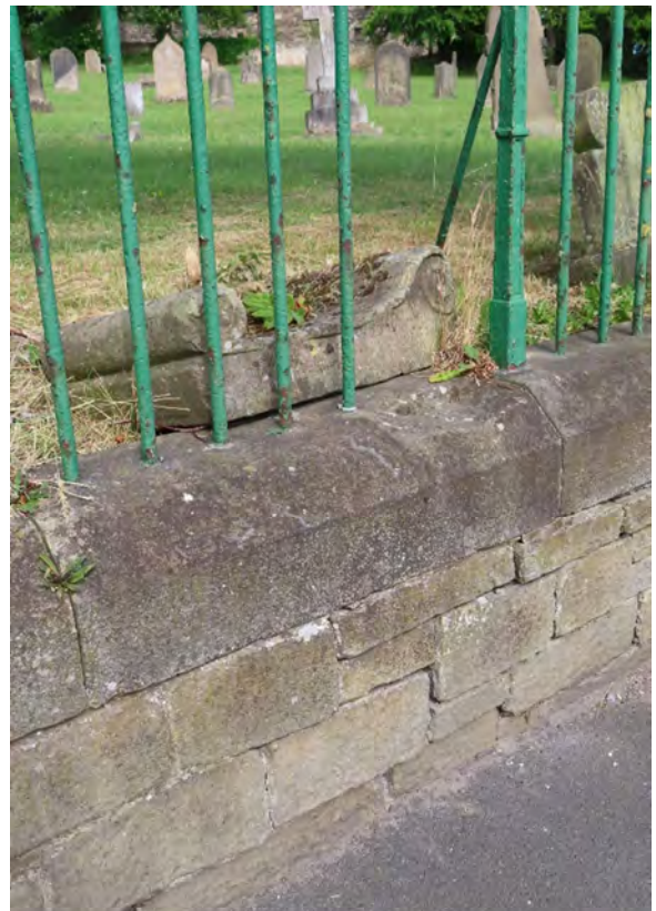
Examples of missing parts of railing and flaking of paint. Open joints to wall under. 58
