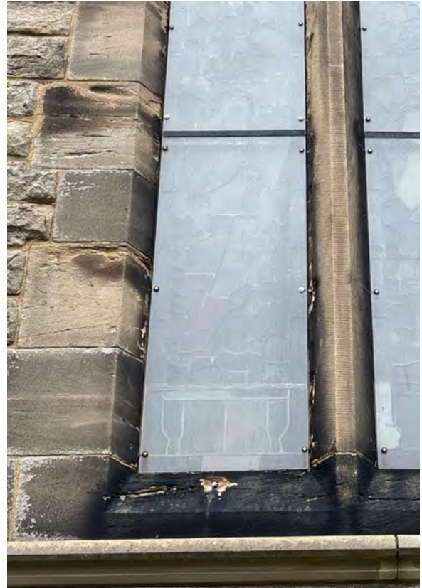
W14 – Deterioration to cill around metal fixing
