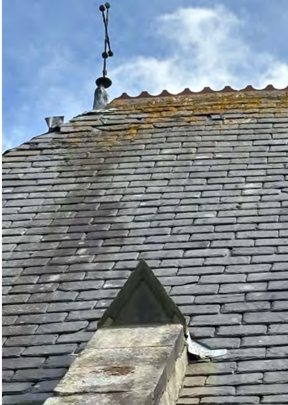
Missing, cracked slipped slates to Chancel
