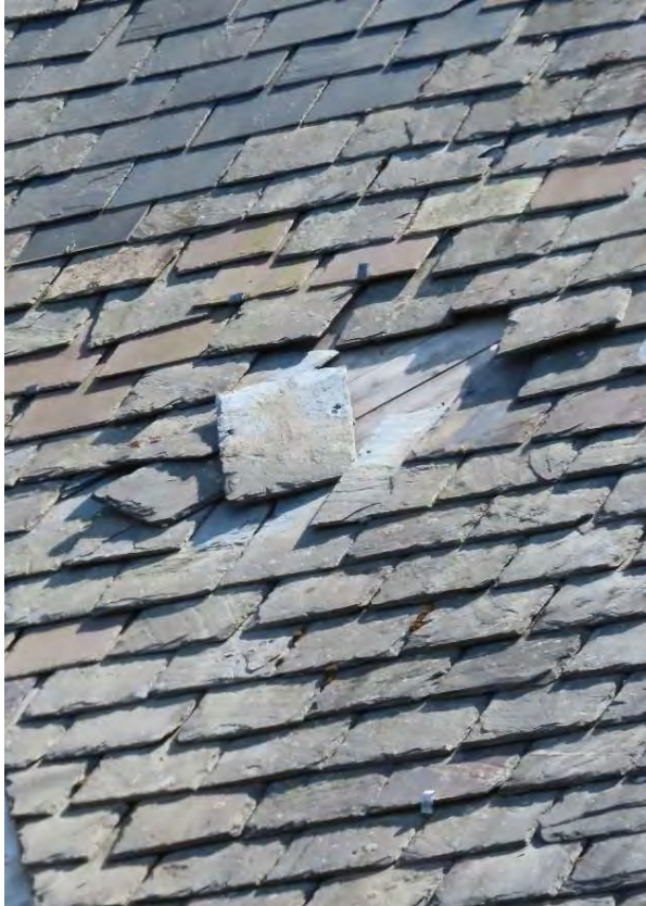
Example areas of damage to North Roof
