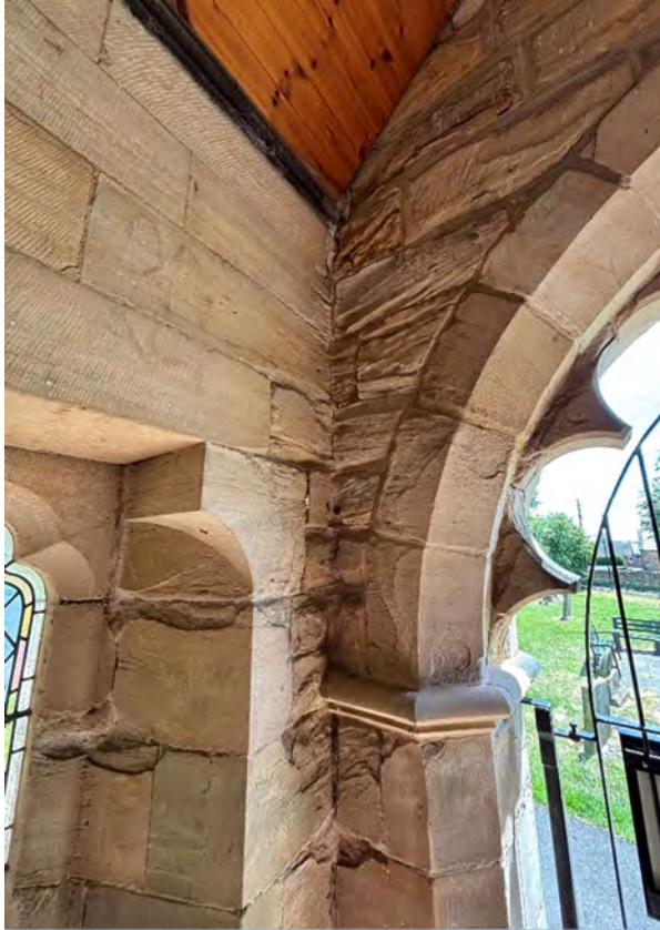
Some deterioration of stones to porch
