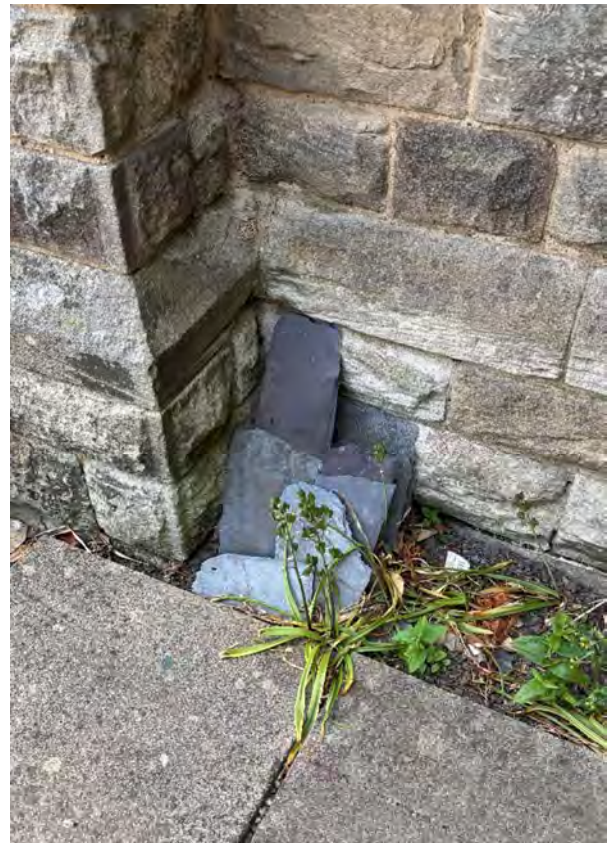
Quantity of slates missing from roof noticeable due to amount stacked next to building in various locations.
