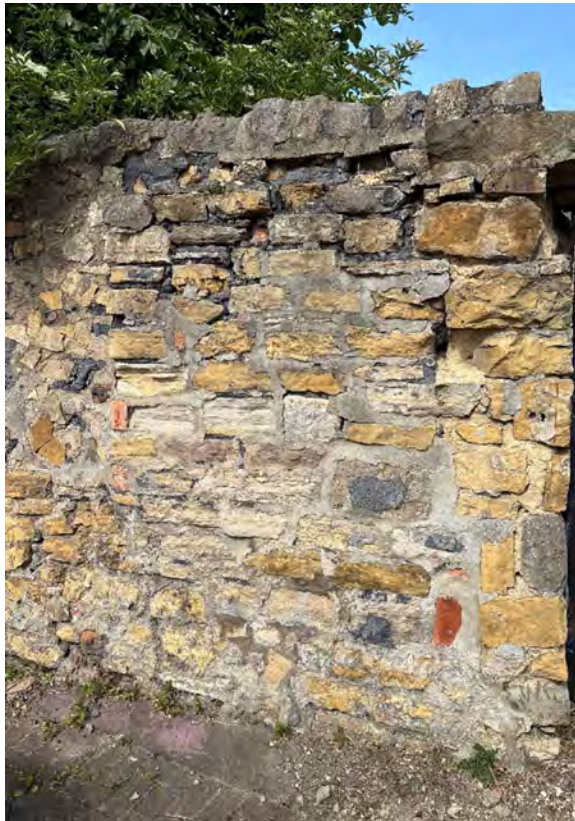
Significant areas of deterioration of stone and pointing to external entrance walls.
