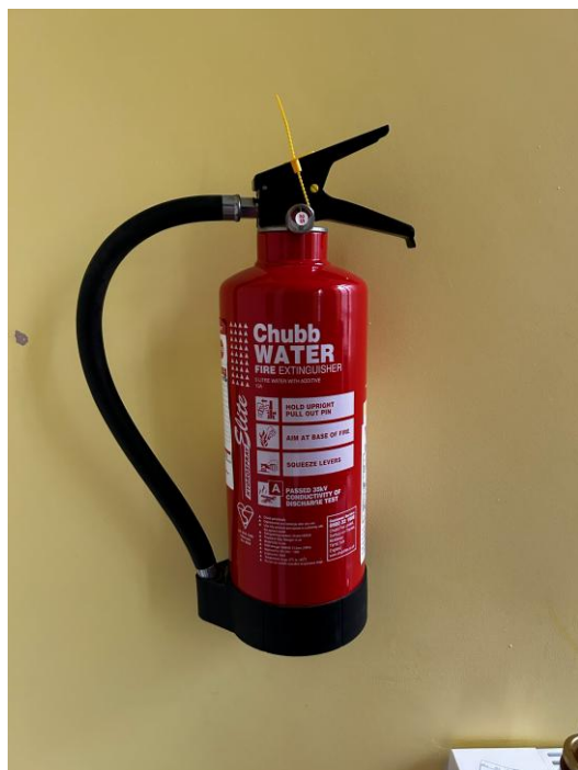
Fire extinguisher in first floor food bank
