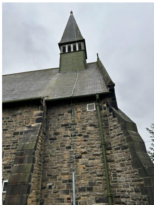
Lightning protection down steeple and northeast corner.
