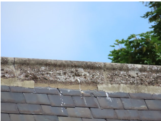
Failing mortar bedding to Southern Nave roof slope
