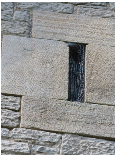
Damaged mesh to eastern slit
