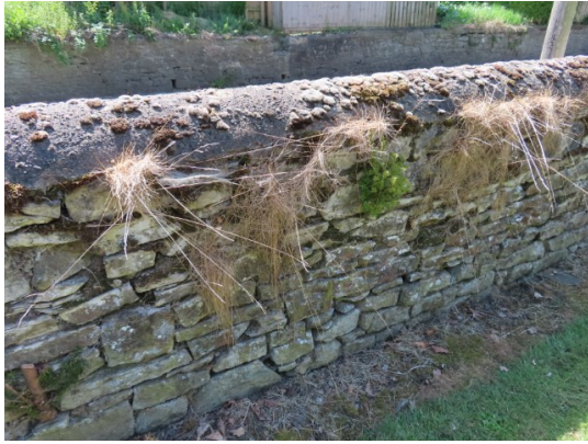
Grass growth to wall below capping on South boundary
