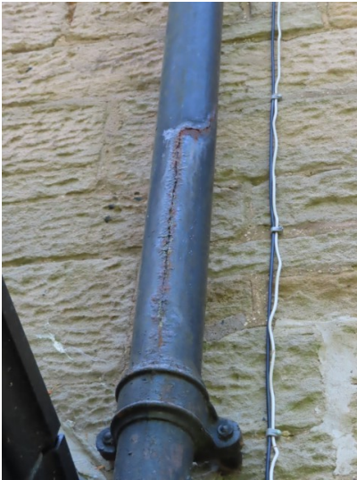
Damaged downpipe to North Elevation
