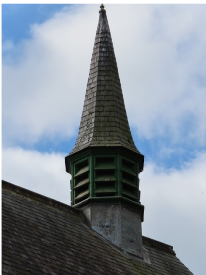
Nesting material and loss of paint finish to the fleche
