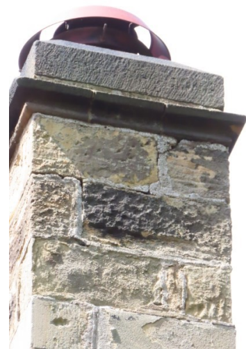
Cracking/open joints to chimney
