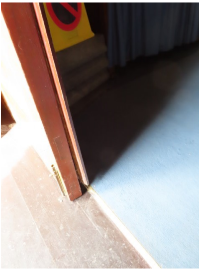
Loose cover strip to internal double doors
