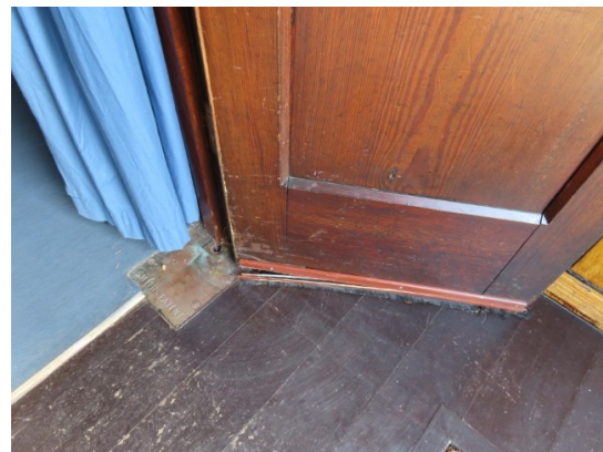
Loose draft proofing strip to the same doors
