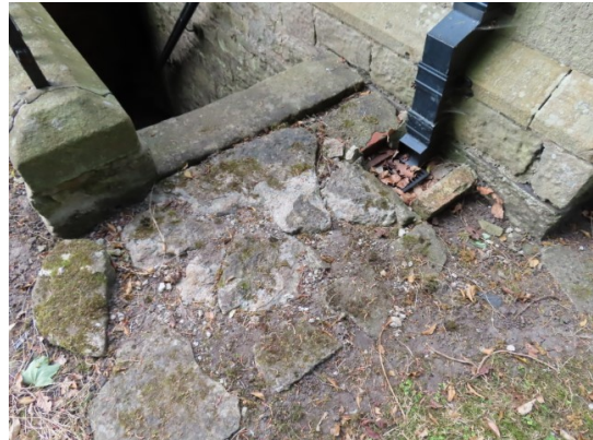
Uneven surface and leaves to Vestry gully
