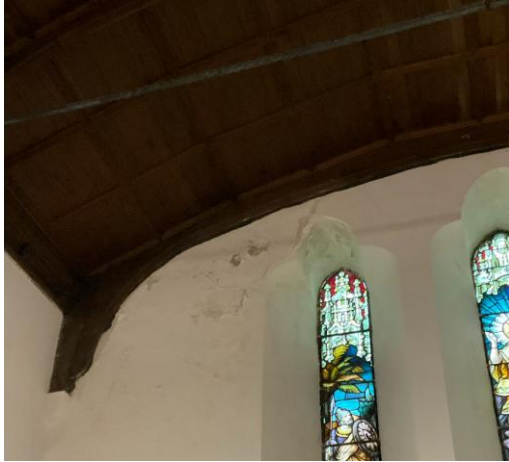
Peeling at high level on east gable
