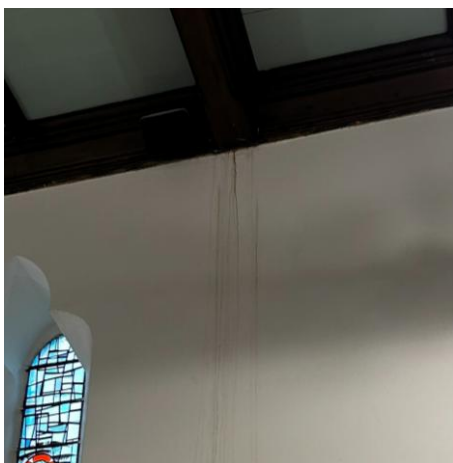
Staining at high level
