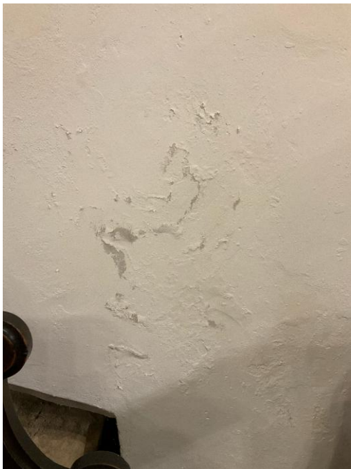
Efflorescence and peeling on north wall
