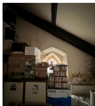
Figure 60 – damp to E wall
