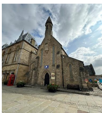
Figure 37 – cracking to W wall
