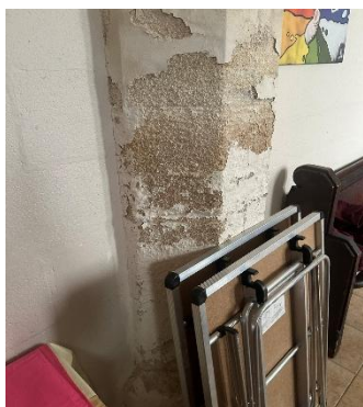
Figure 56 – Columns with damp issues
