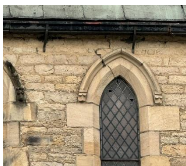
Figure 18 – Crack above lancet
