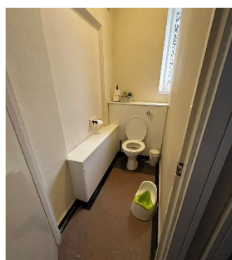
Figure 57 – WC area where floor had temp repairs
