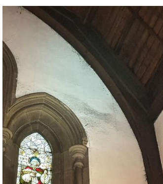
Figure 49 – staining to SE
