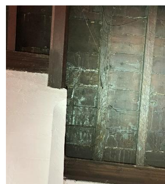
Figure 51 – Staining at mid N Aisle
