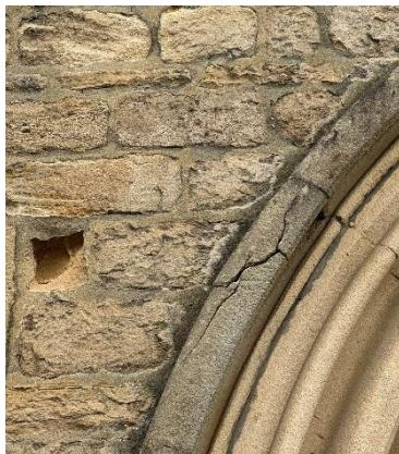
Figure 21 – Hoodmould and erosion
