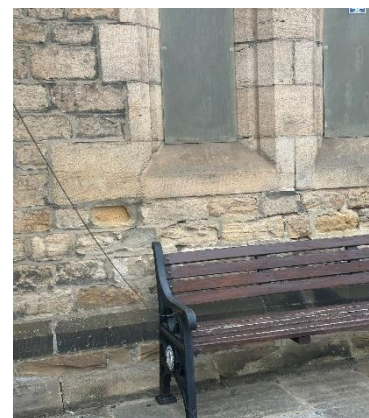
Figure 19 – second bay erosion
