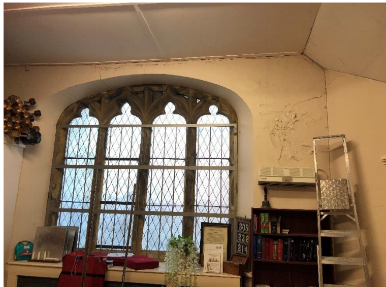
Fig 8. Localised cracking and salts liberated to north wall, Choir Vestry
