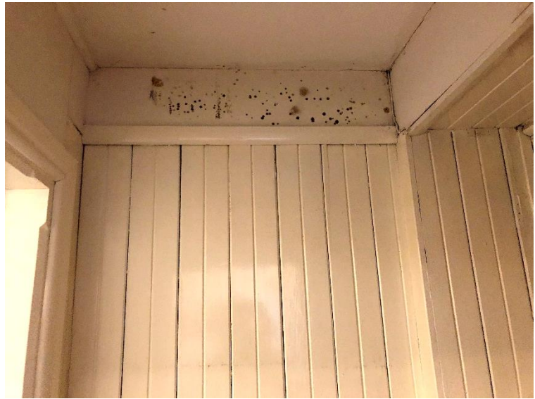
Fig 9. Mould (condensation?) in west lobby, Choir Vestry
