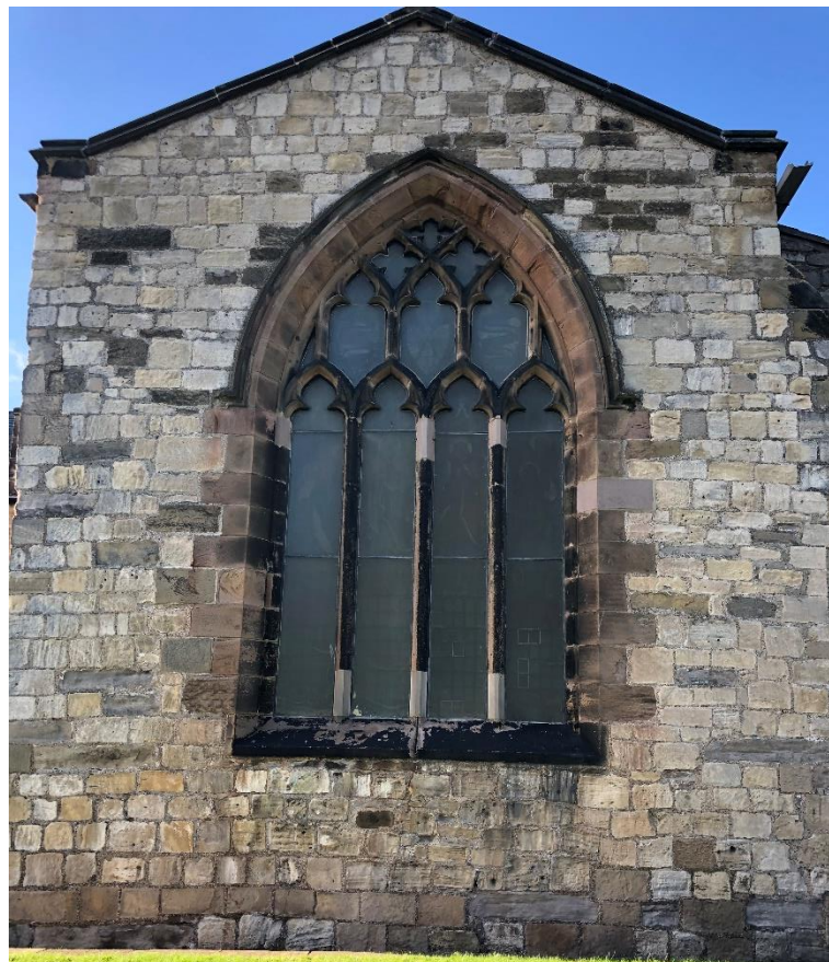
Fig 4. Vertical cracking below east chancel window: no visible change
