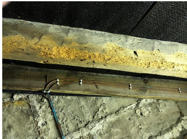
Fig 2. North aisle roof timber, previous window infestation: check treatment
