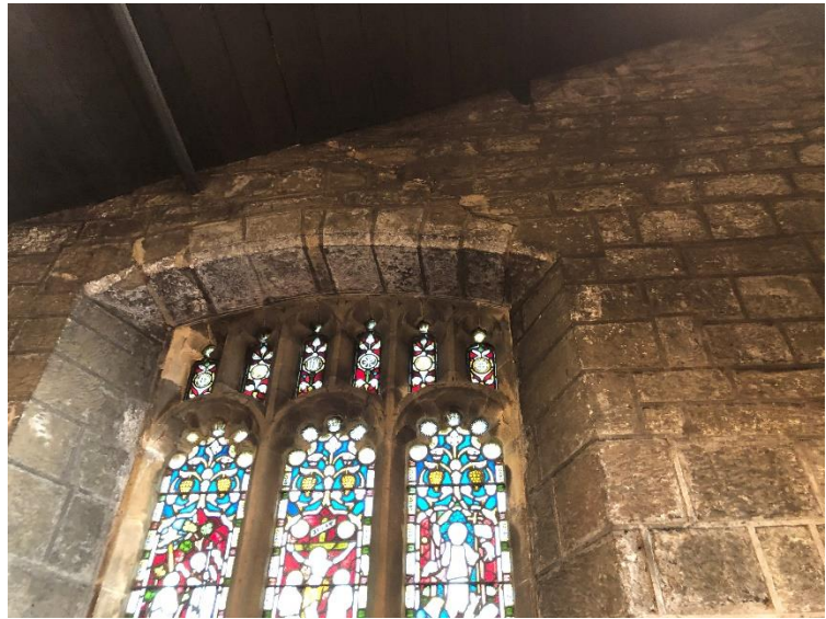
Fig 1. East gable above window cracking (Fulthorpe Chapel): no visible change
