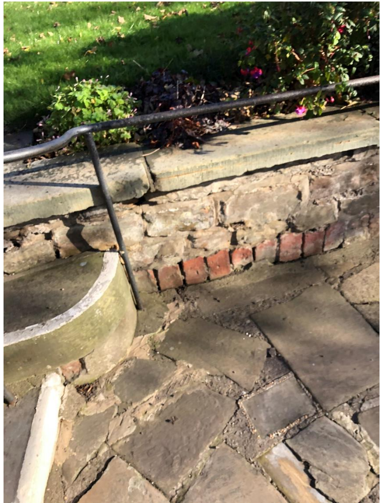
Fig 7. Open joints, entrance steps retaining wall
