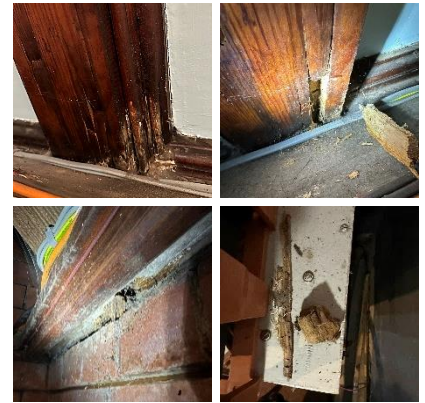
Figure 18 – South Aisle timber decay
