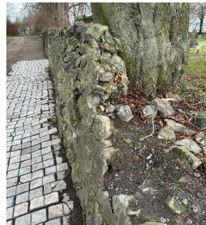
Figure 31 – Collapsed wall to W
