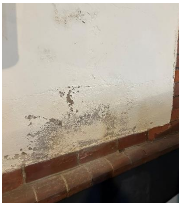
Figure 23- Damp to S Aisle
