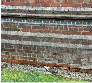
Figure 9 – Eroded brick to LL East
