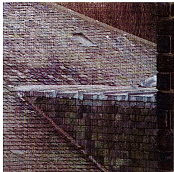
plants in cracked mortar fillet N of the tunnel between Tower and Nave roof
