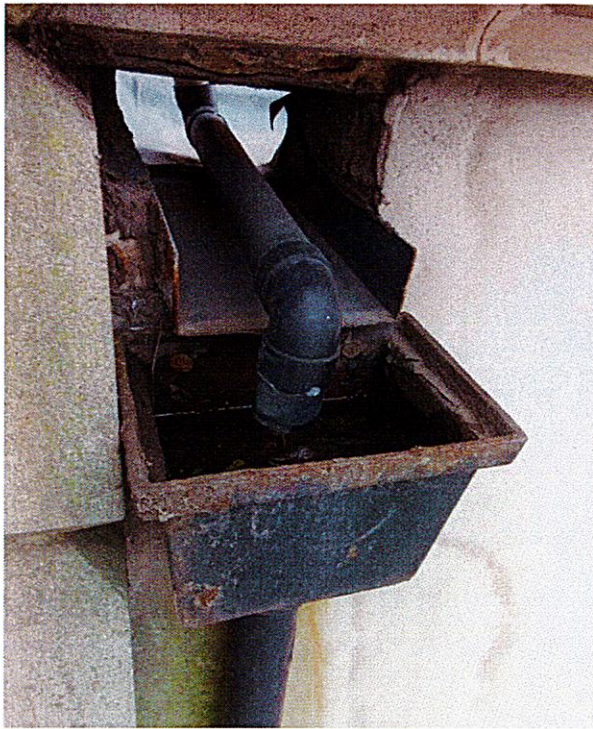
Kitchen hopper blocked and unpainted
