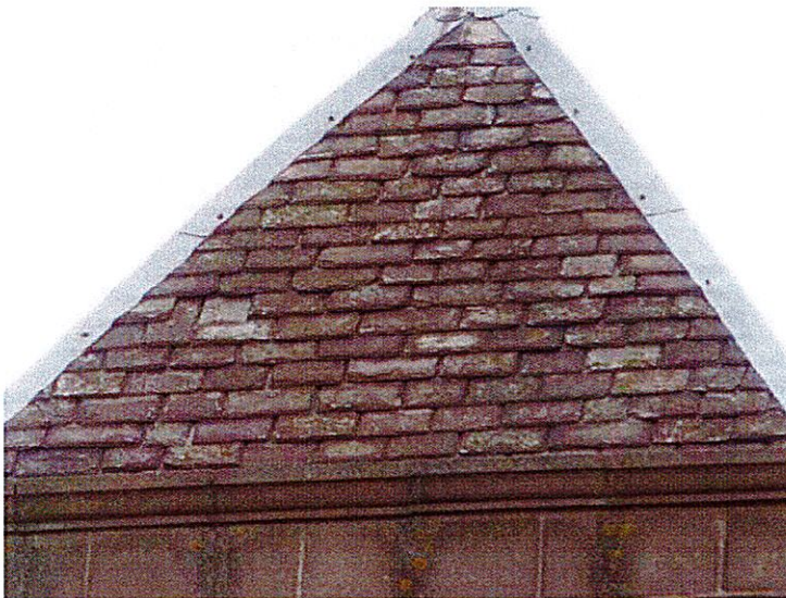
Slate missing from Tower N side
