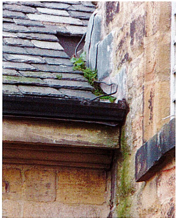
plants blocking secret gutter N of the Tower (paras 20,30) wall below wet
