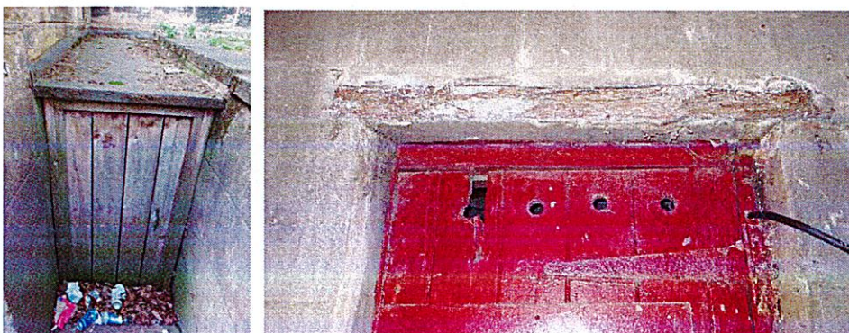
Decaying Lintel at Blower door
