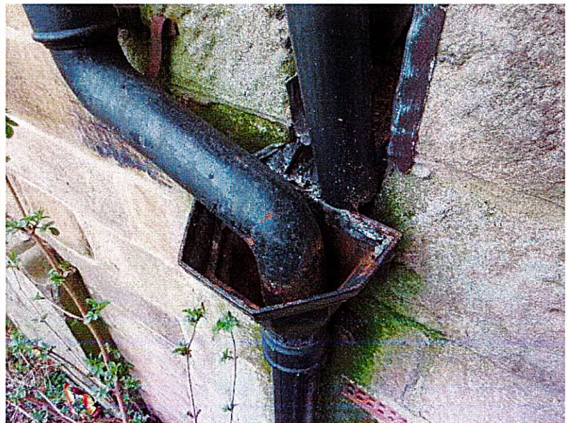
Misaligned pipe misses the hopper E of the Song Room
