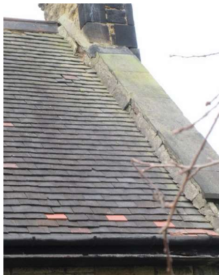
typical broken mortar fillets
