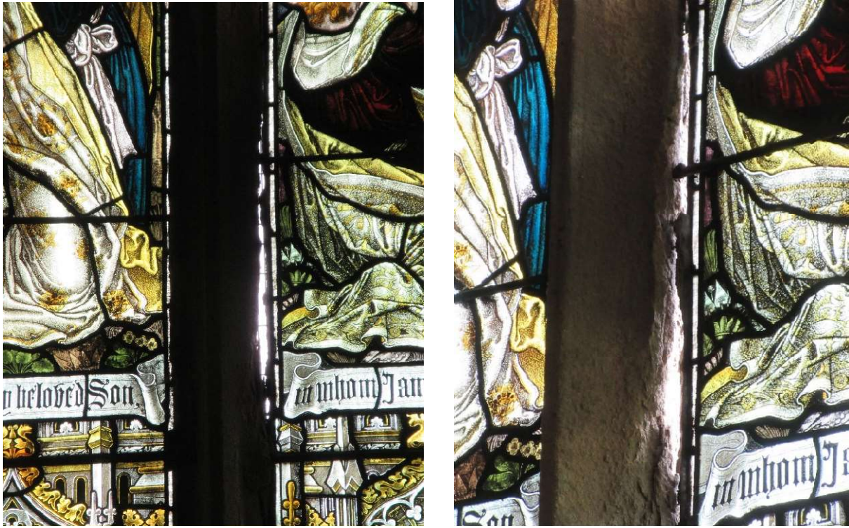
Daylight through the gap between the decayed mullion and the centre light glass
