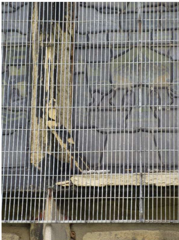
Base of S central mullion
