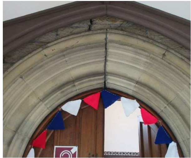
Open joints over Porch outer arch
