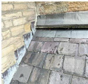
Item29- Flashing to South Porch
