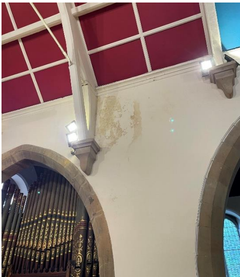
Item 97- Damp & Flaking Paint
