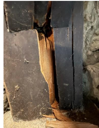
Item 84- Timber Softening
