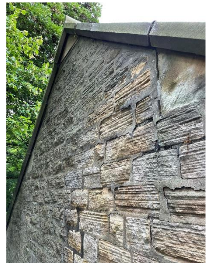
Item 50- Open Joint
