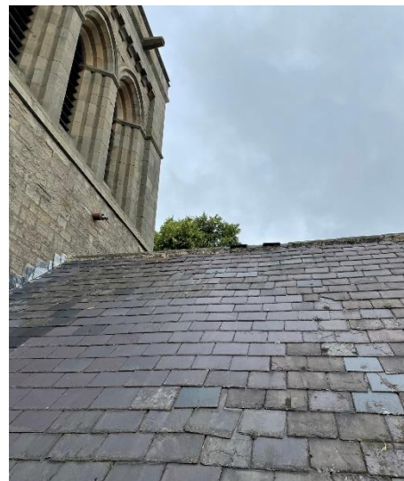
Item 18 & 31- Area of patched fibre slate & Ridge Vents
