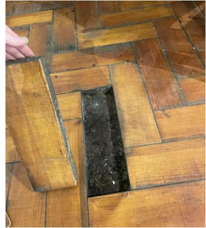
Item 110- Block Floor Loose Piece
