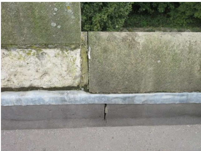
Split asphalt upstand and opening joint between parapet stones at middle of W side
