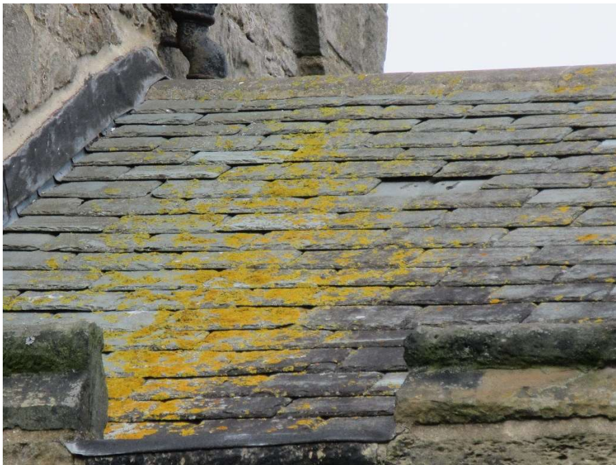
Slipped slate at SW Nave
