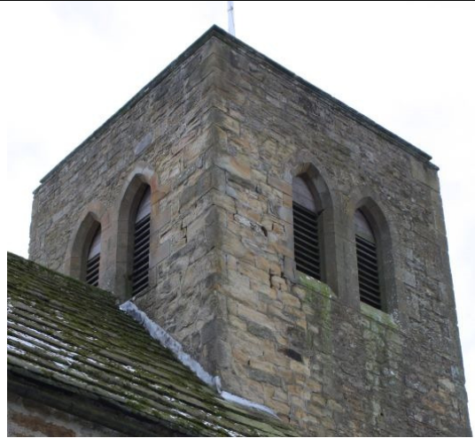
Tower – large open joints (6.6)
