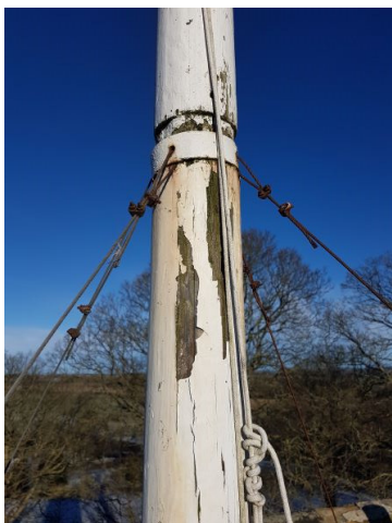
Flaking paint to flagpole (6.3)
