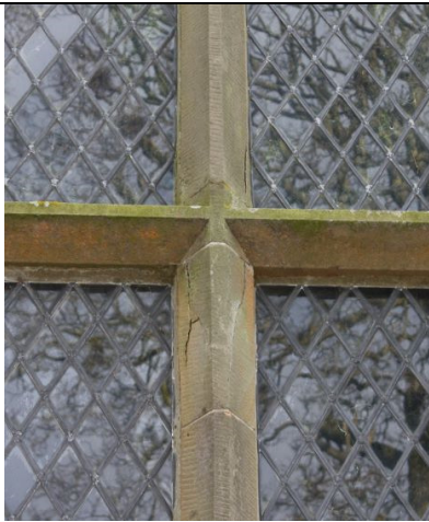
Nave north window n(v) – cracks to mullions (6.7)
