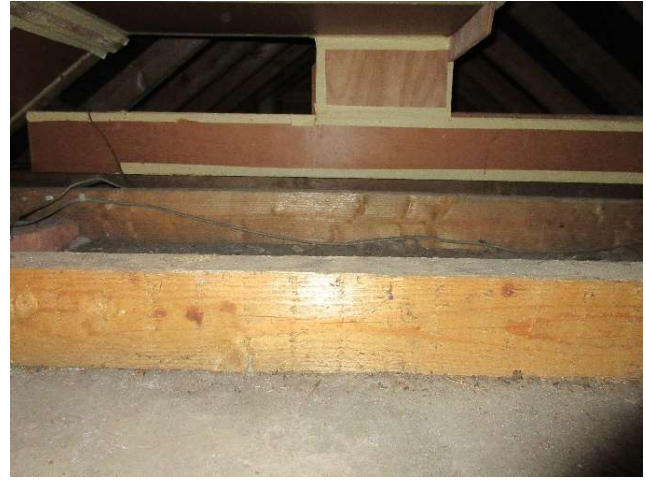
no ceiling insulation
