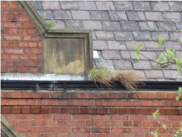
Gutter choked by plants before clearance at the inspection
