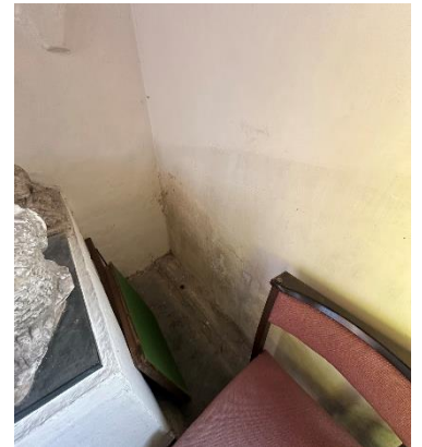
Figure 20- Damp to S Chapel
