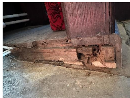
Figure 24 – rotten raised pew platform N Choir
