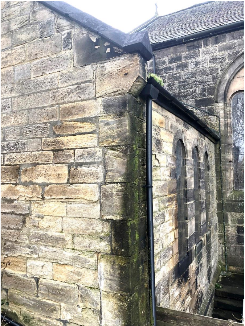
P4 (0555): Vestry gutters blocked
