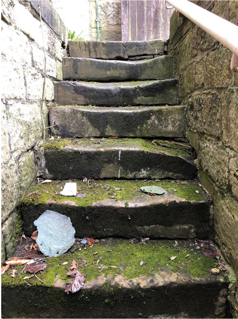
P12 (0653): Boiler room steps to be cleared
