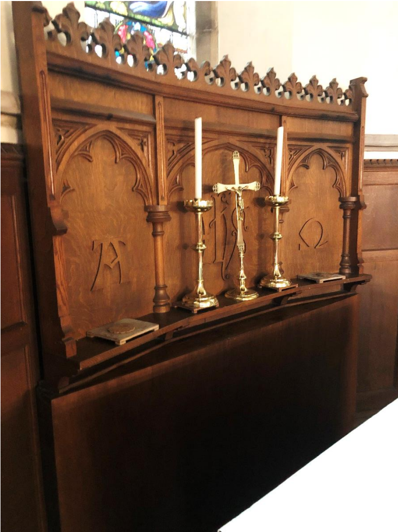
P9 (0618): Missing cresting to reredos
