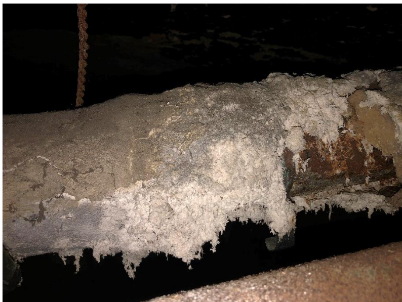
P2 (0651): Deteriorated pipework insulation (asbestos containing material?)
