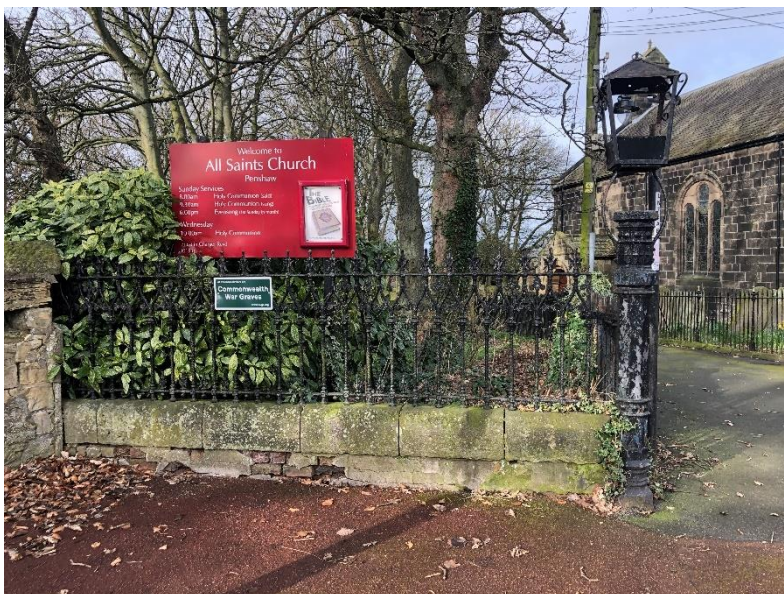
P7 (0584): Boundary entrance wall, lost render (ironwork maintenance responsibility, Sunderland City Council)
