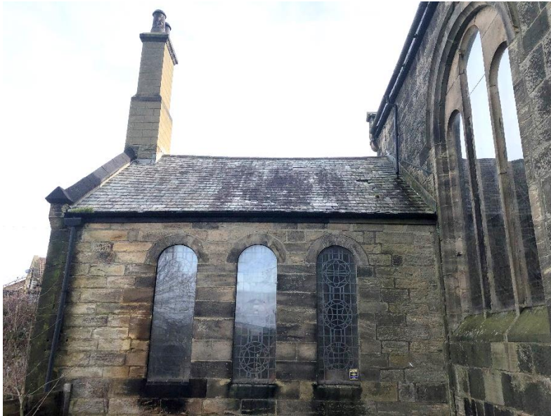
P5 (0561): Vestry roof, missing slates
