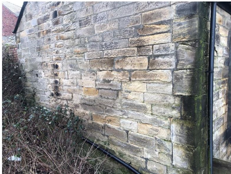
P6 (0554): Pointing issues, north Vestry wall and elsewhere
