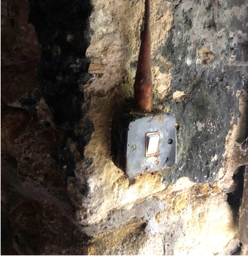
P3 (0649): Deteriorated lighting installation, Boiler Room
