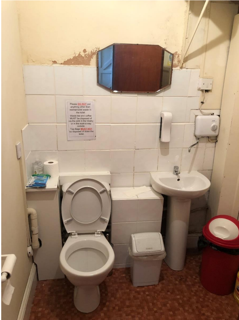
P10 (0636): WC improvements necessary (Doc M pack)
