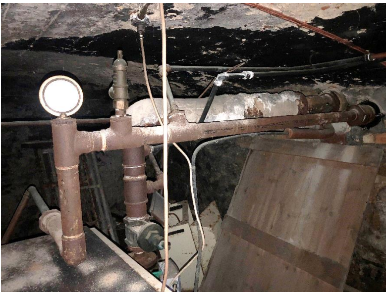
P11 (0646): Boiler room to be tidied
