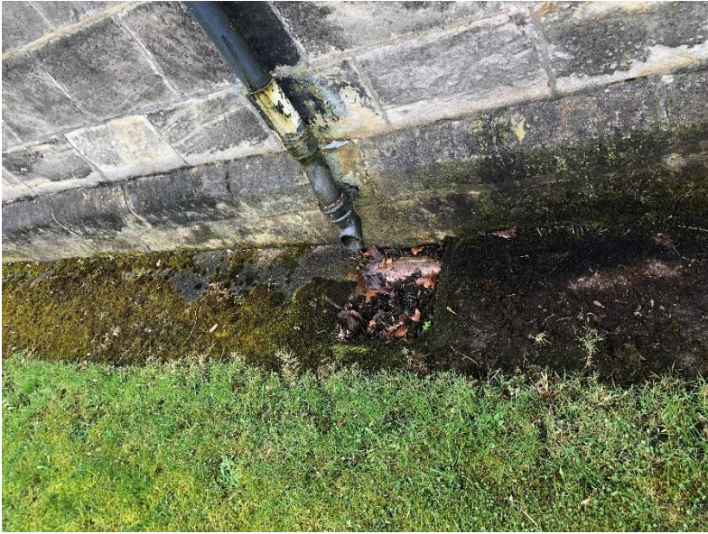
P8 (0570): Gulley/stone channel to be cleaned; downpipe/gutter maintenance needed
