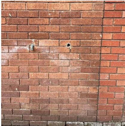
Fig 1 – Holes to west elevation
