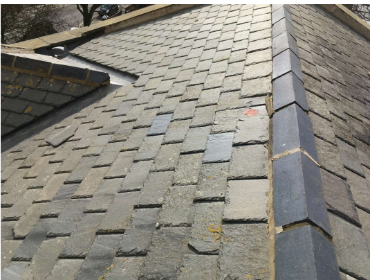
Photo 4 Broken upper slate on South Transept.
