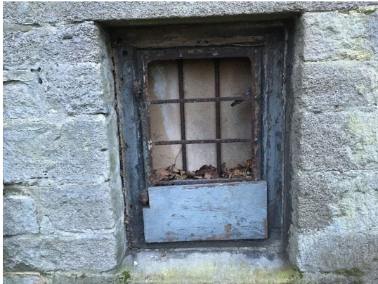
Photo 26 Dilapidated (blocked) window (W8) to rear of safe cupboard.
