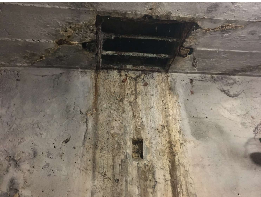
Photo 22 Water staining below ventilator north side of undercroft.
