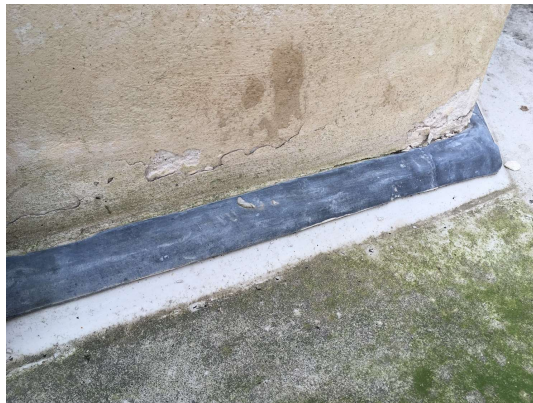
Photo 13 Frost damage to lime render above lead tray on stair abutment.
