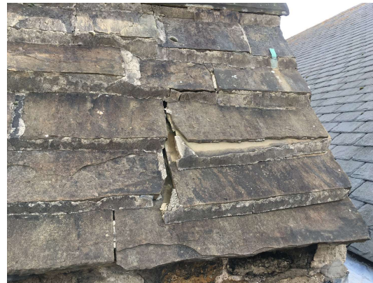
Photo 12 North buttress slipped slates.
