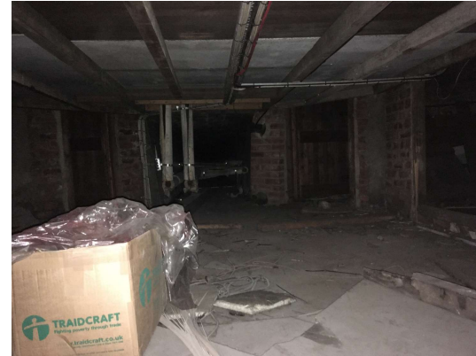
Photo 23 Asbestos cement panels on soffit and possible asbestos insulation to pipework of undercroft.
