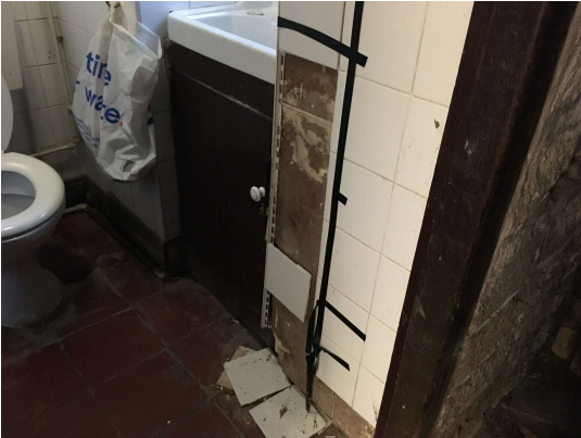
Photo 20 Loose tiles in Vestry WC.
