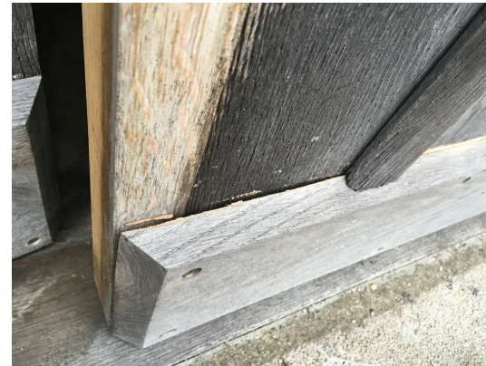
Photo 18 Shrinkage on rear of repaired weathermould southeast Porch.
