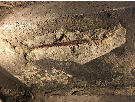
Photo 16 Eroding stair soffit with corroding reinforcement.
