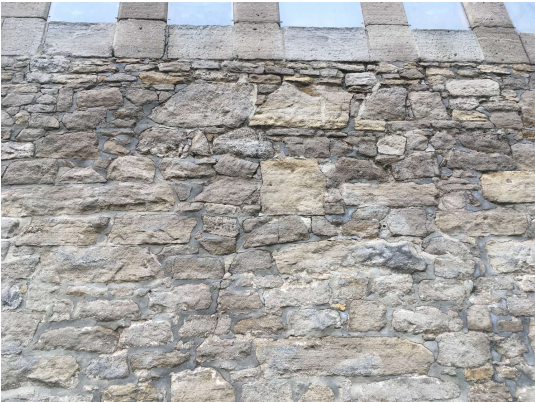
Photo 15 Cement patch pointing on South Transept.
