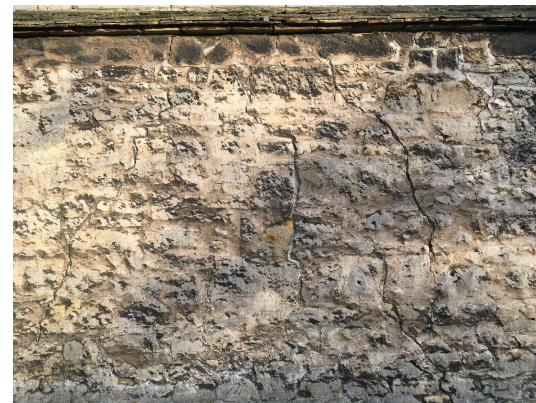
Photo 19 Cracking below west window.
