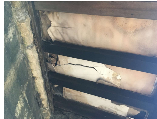
Photo 24 Loose mortar above southwest Porch.
