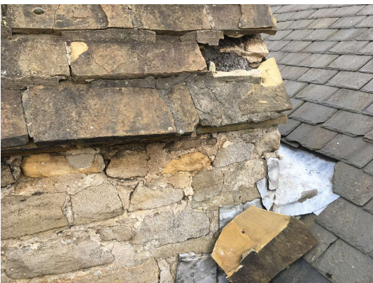
Photo 10 Slipped slate north buttress.
