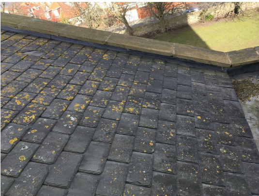
Photo 3 Broken slate on North Transept.
