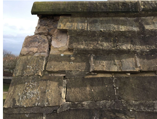
Photo 11 North buttress slipped and missing slates.
