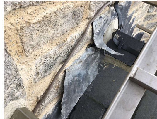
Photo 5 Loose flashings at Tower abutment.
