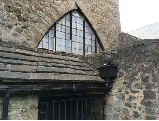
Photo 14 North Porch window with bowed and broken panes, and corroded steel frames which are damaging masonry.
