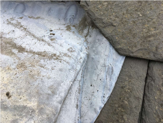
Photo 8 Worn lead on buttress back gutters.
