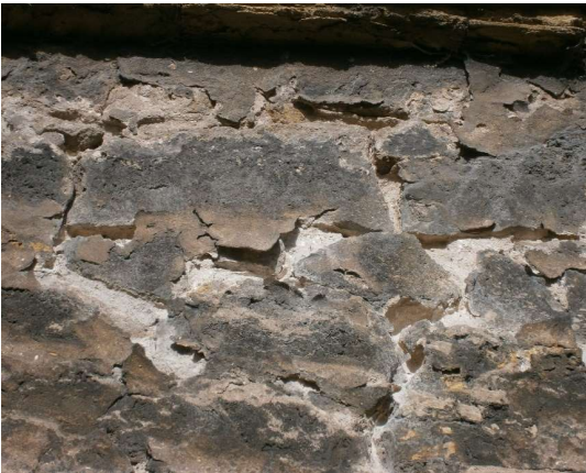
Photo 9 Eroded lime mortar behind cement pointing below cills on Nave.
