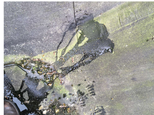
Photo 7 Holed nave gutters contain water between layers.
