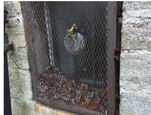
Photo 25 Corroded grille to vestry WC window.
