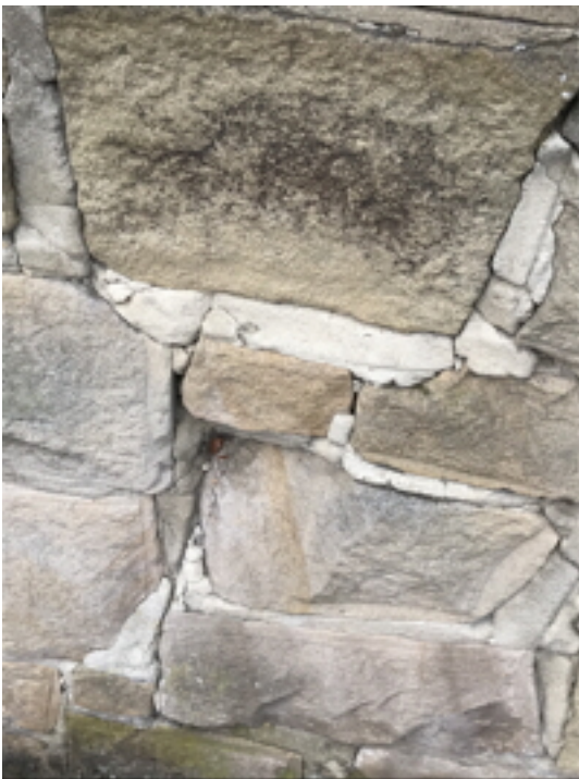
Loose Pointing to East Wall Stonework
