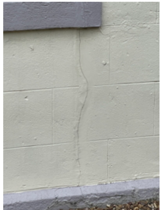
Cracking below Meeting Room windows west elevation
