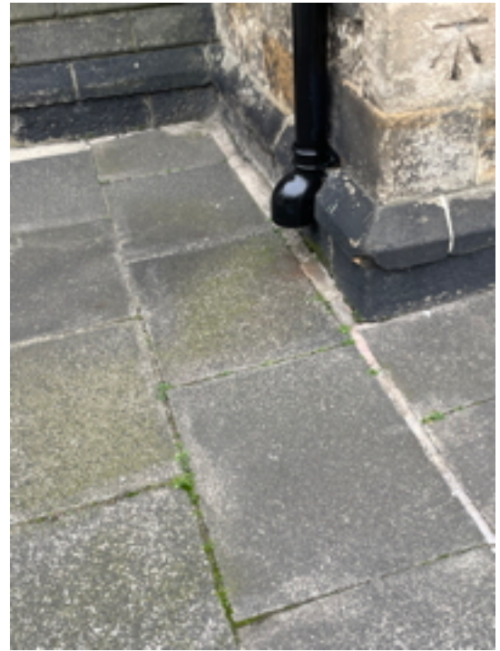
Entrance Porch West Wall pipe discharging over paving
