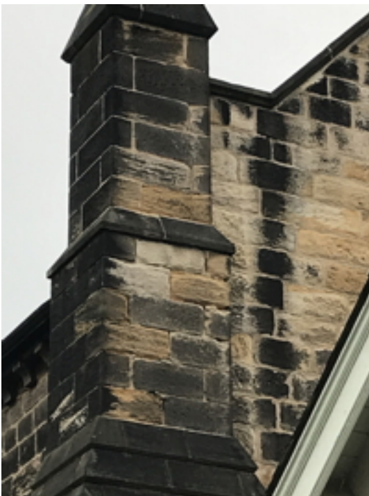
Open Mortar joints to Nave West Wall, North West Corner
