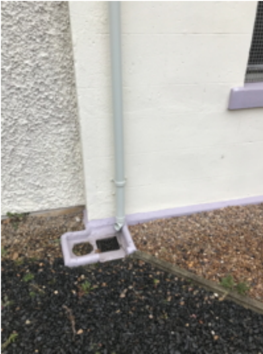
Hall West Wall UPVC Rainwater Pipe
