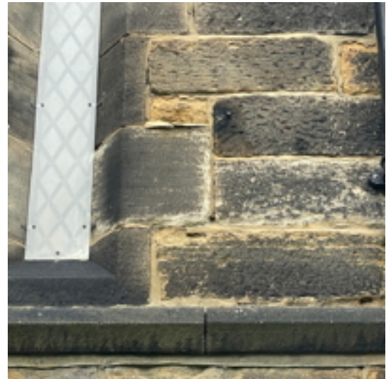
Loose mortar pointing Chancel south elevation east end
