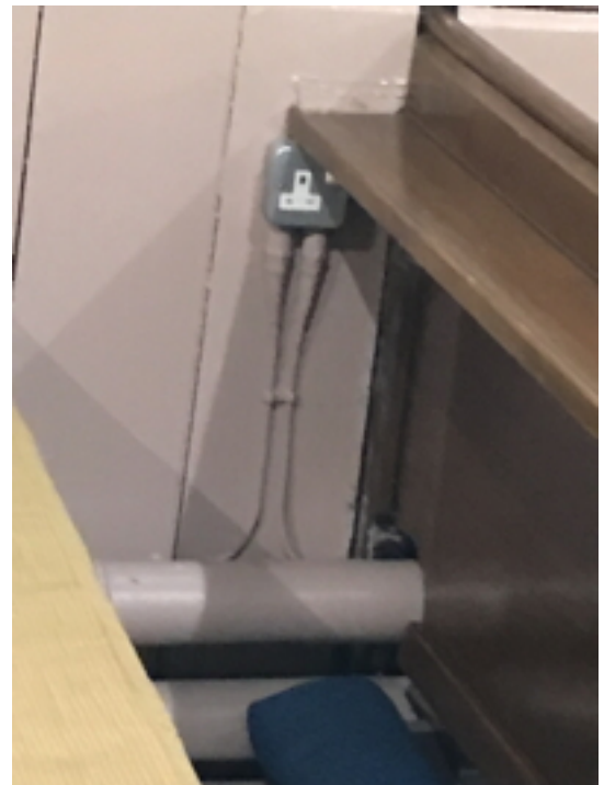
Perimeter Heating Pipework
