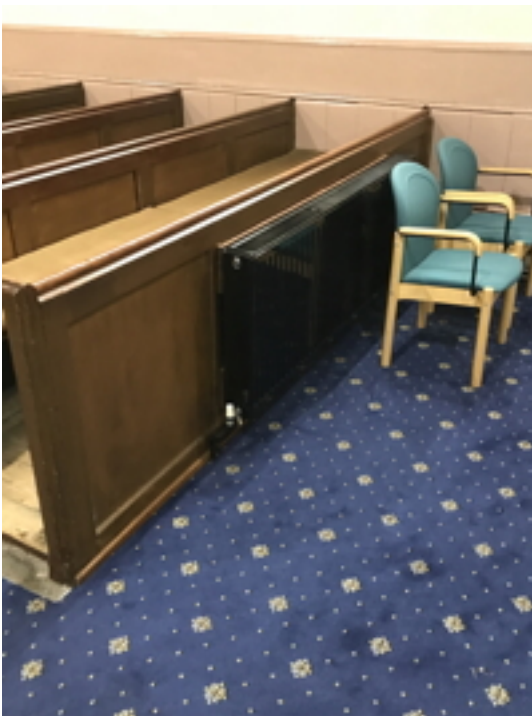
Front Pew Radiator
