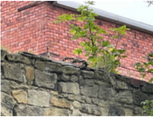
Sycamore seedling to west boundary wall coping
