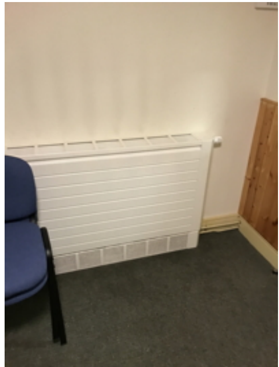
Typical Hall Radiator
