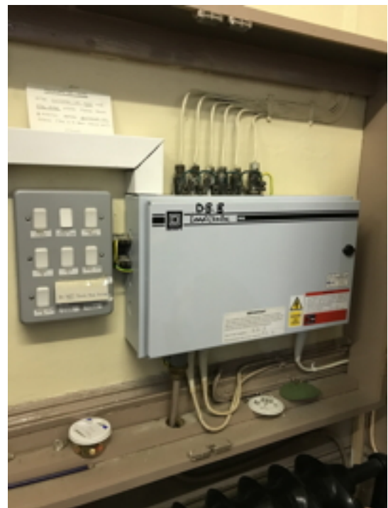
West End Distribution Board
