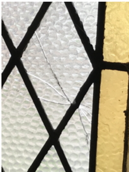
Cracked glass panes visible from organ loft
