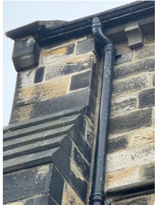
Church Gutters and Rainwater Pipes in need of redecoration
