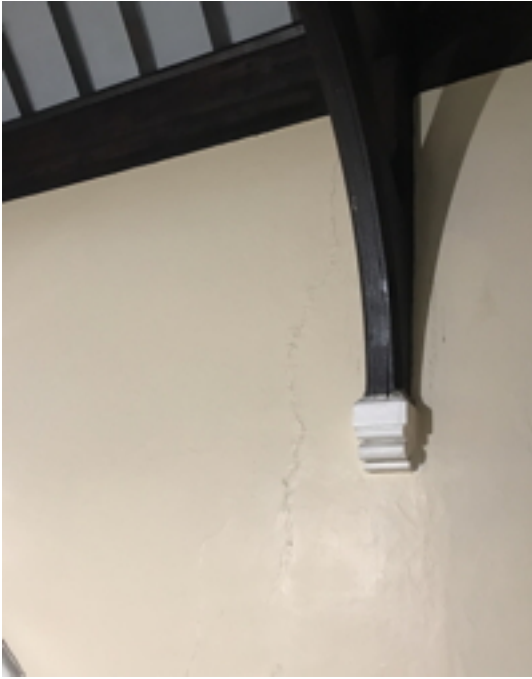
Crack to South Wall
