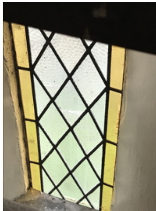
Cracked glass panes visible from organ loft
