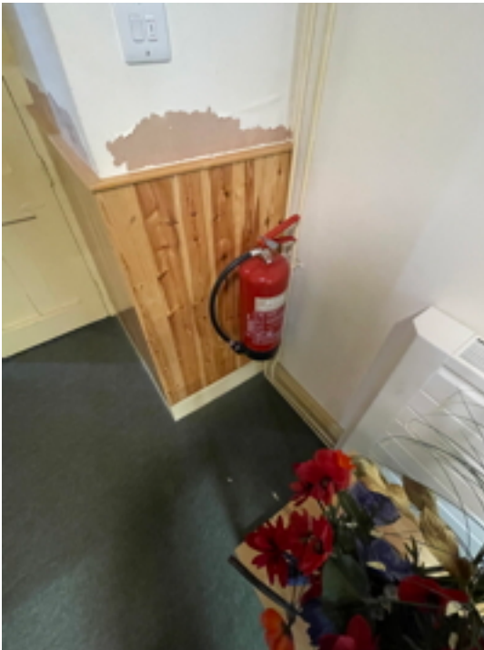
Peeling paint to Meeting Room
