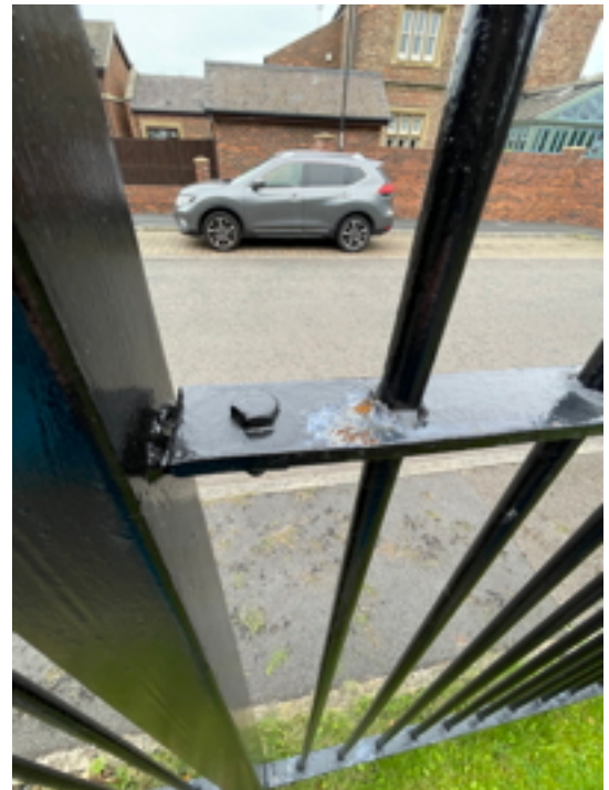
Rust to North Boundary Railings
