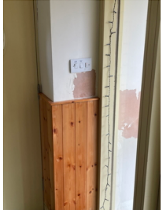
Peeling paint at Meeting Room entrance doors
