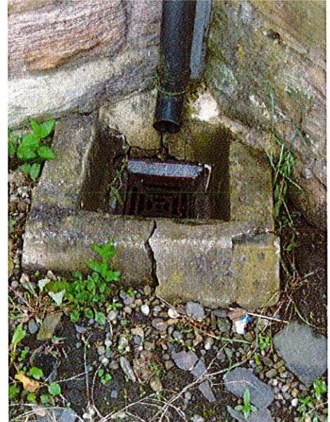
Cracked gully surround at SE nave-para 24
