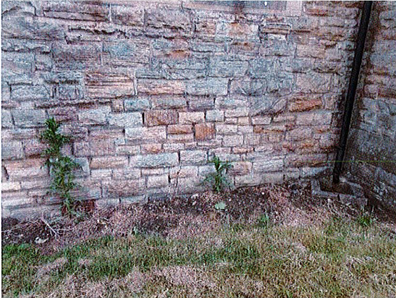
SE Nave – ground level too high – air brick part blocked by soil and plant
