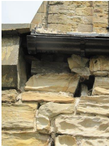
Exposed wall plate and open joints to South elevation of South Aisle
