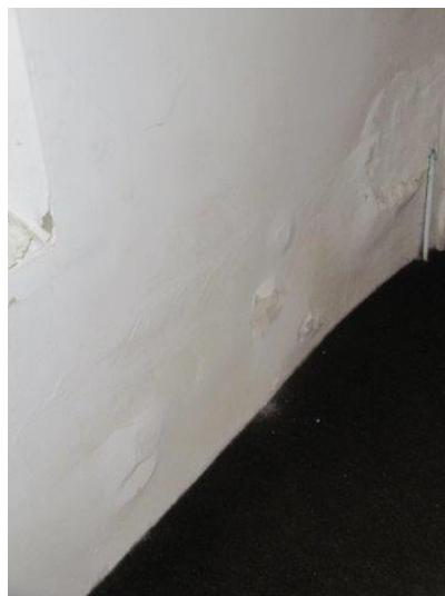
Damaged plaster in Vestry
