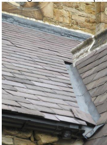
Lifted flashings to Nave roof (South)
