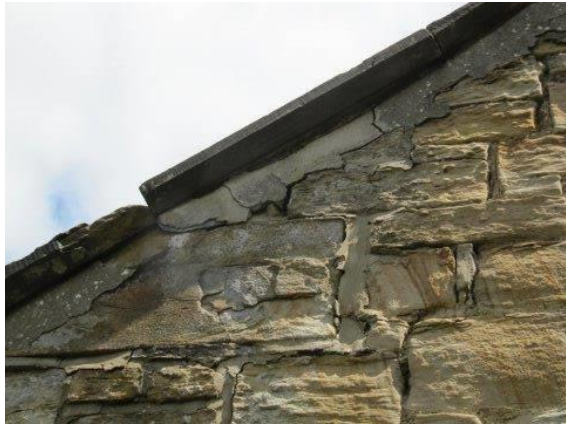
Cracked pointing and open joints to West Elevation of North Aisle
