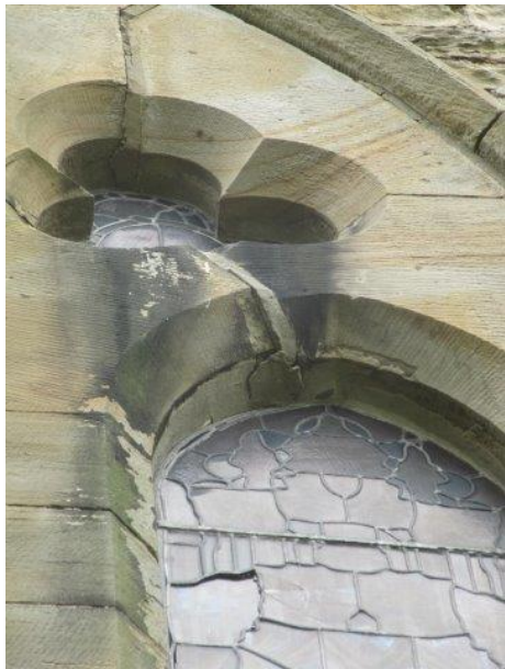
Cracking and loose mortar to east Chancel window
