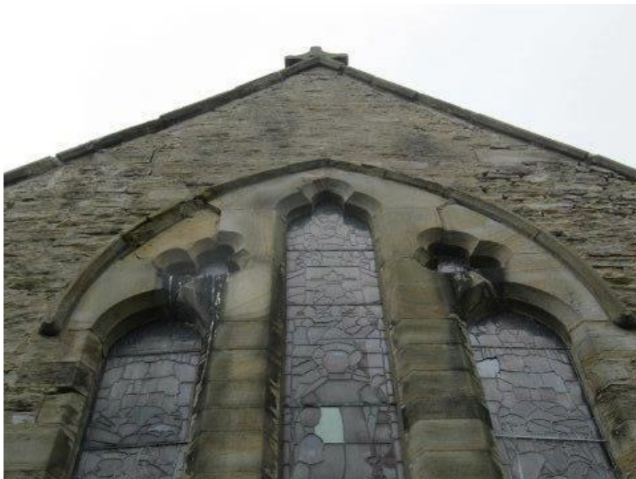
Damaged and rusty window guarding and resultant rust stained wall to Chancel
