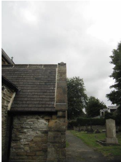
Salts visible to West Elevation of South porch
