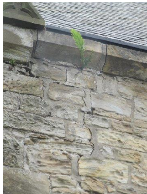
Crack and sapling to North Elevation of Chancel
