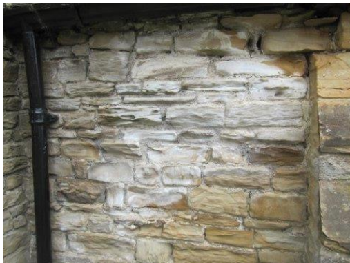
Salts visible to West Elevation of South porch
