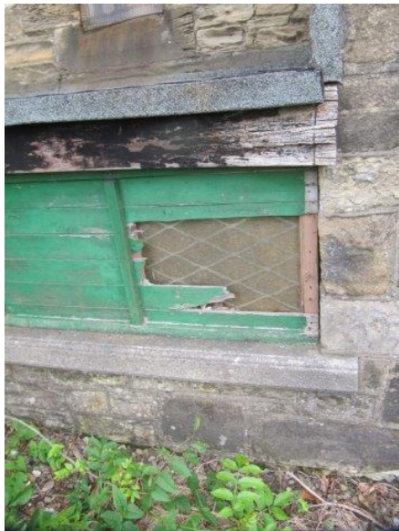
Damaged timber cladding to stairs
