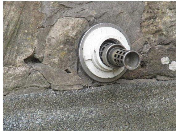
Cracked mortar around heater flue to East of vestry
