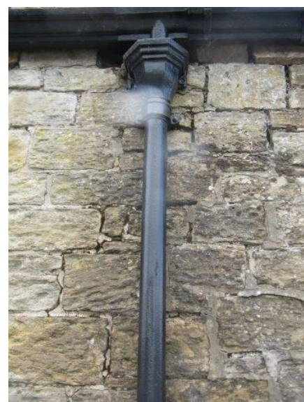
Cracking/open joints to West end of North Elevation of Aisle
