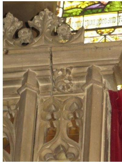
Cracking to carved stonework behind altar
