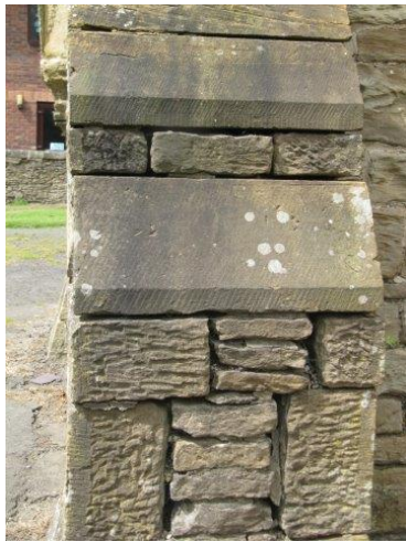
Hungry/open joints to East buttress of porch
