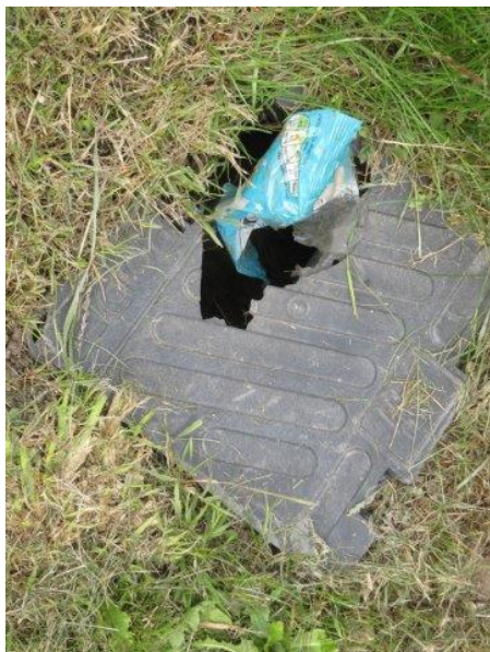
Cracked cover to West of the church
