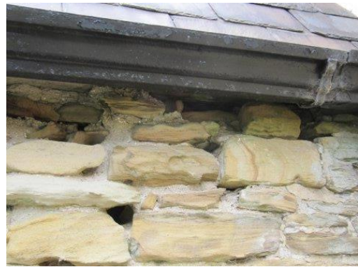
Deep cavities, open joints and weathered and missing stonework to East elevation of porch
