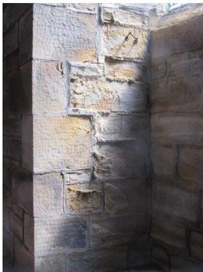
Salts, sanding stonework and loose pointing
