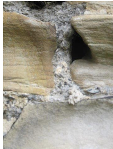
Deep cavity to South Porch wall
