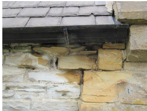
Salts, open joints and weathered stonework to West Elevation of porch
