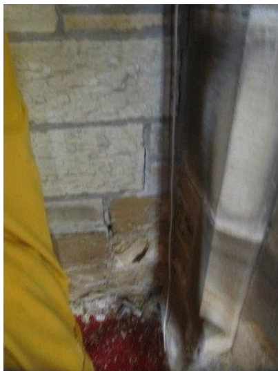
Damaged stonework behind curtain to East wall of North Aisle
