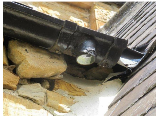
Loose and missing stonework to South Aisle and missing section of downpipe
