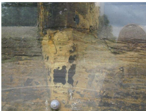
Damage to stonework to mullions of Northern Windows sheltered by window protection
