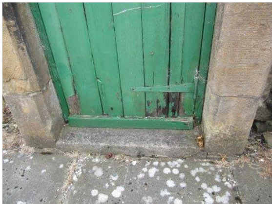
Damaged paintwork to door to old boiler room
