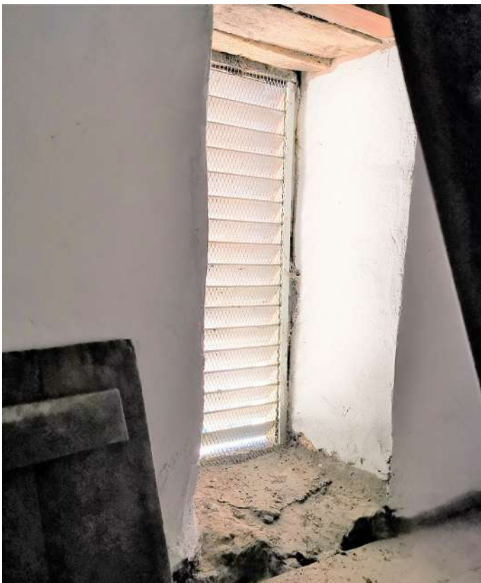
Lintels to south louvre still timber, in good condition. All others concrete. Metal grills in good condition, fixed securely
