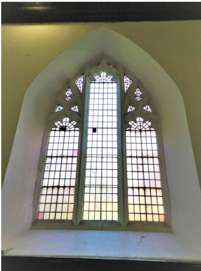
Window in north of nave has several broken square quarries and some leadwork distorted
