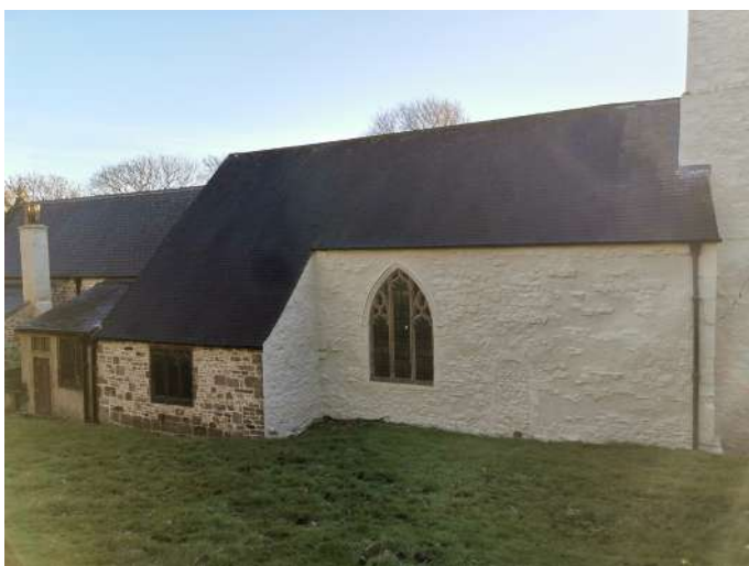
Nave roof with cat-slide roof over Thornley Porch - repairs required
