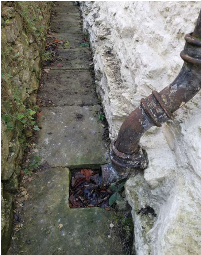
Gullies restricted by leaves, downpipe rusting
