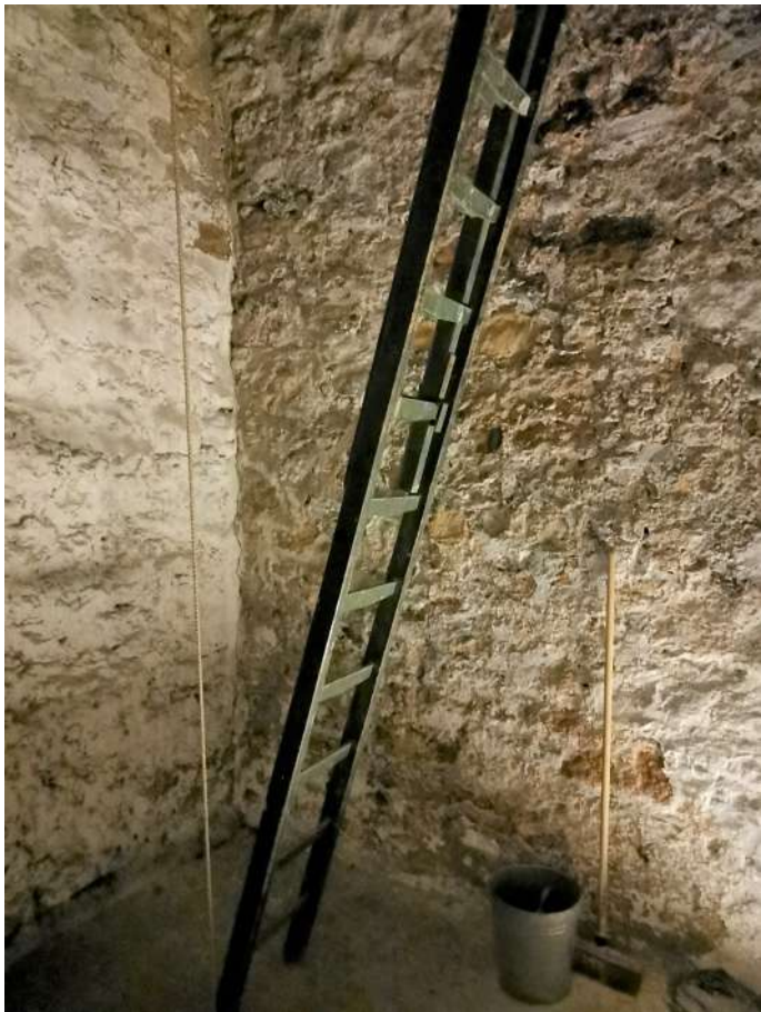
Cement pointing/render internally, north wall
