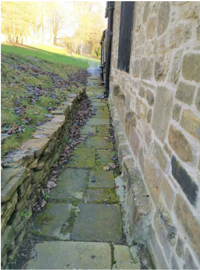
Hardstanding against base of wall will be trapping moisture - consider removal and laying grass directly up to base of walls
