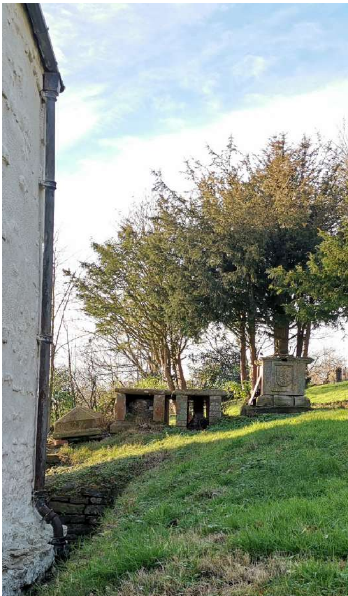
Tombs to north-west corner of tower in perilous condition
