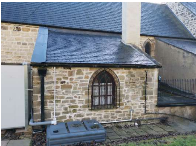
Vestry roof - damage to eaves at western end, and temporary covering to copings on east that require investigation and repair
