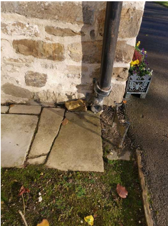
Porch downpipes discharge over ground
