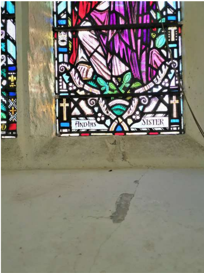
Impervious paint peeling in areas of damp or condensation, particularly noticeable at window surrounds. Minor cracking in several cills
