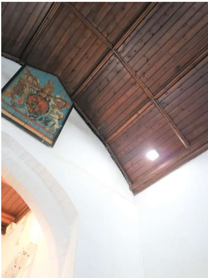
Nave ceiling boarded. Gap between ceiling and tower wall would benefit from clearing of debris and filling
