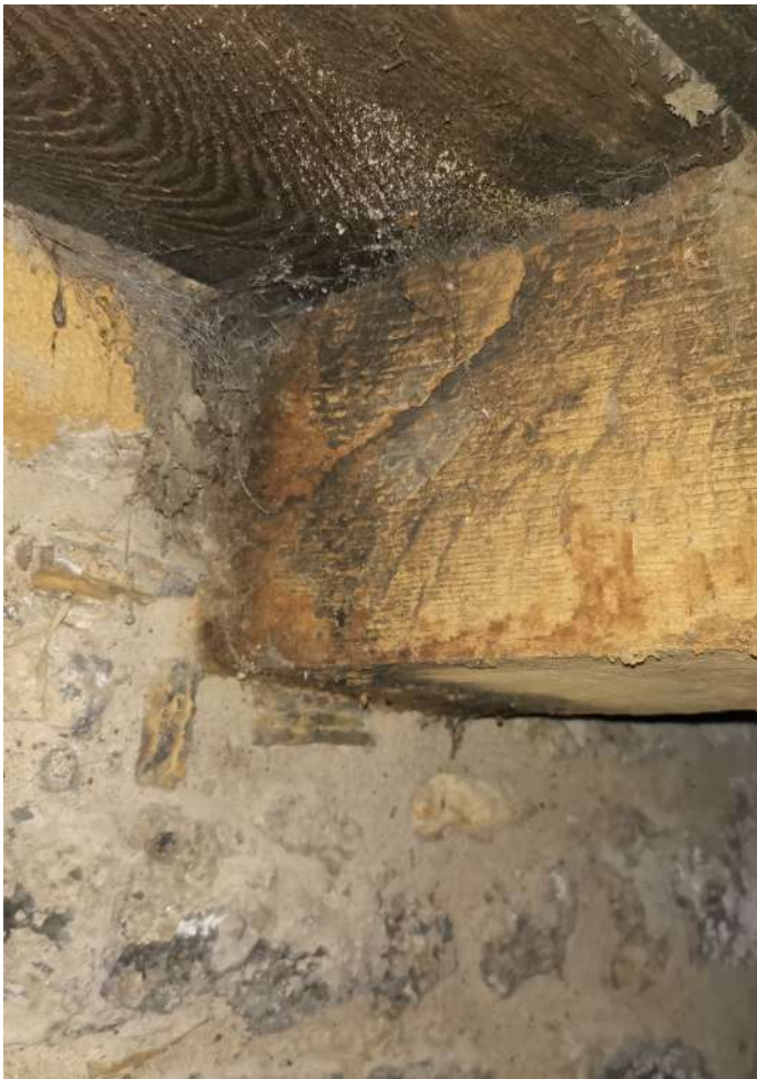
Timber joist embedded into north wall of tower damp
