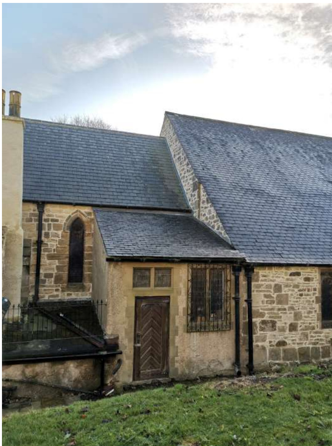
Organ blower and boiler room at lower level, both brick rendered in cementitious pebble-dash - require re-rendering in future
