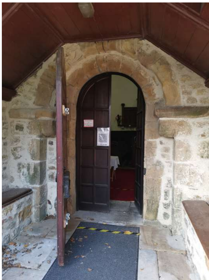
Flat central section of ceiling cuts off the top of the original round-headed opening of the medieval doorway. Consider reconfiguring ceiling, and possible removal or external door
