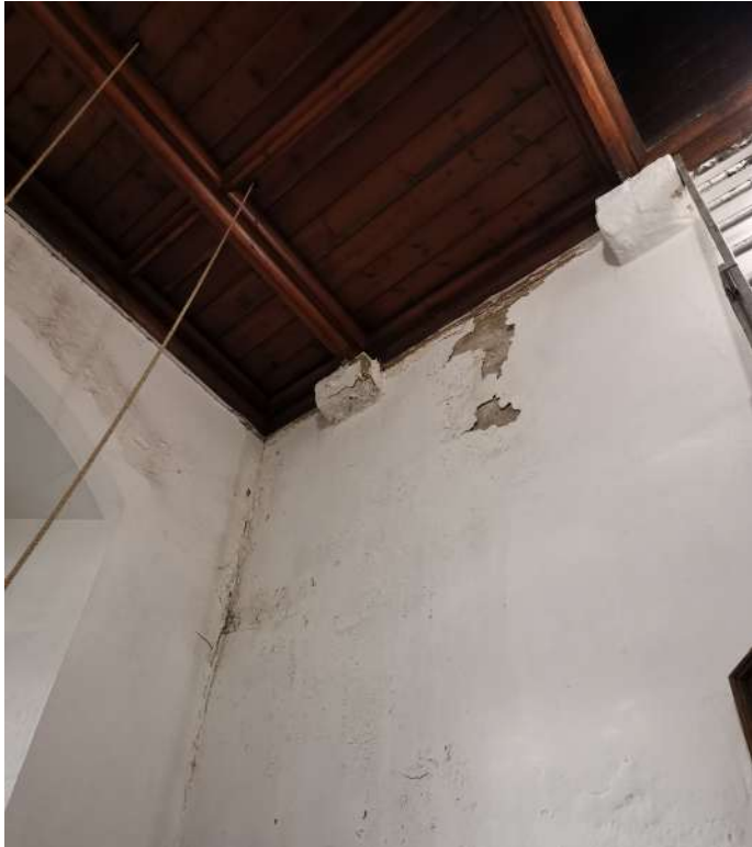
Peeling of impervious paintwork in tower - north wall, assumed drying out. Cement render internally in stage above requires removal
