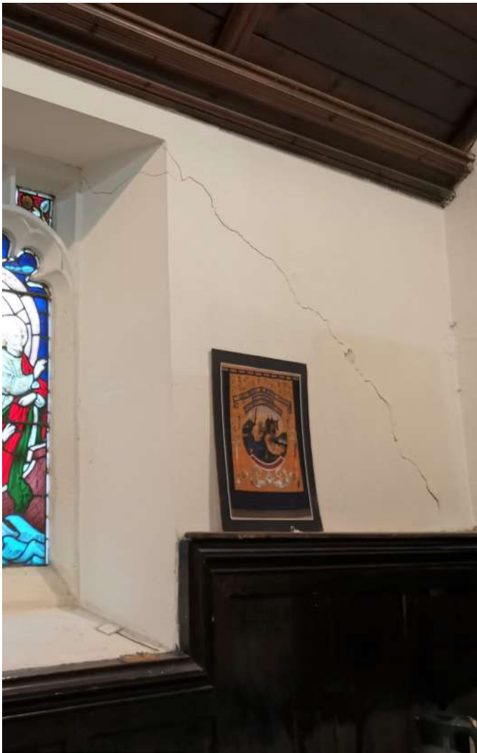
Crack to right hand of window in Thornley Porch
