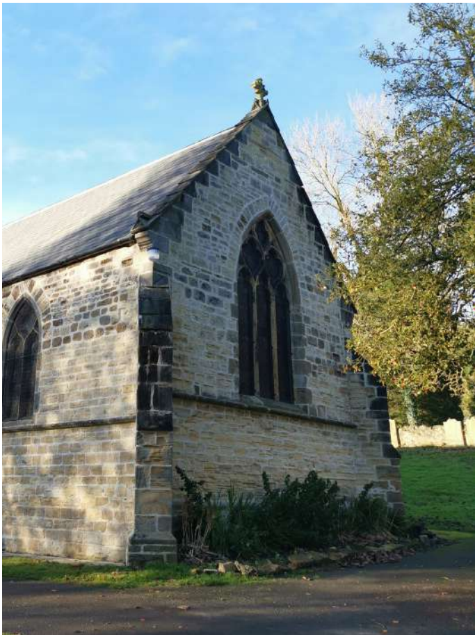
Main east elevation and principal east window. Minor stone deterioration
