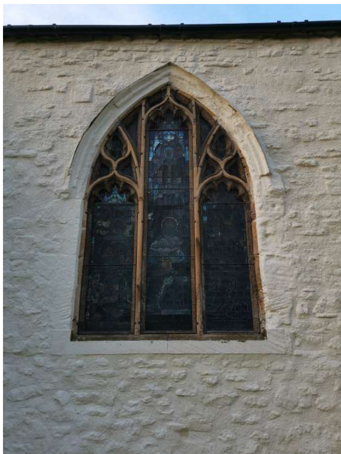
Window on south nave - stonework surrounds heavily deteriorated. Hoodmoulds now protected with lead
