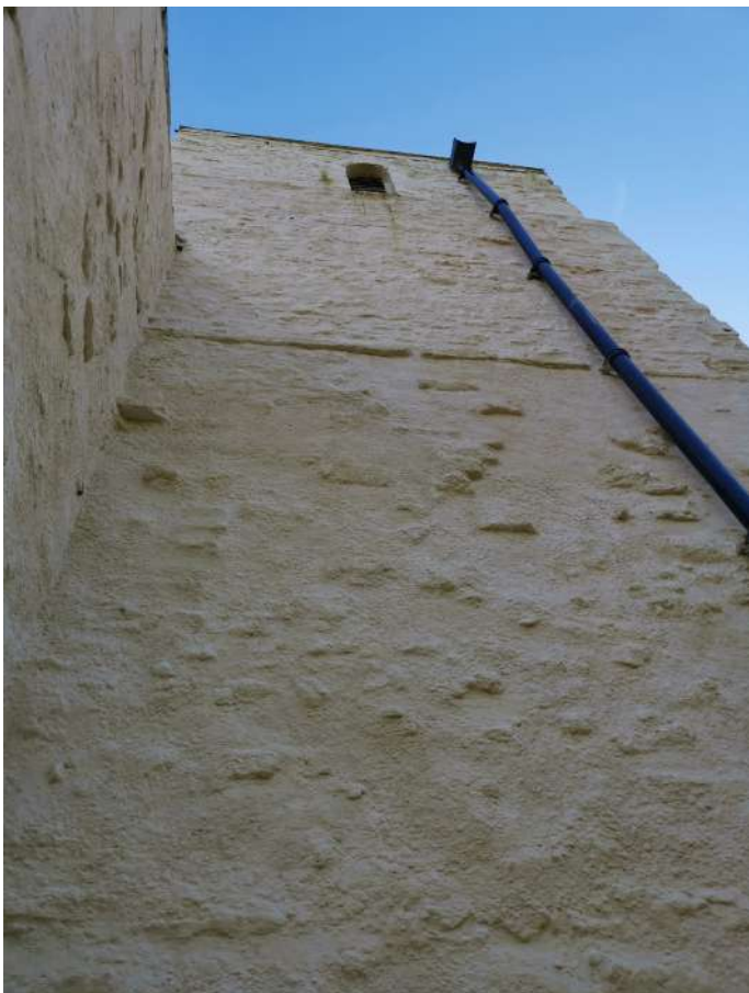
Heavily deteriorated masonry received mortar coating to bring out face and protect - all limewashed
