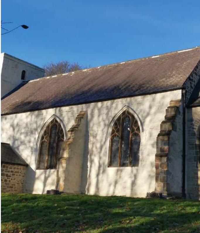
Hoodmoulds with mortar repairs and lead caps, but tracery and reveals still require repair
