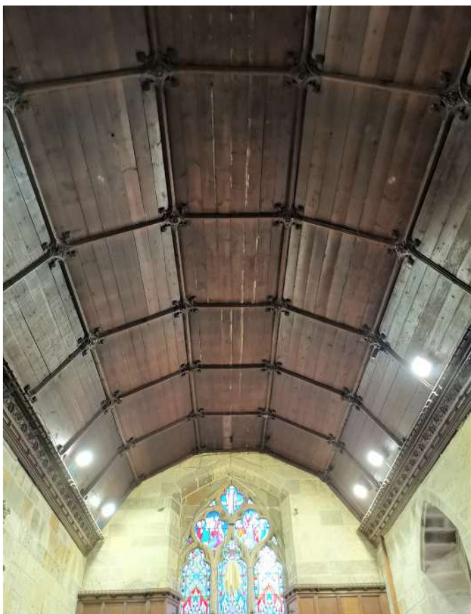
Chancel ceiling, water staining historic
