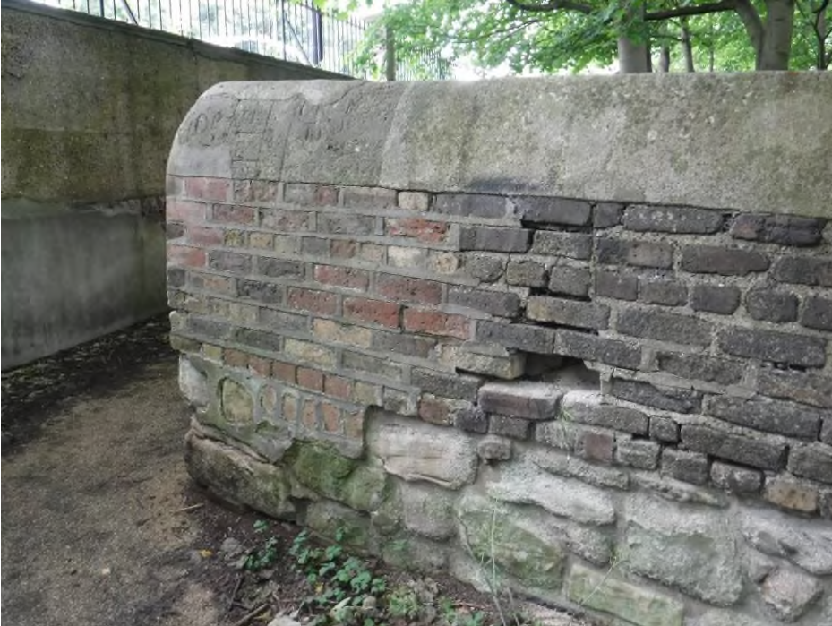
Brick erosion at sw corner
