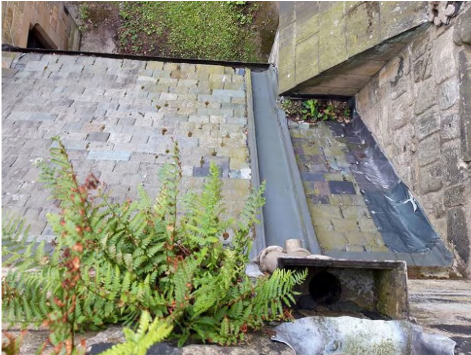
Back gutter clogged and high level planting.
