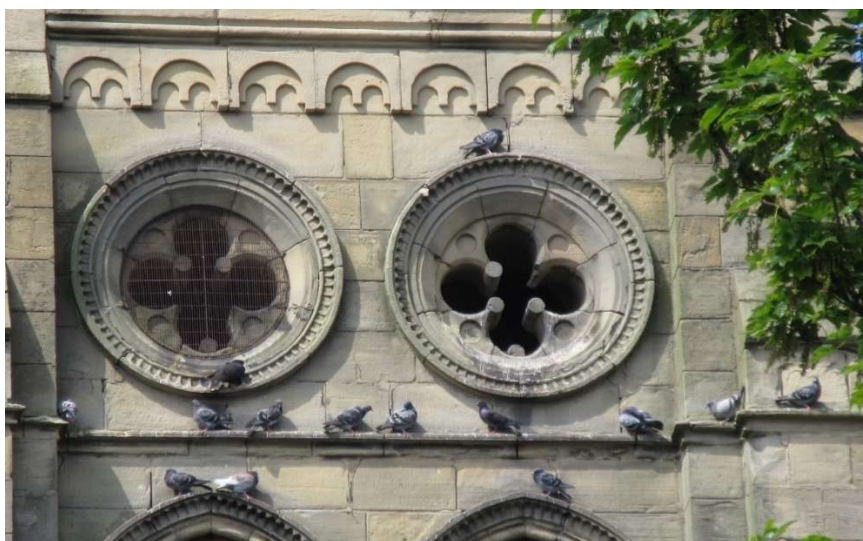
Mesh missing from one E round opening. It lies by the basement steps instead of keeping pigeons out
