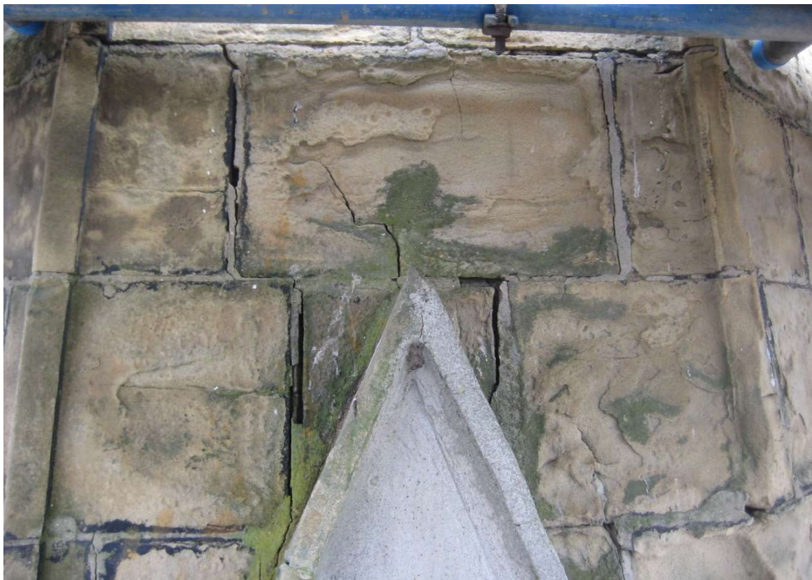
COMMON SPIRE DEFECTS 2011 photos – cracked stones and joints, past mortar patching at openings and further wind erosion
