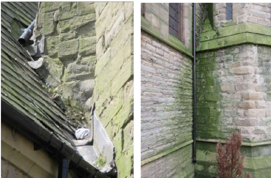
Plants in back gutters between Tower and Chancel and damp masonry between Chancel and Stair
