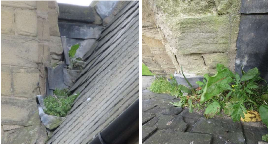
Blocked back gutters between Tower and Nave and deep decay at Tower SW buttress
