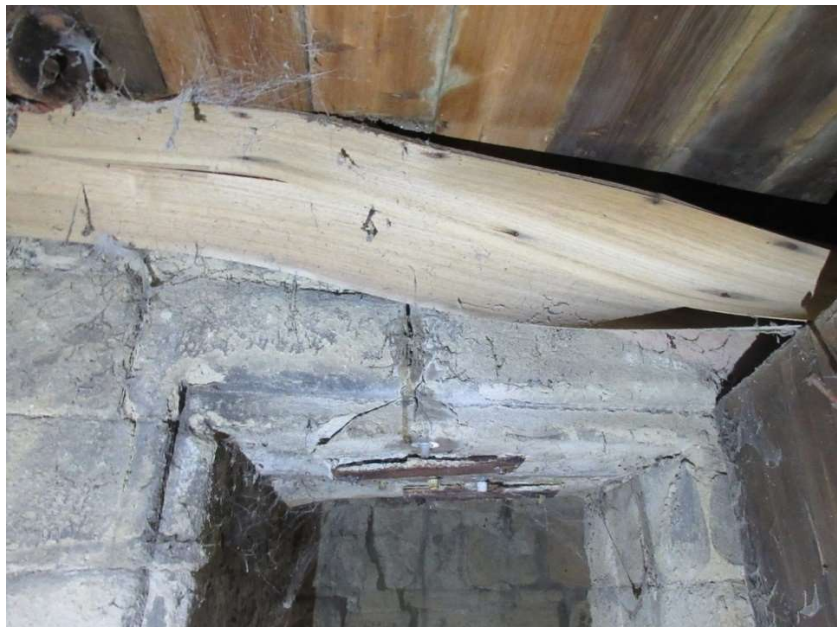
Cracked Lintel of Top Door from the Chamber side. Rusting steel plates no longer in close contact with Lintel. Board Ceiling patched over
