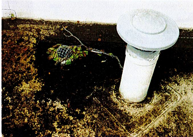
Debris around caged roof outlet before clearance and draining of the pond at inspection
