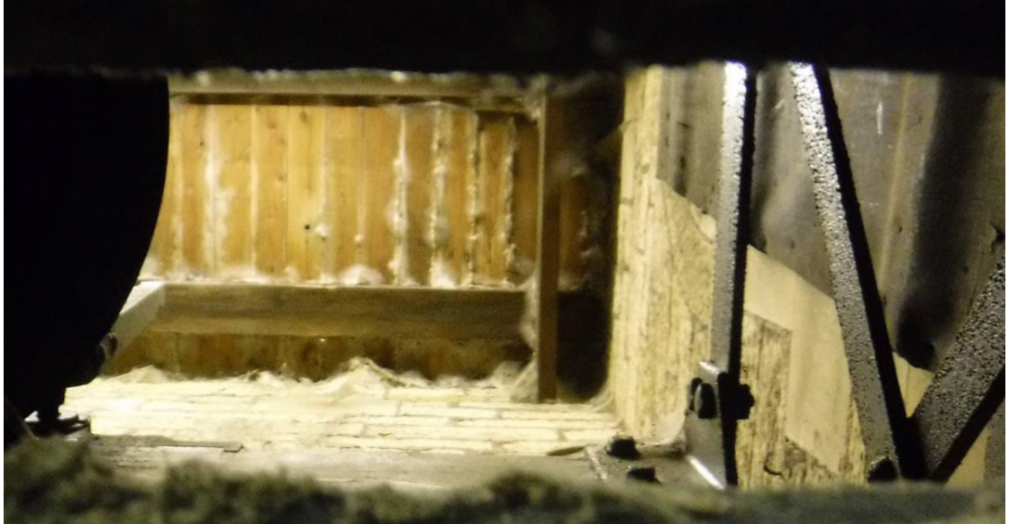
Belfry ceiling showing white marking suggesting guano build up and possible timber decay
