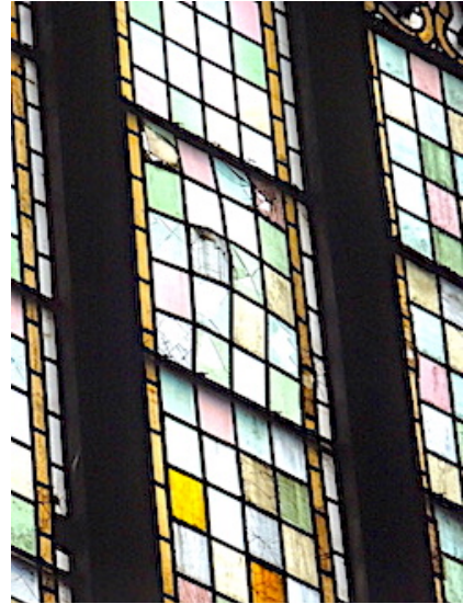
40. Nave north clerestory wall – glazing defects
