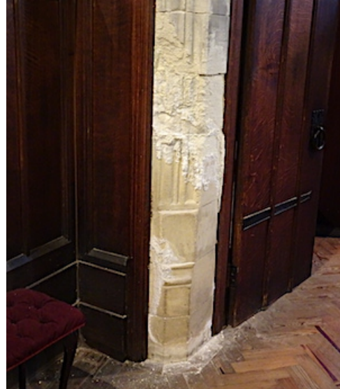
42. Lady Chapel – eroded stonework to east doorway
