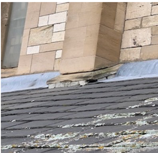
09 South Aisle roof junction with buttress – defective mortar.
