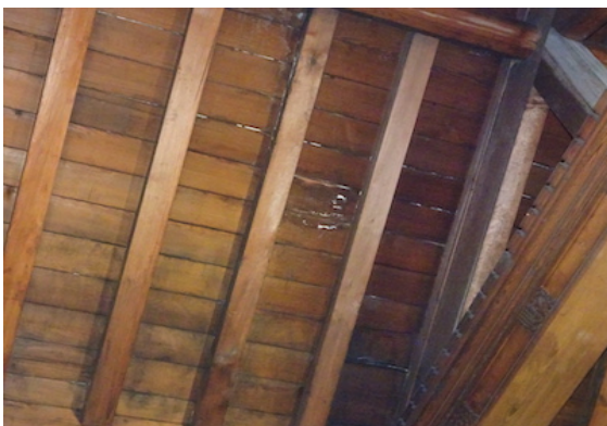
37. North Aisle roof – white marks/stains on boarding to note
