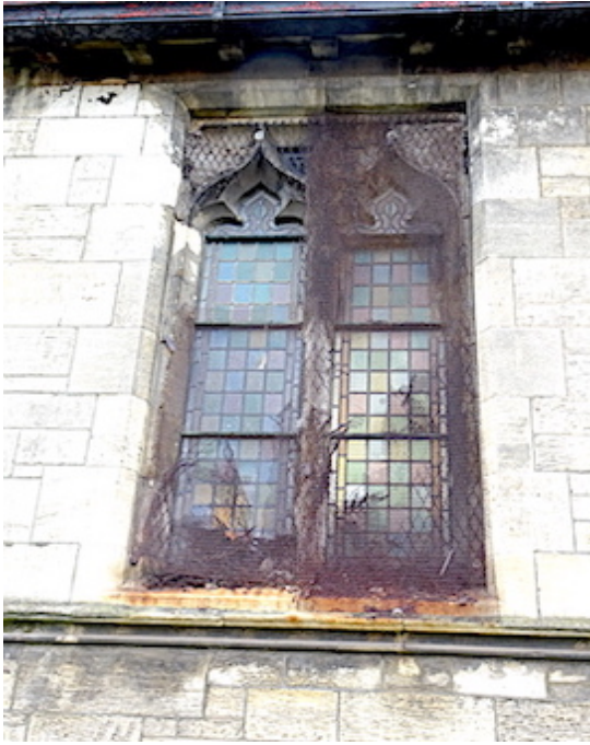
17. North Aisle window – damaged window guards
