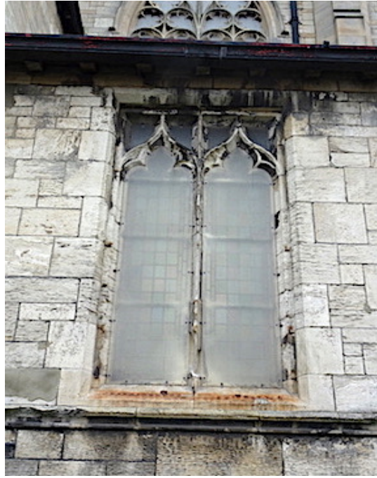
18. North Aisle window – damaged window mullion stonework
