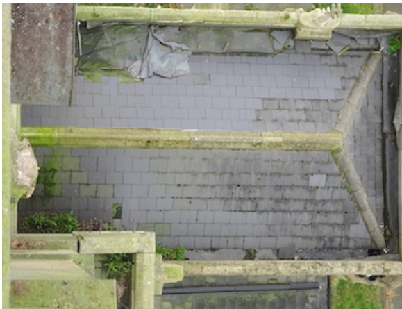
07 North Porch roof - slipped slates and temporary covers etc.
