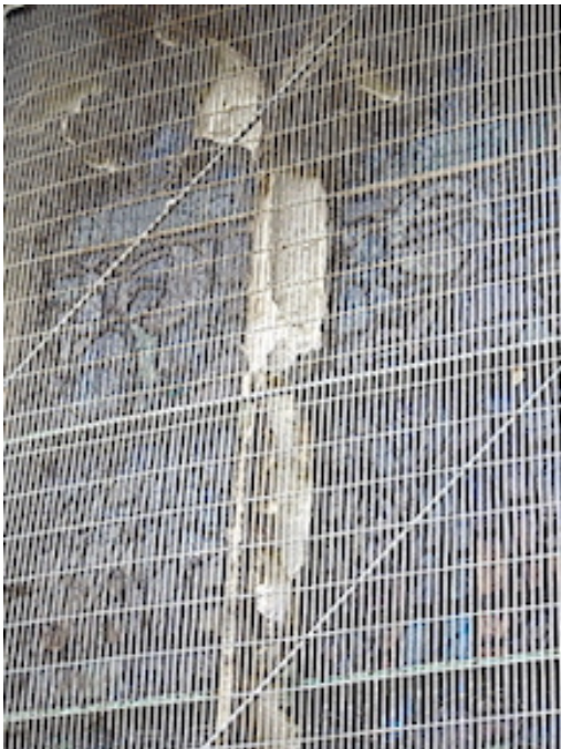
26. Lady Chapel south side–eroding window mullion.
