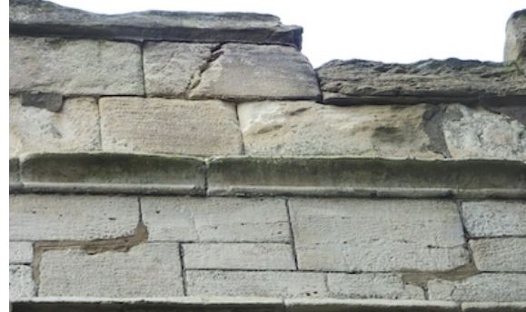
25. Lady Chapel south wall –eroding stonework
