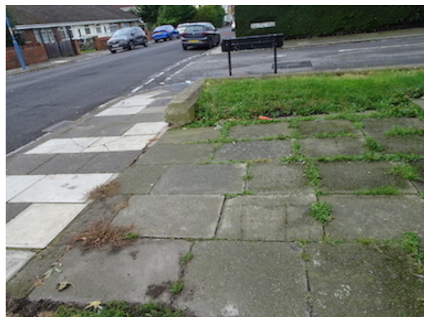
27. South entrance path – open joints and weeds.
