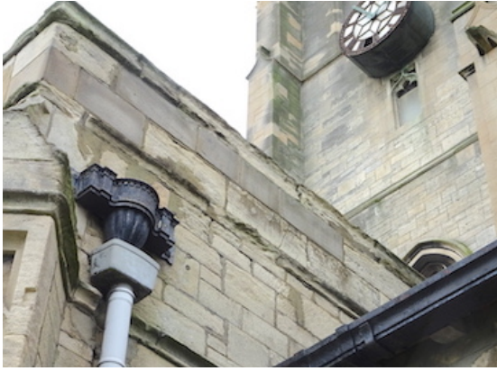
22. South Porch – east wall high level, eroding stonework
