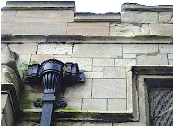
24. Lady Chapel south wall –eroding stonework & blocked hopper.
