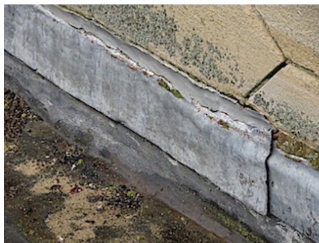
10 Tower roof north parapet – defective pointing
