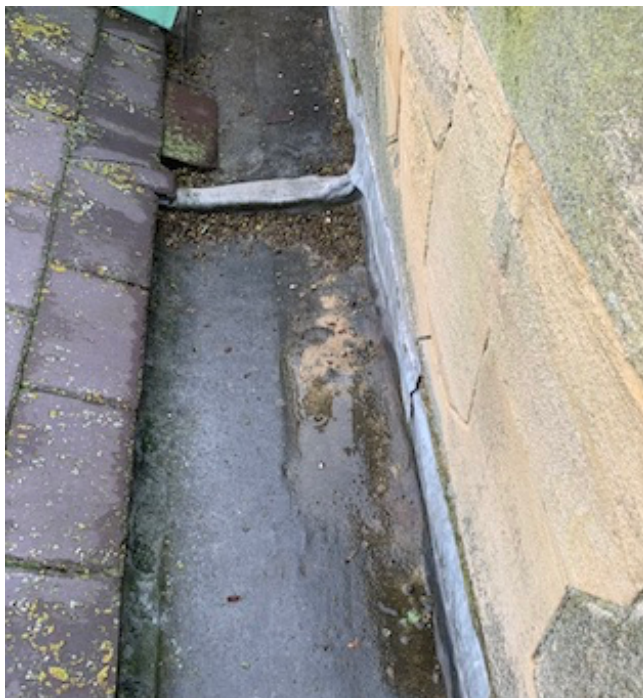
02 Tower Roof north side – sinking substrate in gutter below leadwork
