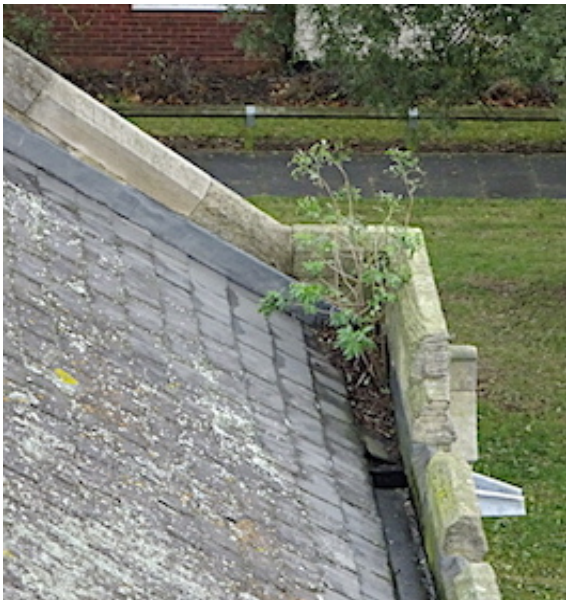
05 Nave roof south slope – tree growing at east end gutter!
