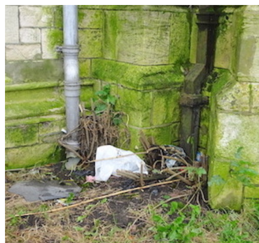
16. North Porch east face – growths at downpipe gully level
