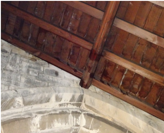
35. North Aisle west end – leaks from roof junction.
