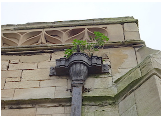
21. South Porch – blocked rainwater hopper on west face
