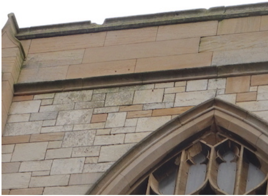
11. Nave north parapet – defective stones at coping
