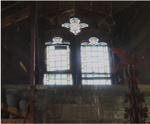
28. Tower upper part of base stage – window glazing defects.
