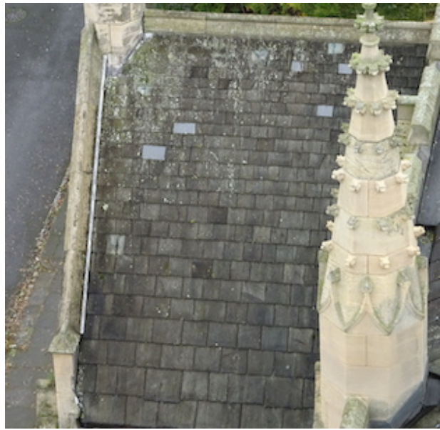
06 Organ Chamber roof west slope – slipped slates at ridge
