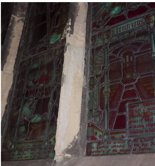
43. Lady Chapel – eroded mullions on south windows
