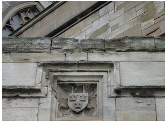
23. Lady Chapel Porch – eroding stonework above doorway
