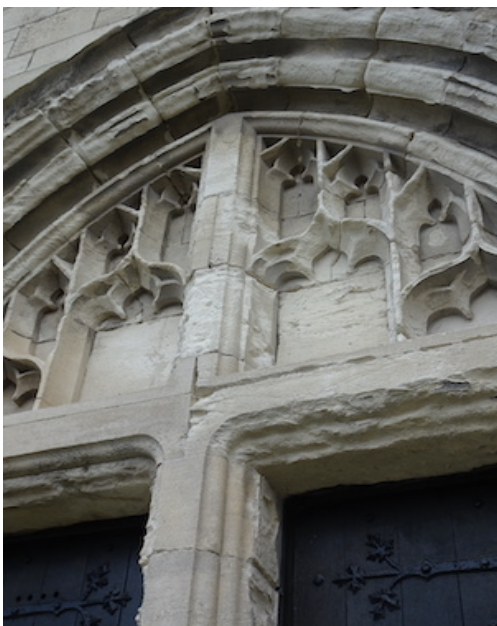
13. North Porch west face – eroded doorway stonework.
