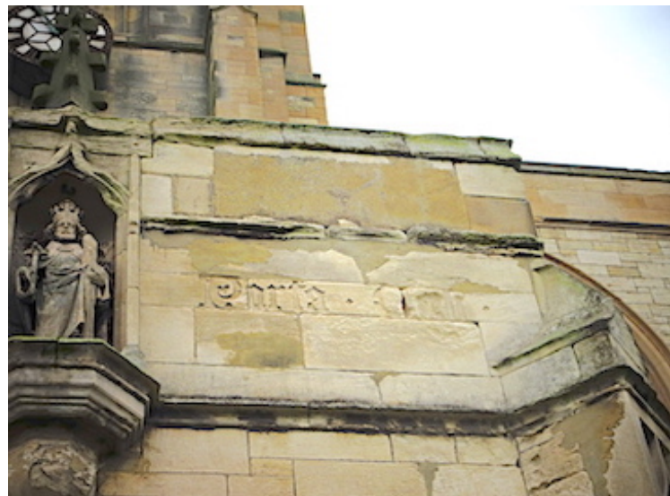
20. South Porch – defective stonework on south front
