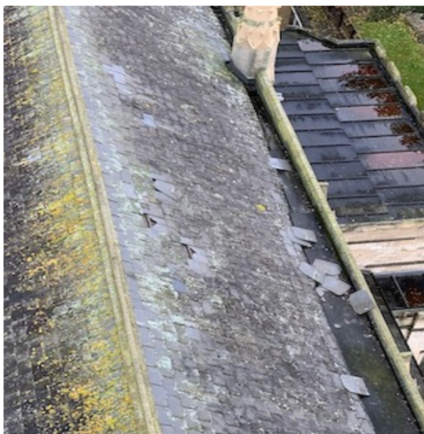
03 Nave Roof south slope – missing, broken or slipped slates.
