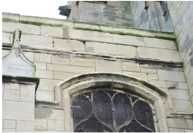
12. North Porch west face – defective and eroded stones and open joints
