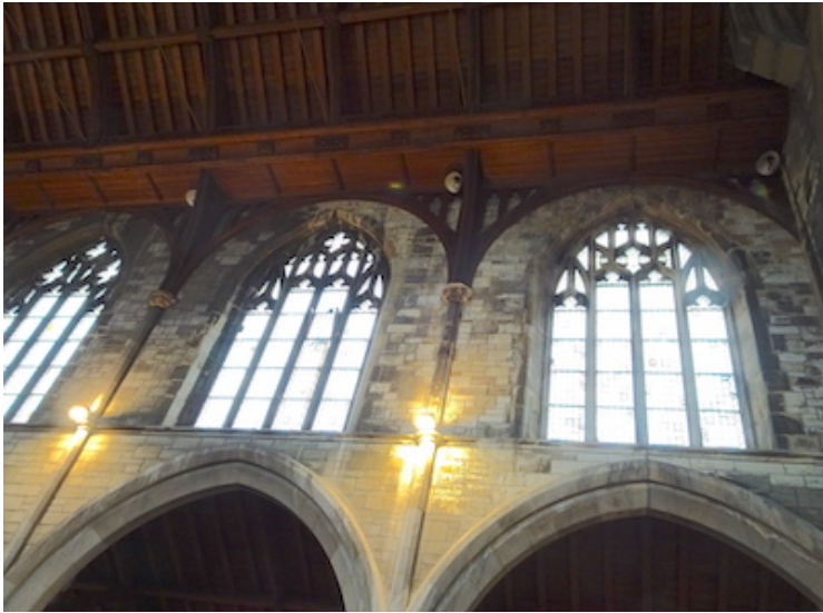
39. Nave north clerestory wall – stained stonework at high levels
