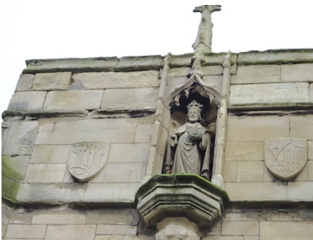
15. North Porch west face – eroded niche, label and pinnacle stonework.
