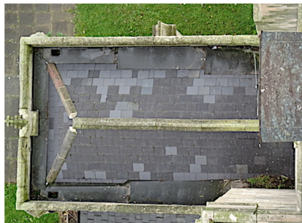
08 South Porch roof – grass build up at northeast corner gutter.
