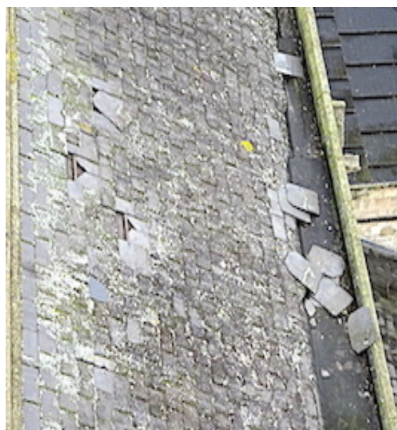
04 Nave Roof south slope – close up of slate defects.
