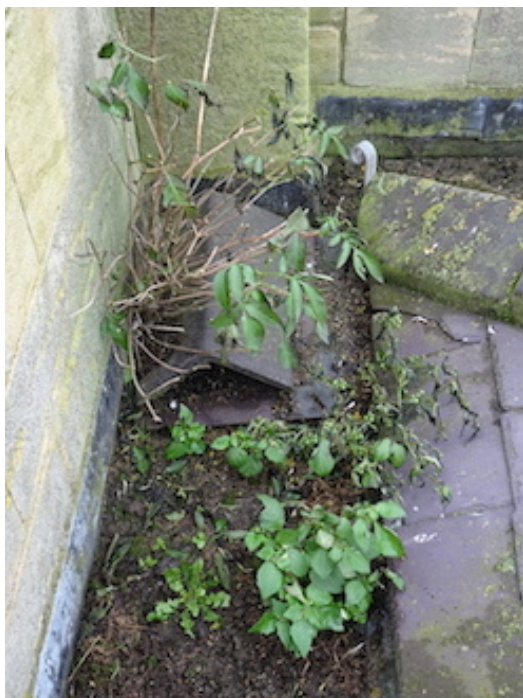
01 Tower Roof south side - blocked gutter and sump
