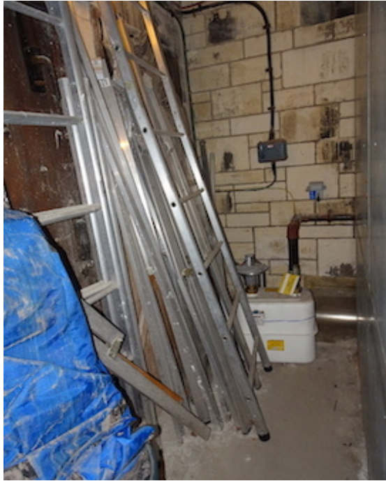
34. North Porch – gas inlet and heating chamber on right hand side with west doorway on left.
