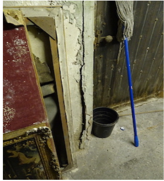
46. Passage below Chancel – defective reveal to east dooway
