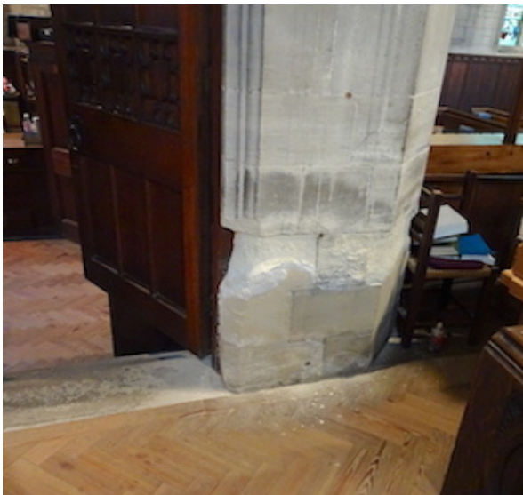
41. Chancel - north side doorway stonework decay down to Vestry
