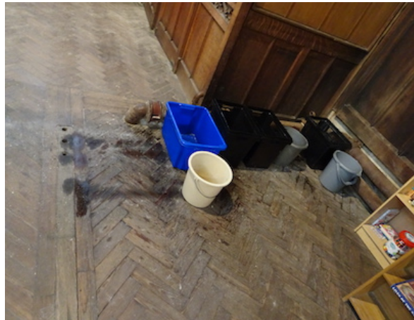
36. North Aisle west end – buckets catching the leaks from above
