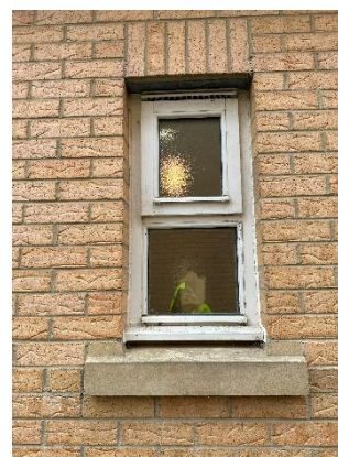
Figure 21 – Windows Require Decoration
