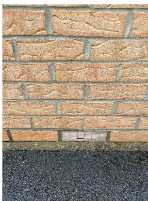
Figure 20 – Air Vents Below GL
