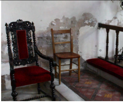
Blistering paint to Chancel
