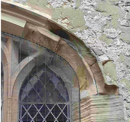
Deep decay to hood mould and arch to window s(viii)
