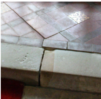
Sanctuary open joints to steps and unbonded tiling
