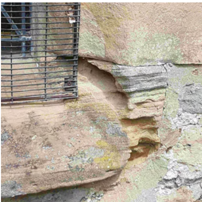
Deep decay to cill to window s(viii)
