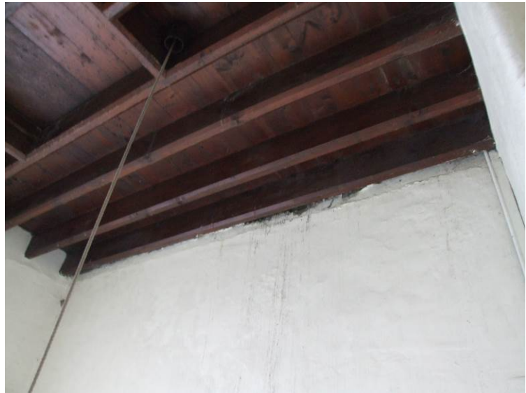
Underside of first floor lower level, showing water staining to north elevation
