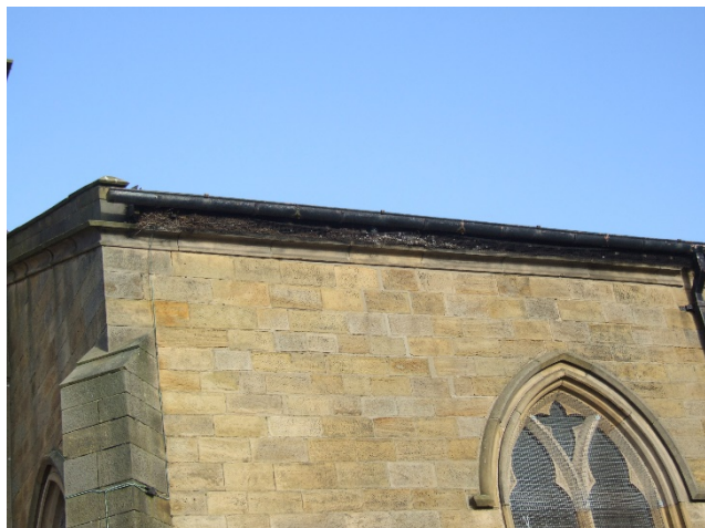
Nave south elevation; evidence of bird nesting
