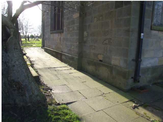
East end pathway; trip hazards
