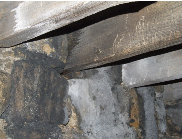
Tower parapet floor joists; damp to joist ends
