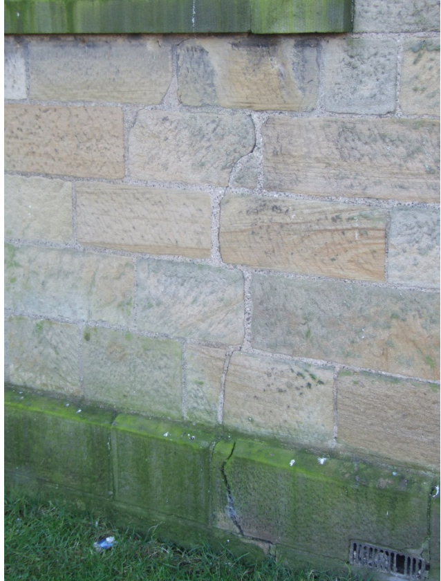
North elevation; historic movement cracking
