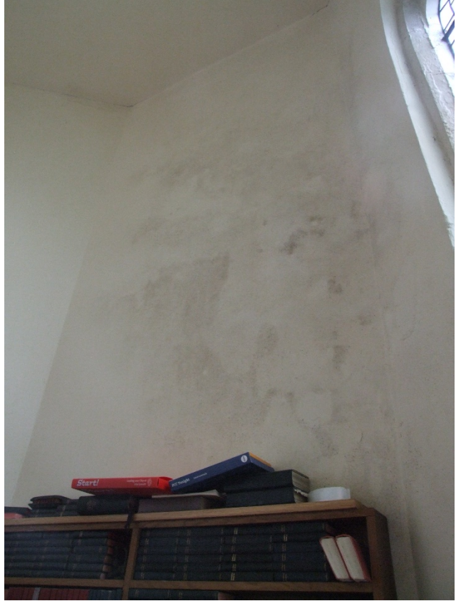
North vestry wall showing water staining
