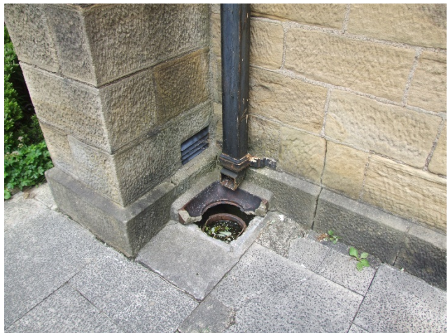
Damaged gulley, south elevation
