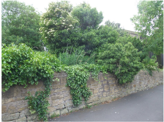
Ivy growth ultimately damaging to stone walling
