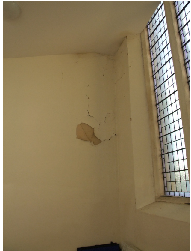
Meeting room; spalling plasterwork
