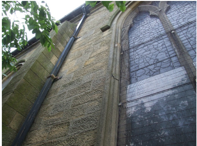
North elevation nave window; moulding cracking
