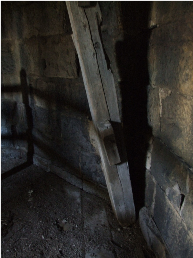
Disused/damaged access ladder within tower spire
