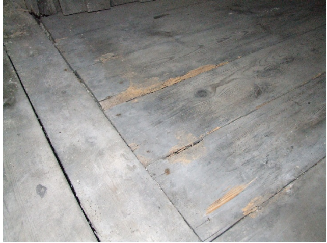
Woodworm to access floor; nave loft
