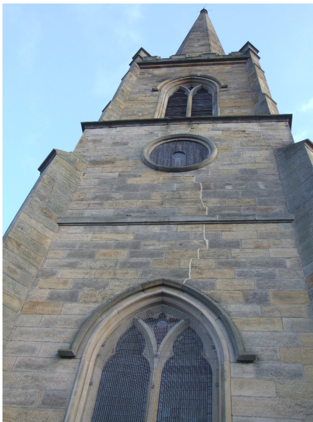
Tower, west elevation; historic crack pointing
