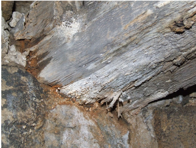
Tower parapet floor; principal beams showing advanced end decay
