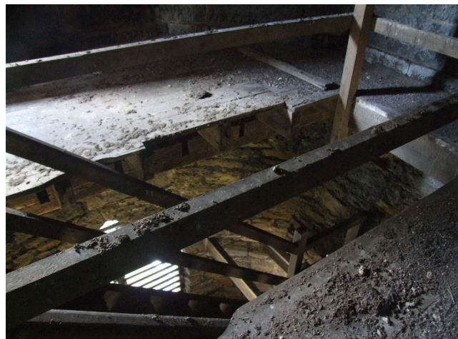
Parapet level floor; bird guano
