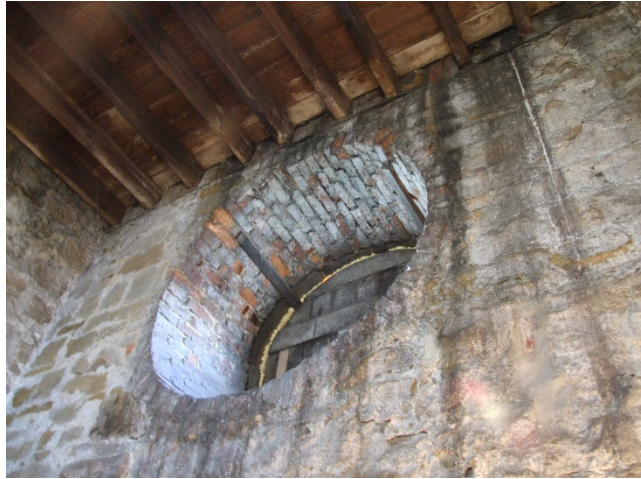
Tower: Historic water pattern staining
