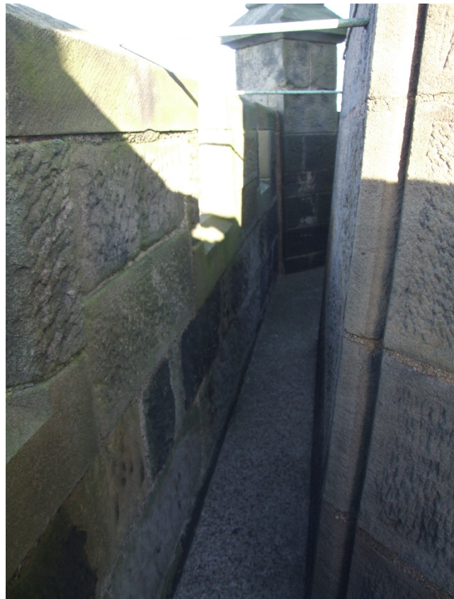
Narrow gap between parapet and tower spire
