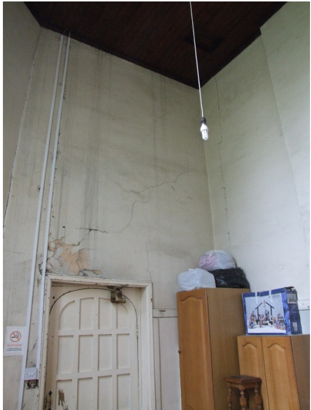
Cracking to west wall of vestry
