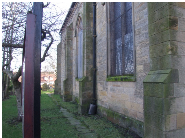
Northern chancel elevation; faulty gully
