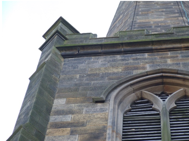
Tower parapet rainwater outlet; previous issues with blockage
