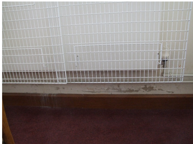
Meeting room; moisture indication to plaster
