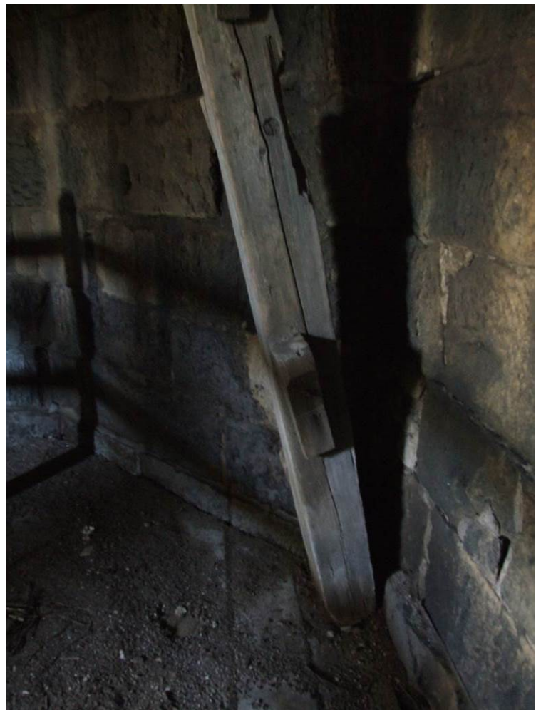
Spire access 'ladder' and debris
