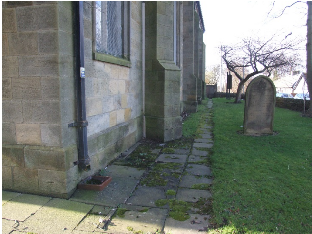
North end pathway; moss hazard (note proximity of trees)
