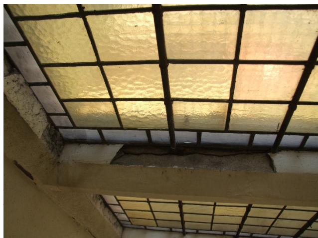
Meeting room; Missing pointing to glazing
