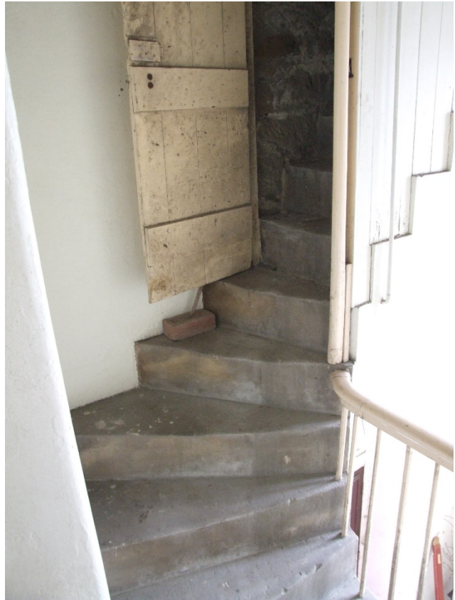
Inadequate guarding to tower stair
