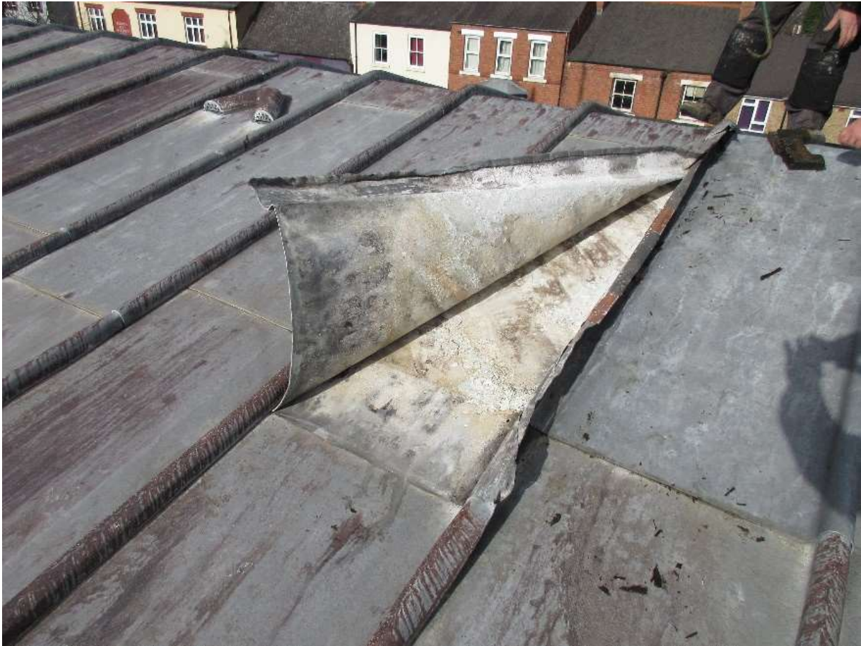
Heavy corrosion under a S bay near the Nave ridge
