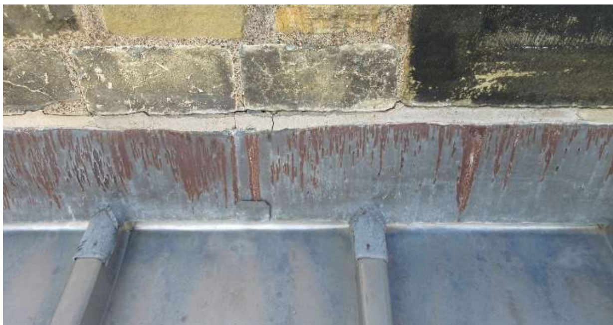
Cracked pointing at flashing at top of stainless Aisle roof
