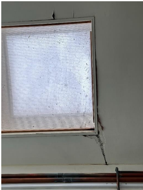
Figure 30 – Crack and leak rooflight 19
