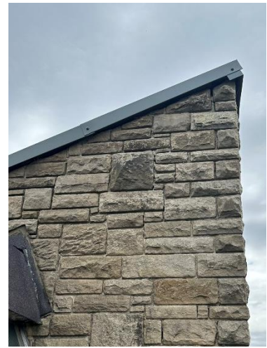
Figure 20 - high level open joints
