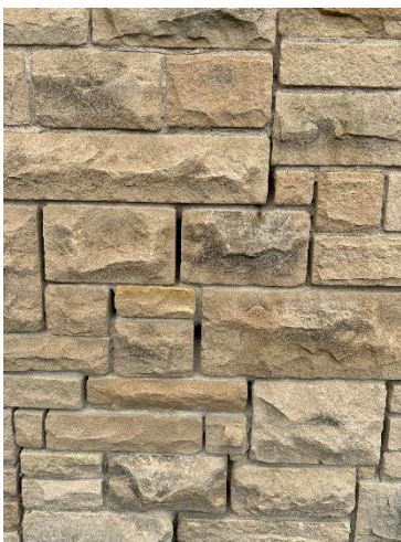
Figure 18 - mortar gaps at low level
