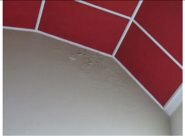
Chancel East wall – flaking paint through leak
