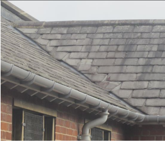
Slipped slates by valley of Organ Chamber roof
