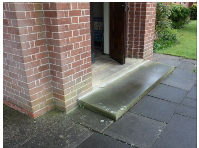
2No steps into Porch – consider re-laying paving flags to a gentle slope to give wheelchair access
