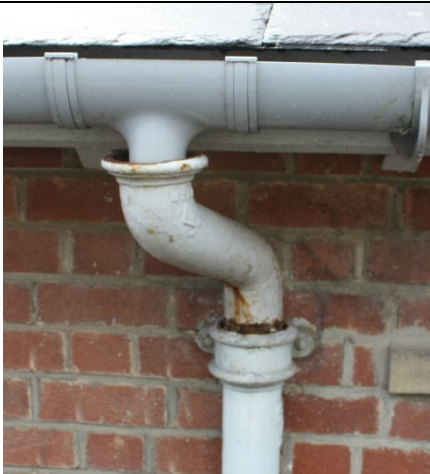
Rusting cast iron downpipe collars
