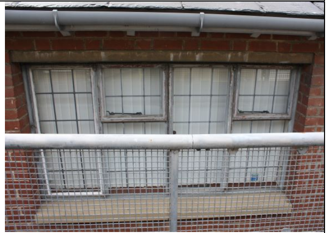
Rusting metal framed windows
