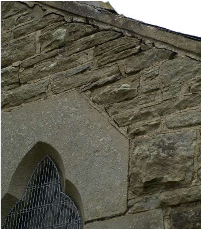
Cracked pointing and open joints will be contributing to the damp walls in the Vestry
