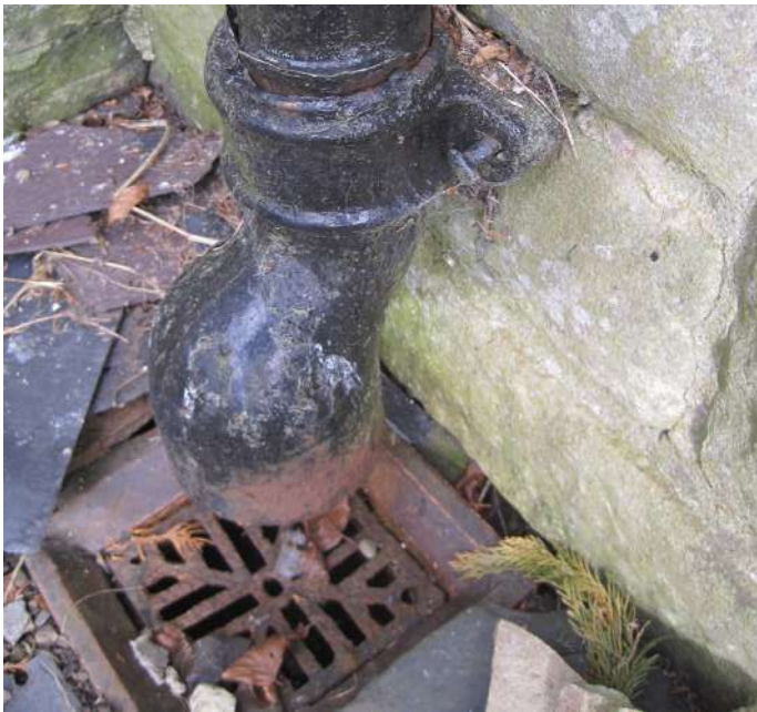
Some rainwater goods are rusting, and fixings are working loose
