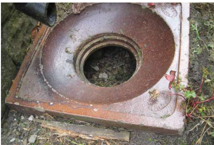
Rainwater gullies need to be kept clear of debris, and should have grilles fitted
