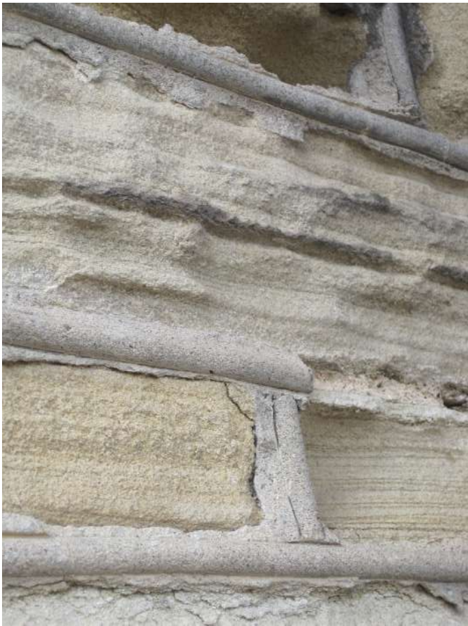
Walling stone suffering from differential erosion due to hard cement mortar. Where a danger to public, loose masonry should be brushed down and any larger pieces gently pulled away using fingers
