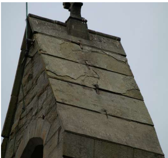
The masonry of the bellcote in reasonable condition, apart from shaling and opening of joints in the water-tabling
