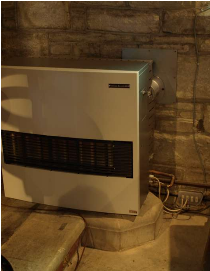
Two new gas convector heaters fitted October 2021.
