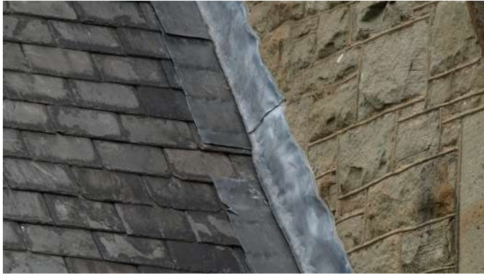
Slipped soakers to extension roof.
