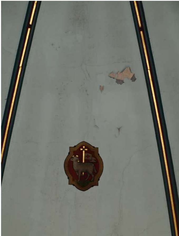
Cracking and loss of paint from Apse ceiling
