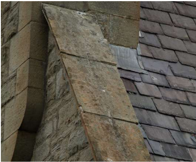
Displaced water-tabling to Nave verge, and loss of pointing from joints
