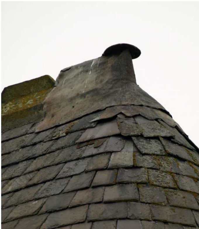
Several slates on curved apse are displaced and need to be relaid. The lead finial would benefit from renewal
