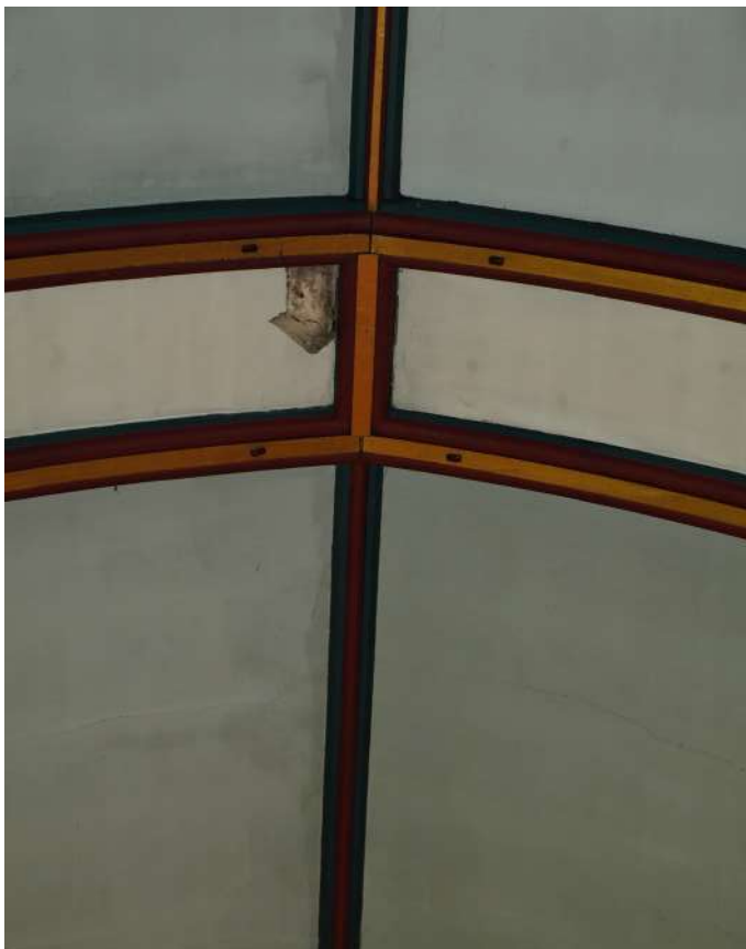
Minor loss of plaster at the junction of Nave and Apse
