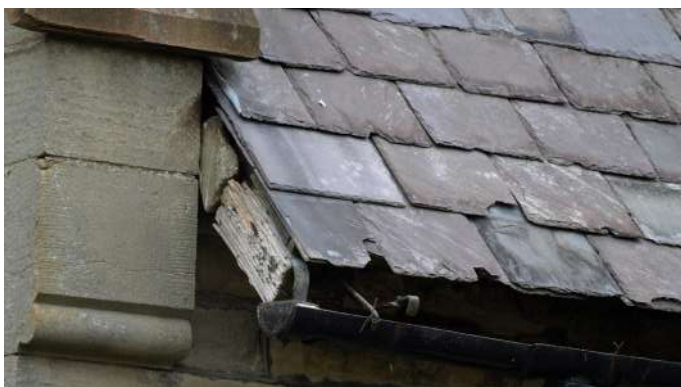
Decayed rafter end to Nave roof above Porch, and damaged slates
