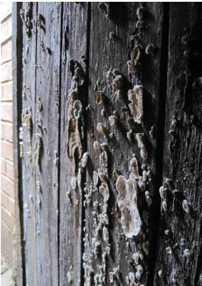
Original boiler room under south porch - door is decaying due to damp. Improve the ventilation
