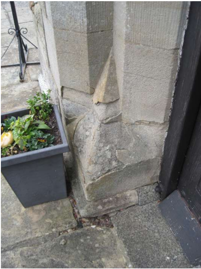
Delamination of soft sandstone jambs to the main church doorway
