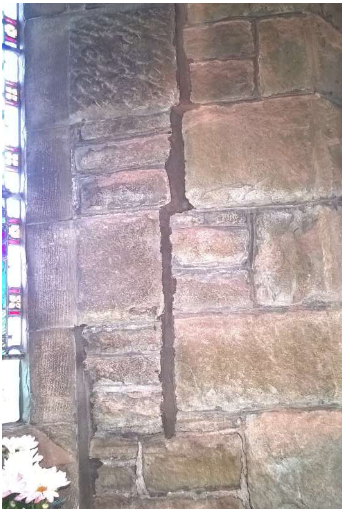
Historical cracking, repointed, to Nave window.
