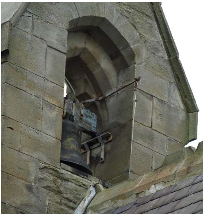
Bell headstock is decayed. The whole mechanism requires overhaul
