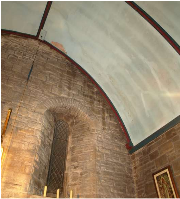
Loss of paint and water staining to the west end of the Nave
