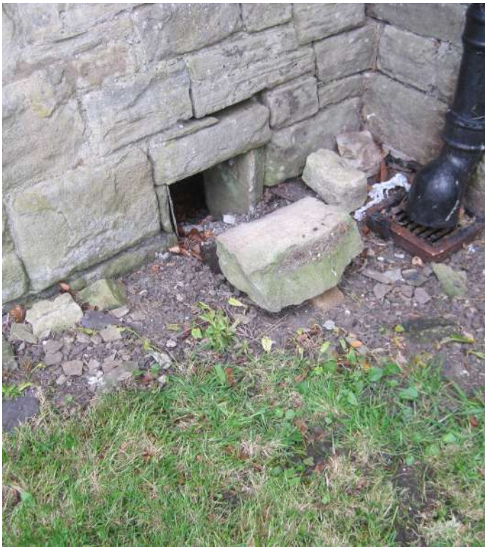
Vent to the former boiler room - needs to be kept clear. Fit a cast iron grille, and keep vegetation clear.
