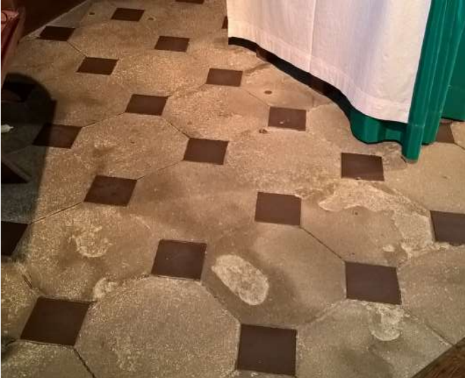
Stone damage to floor in sanctuary, as well as damp showing through - investigate construction of floor build-up
