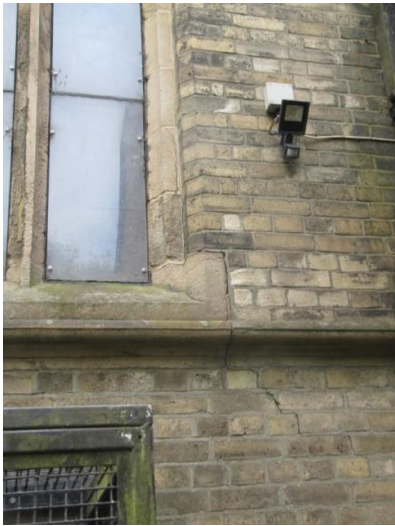
Cracking to North Elevation of the Chancel
