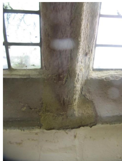
Failed coating and stonework behind in the Vestry.
