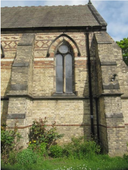
South Elevation of the Chancel currently being monitored due to movement
