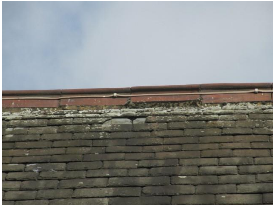
Slipped slate and missing mortar to ridge to Nave
