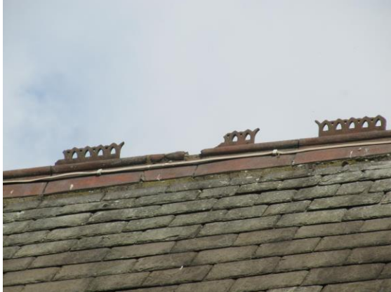
Weathered ridge tiles to the Chancel roof
