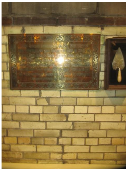
Cracking to West wall of the Nave
