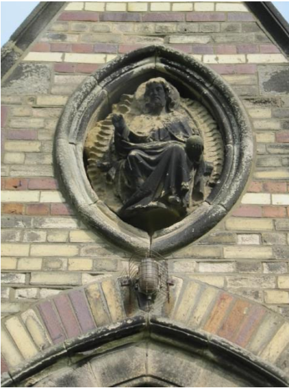
Weathered stonework to the carved stone Christ in mandorla
