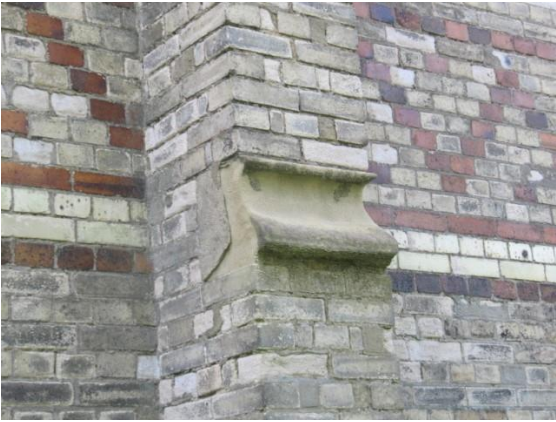
Weathered stone to North Aisle buttress
