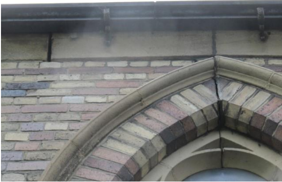
Cracking to North Elevation of the Chancel Of the Chancel
