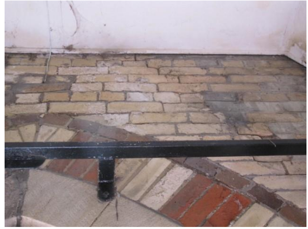
Salts and damaged bricks to porch over main door
