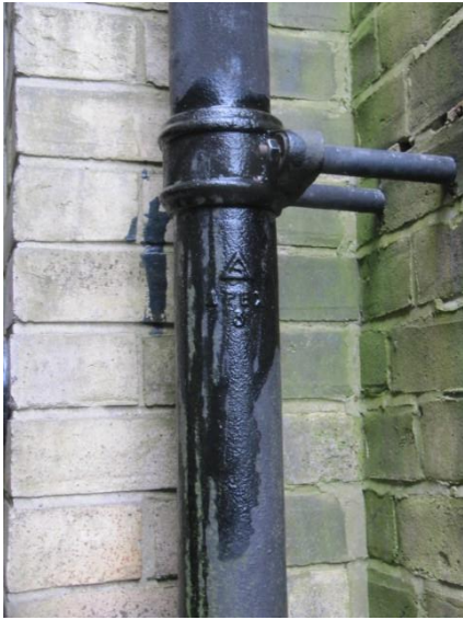
Leak to Downpipe by rear entrance door
