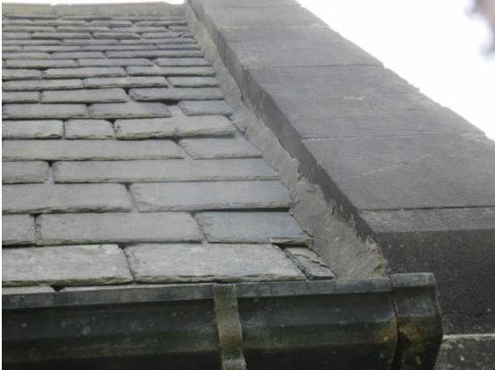
Cracked mortar fillet to porch roof
