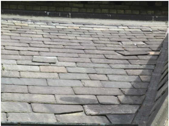
Slipped slates to South Aisle roof
