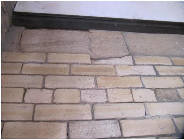
Weathered stonework to porch
