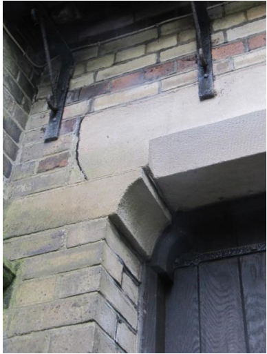
Cracked Lintel to rear entrance door
