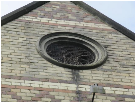
Damaged mesh to opening on the East Elevation Of the Chancel
