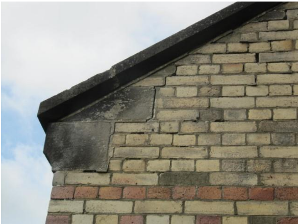
Crack to East elevation of the South Aisle
