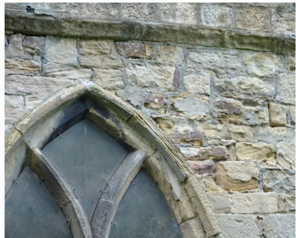
North Aisle north wall - eroded and laminating stonework
