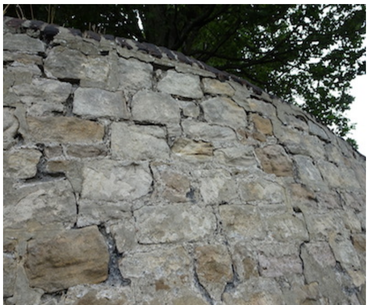
Churchyard wall south east corner – open joints
