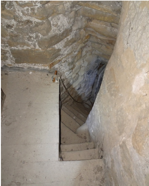
Tower bell chamber access – no guard rails
