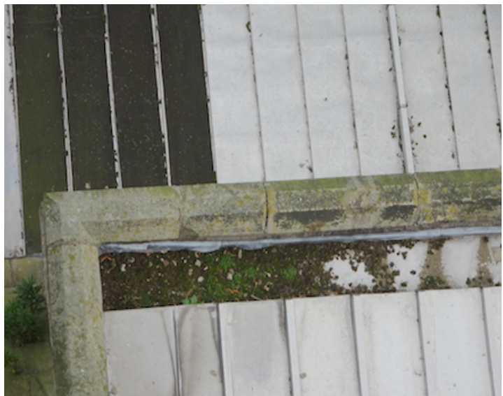
North Nave – gutter debris at west end and open coping joints
