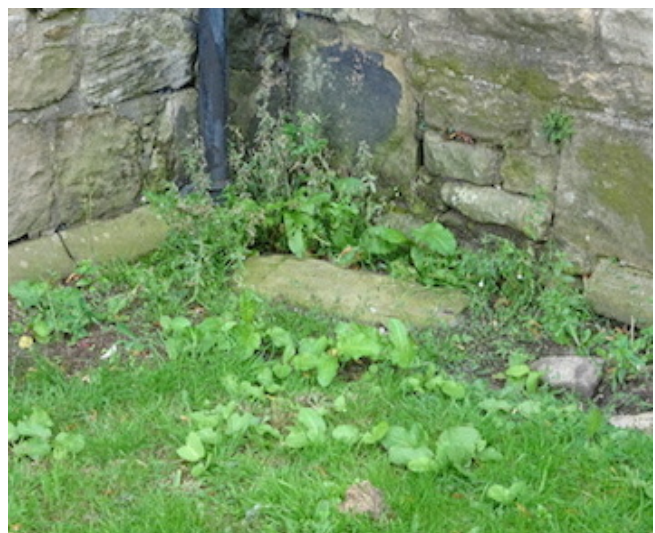
South Porch wall base – overgrown gully at north west corner
