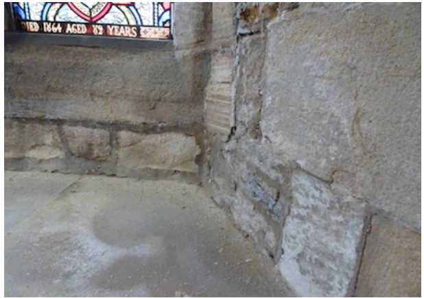
Chancel – open joints at window sill reveal on north side
