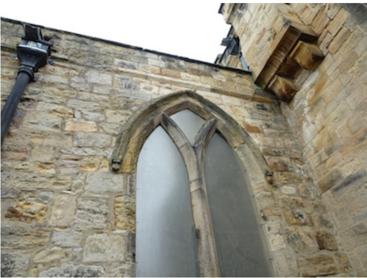
South Aisle and South Junction – eroded stonework and open joints at high and low levels.
