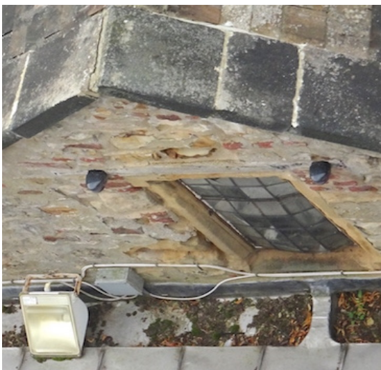
South Porch north wall – buckled glazing and poor stone
