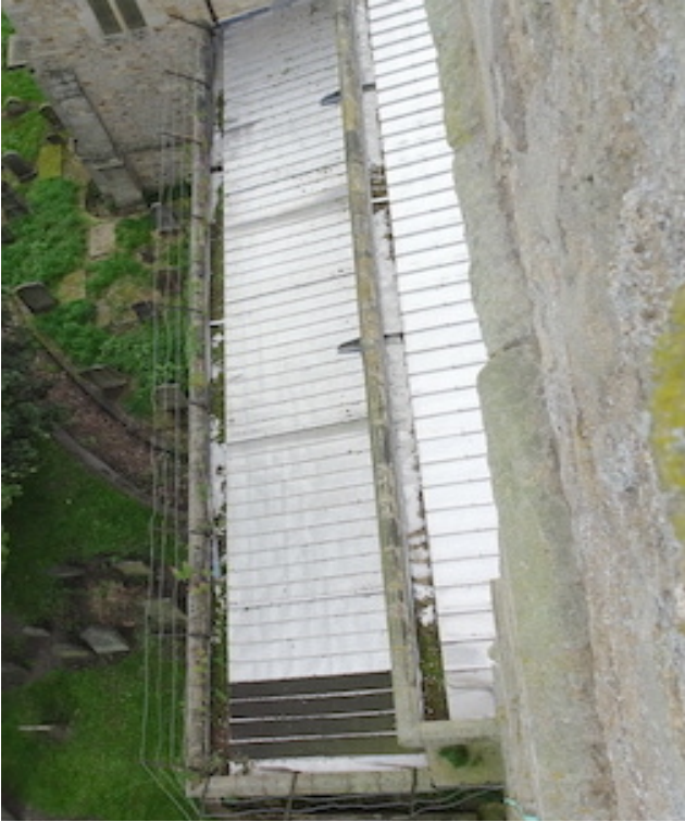
North Aisle roof – vegetation in north parapet gutter
