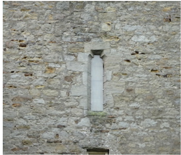
Tower north face - eroded pockets in masonry
