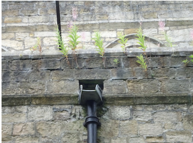
North Aisle north wall - vegetation and open joints at parapet.
