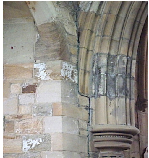
Nave - Chancel arch north side, signs of damp
