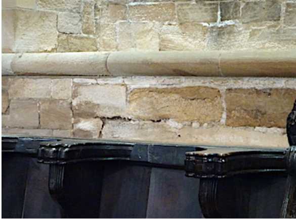
Chancel – open joints above choir stalls on north side
