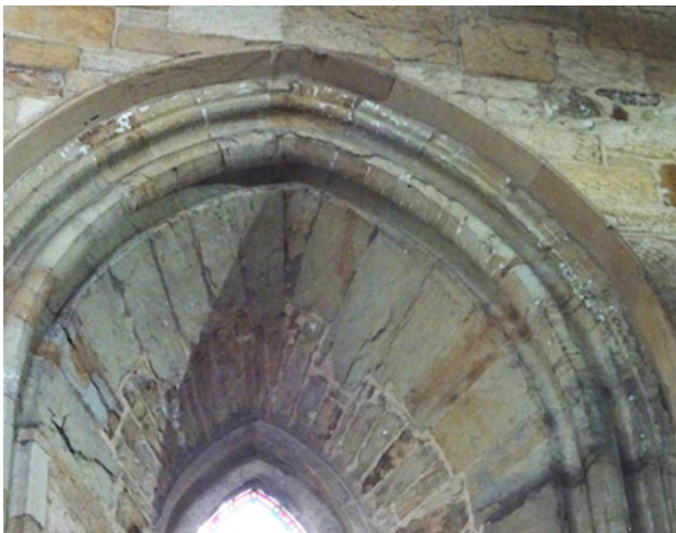
North Transept - cracked and laminating stone to north window.
