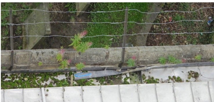
North Aisle gutter – flashings adrift at north wall
