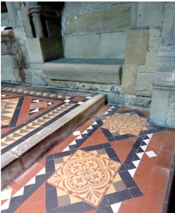
Chancel – open joints to masonry south wall
