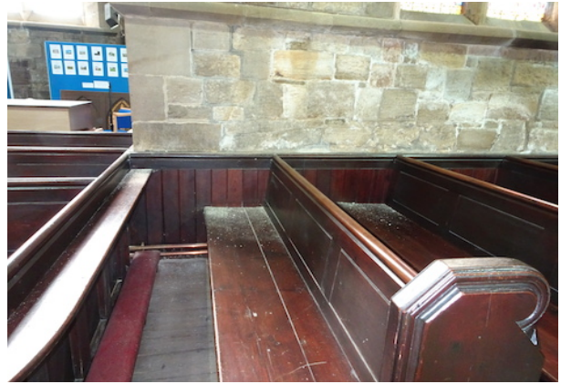
South Aisle – salts escaping at low level - stone dusting on pews
