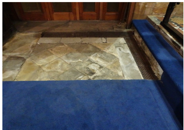
Chancel – rising damp to floor slabs in front of Sanctuary
