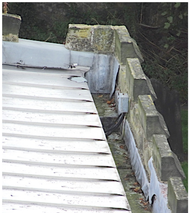
Chancel roof east and south parapet – loose non-lead flashings
