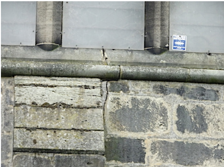
Chancel East gable - fracture in sill level
