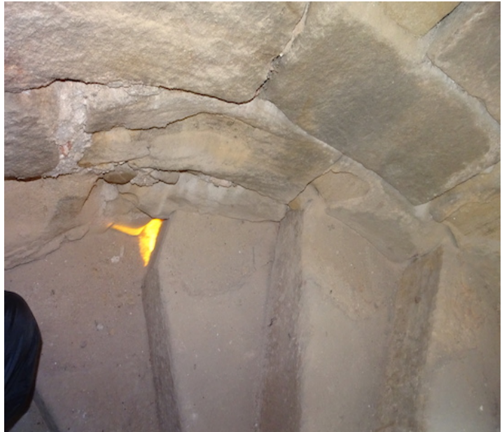
Tower staircase – gaps between stone treads and dusting of surfaces
