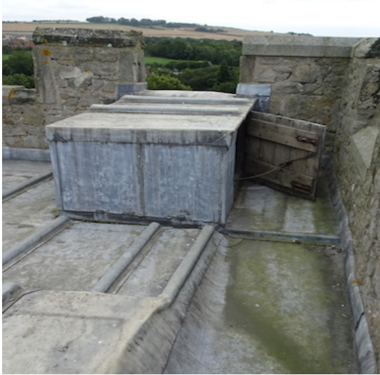
Tower roof – awkward access onto roof defective door.
