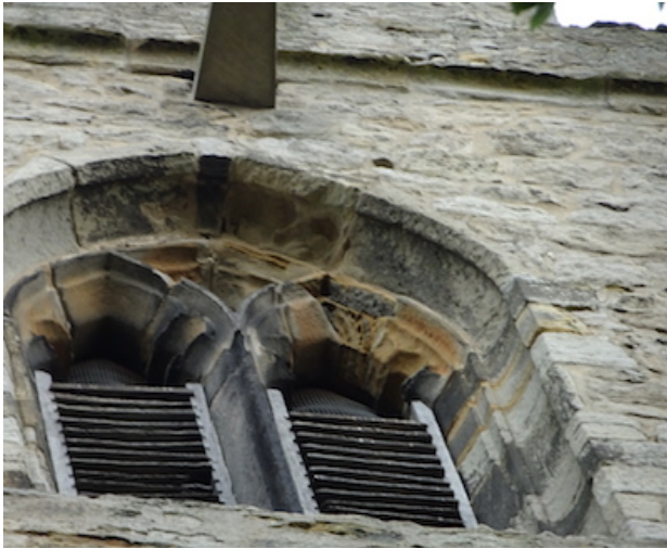
Tower north face - bell chamber eroded window masonry
