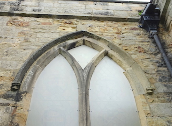
South west Aisle – poor stonework to window arch heads
