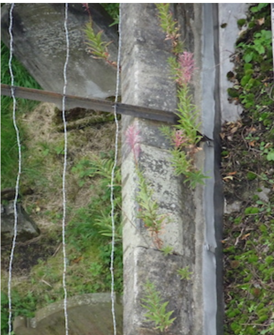
North Aisle roof north parapet – vegetation on coping
