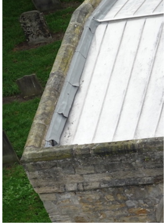
North Transept roof – deformed non-lead cover flashings
