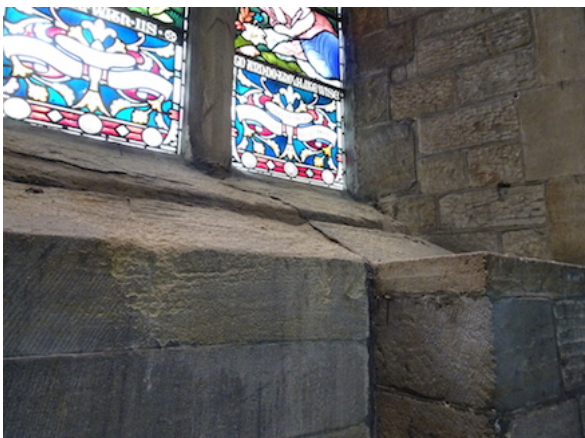
Chancel – south wall lamination and fracture to window sill
