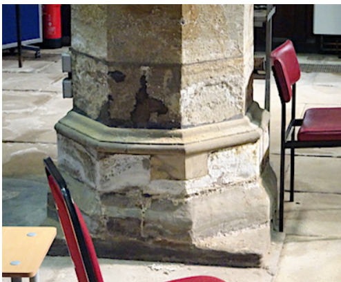
Nave – typical rising damp to column base
