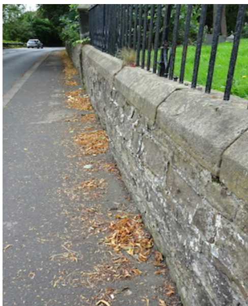
Churchyard wall east side – open joints and bulging.
