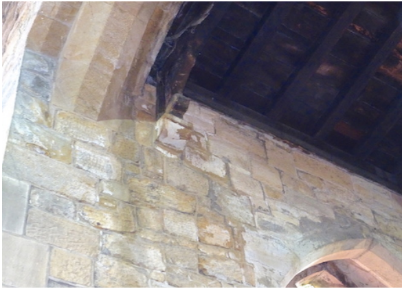
South Aisle – signs of water ingress at ceiling level east end.
