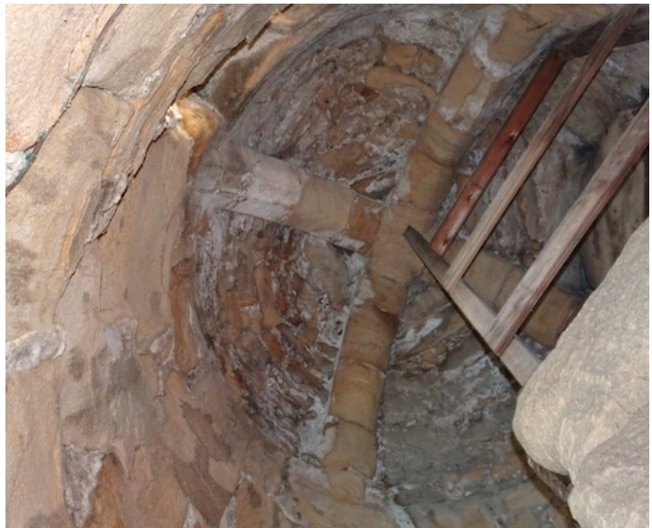
Tower staircase – eroded stone, open joints and salts at roof soffit
