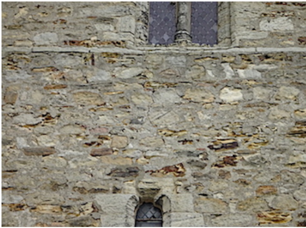
Tower south face - crack in masonry at ringing chamber level
