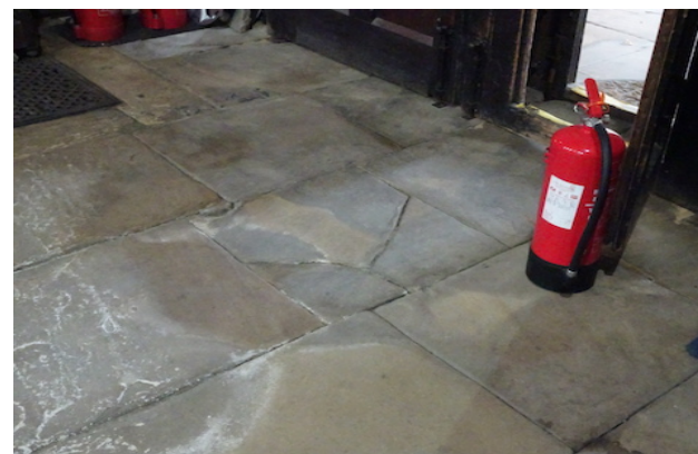
South Aisle – rising damp and cracked flags near south door
