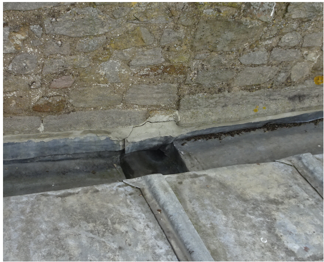
Tower roof – cracked mortar to cover flashing on west parapet wall
