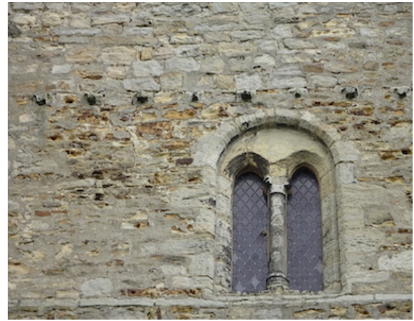
Tower south face - eroded pockets in masonry
