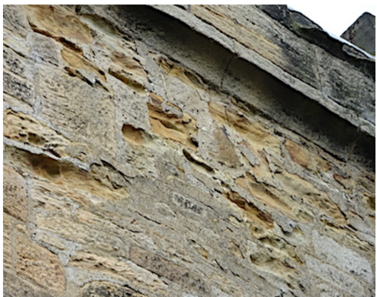
South Transept – eroded stonework and pointing on east wall high level
