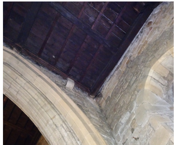
South Aisle – damp penetration at east end at eaves.
