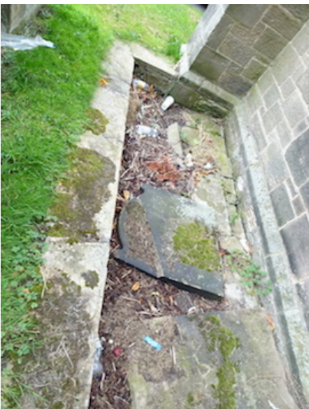
South Chancel wall – debris in perimeter gutter
