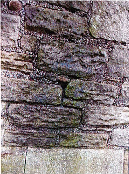
S Transept - open joints between hopper and top of buttress.
