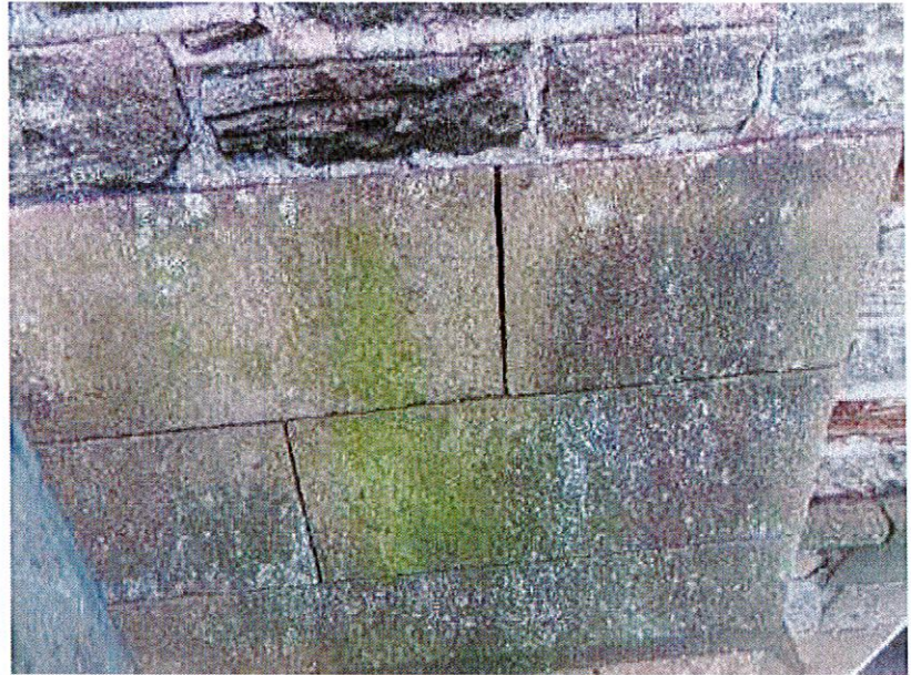
N Transept similar and open joints in top of buttress
