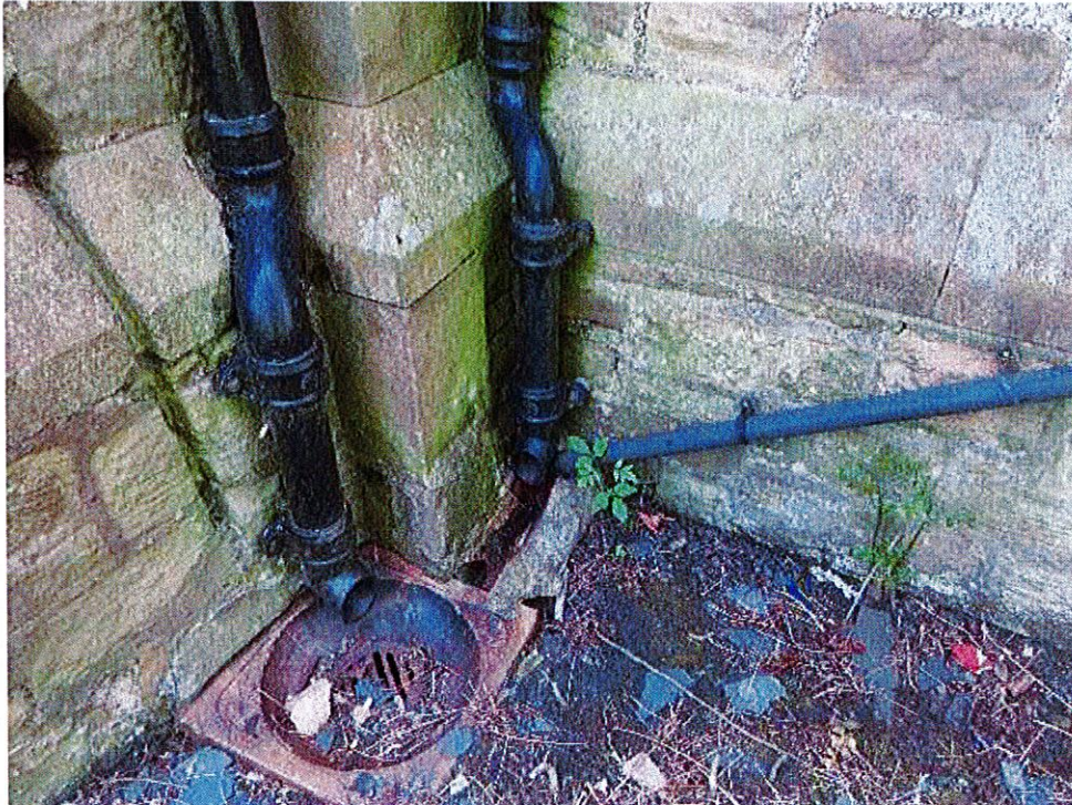
At corner of Sanctuary and Sacristy hole in concrete ground channel wets ground at base of wall
