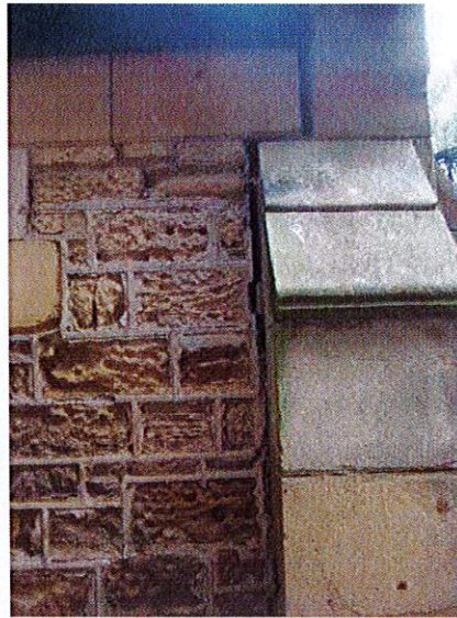
Crack at SW of Porch 2013
