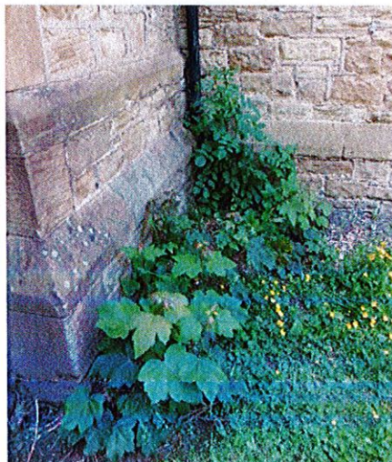
SW Choir – gully cracked and overgrown
