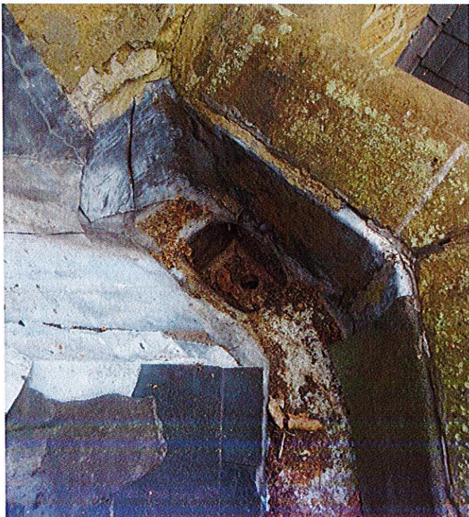
para 23 – loose flashing at E corner of Office
