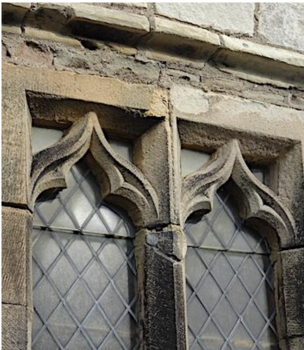
15. South Nave clerestory wall - open joints to window stonework.
