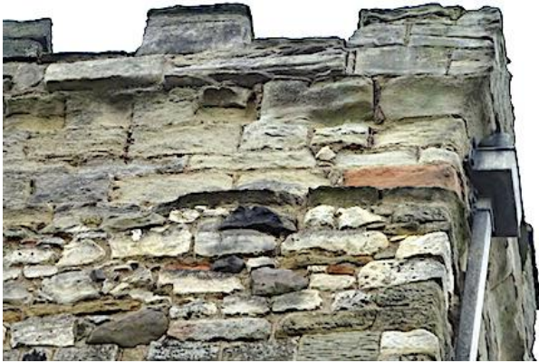
11. Tower parapet wall showing eroded stonework and open joints.
