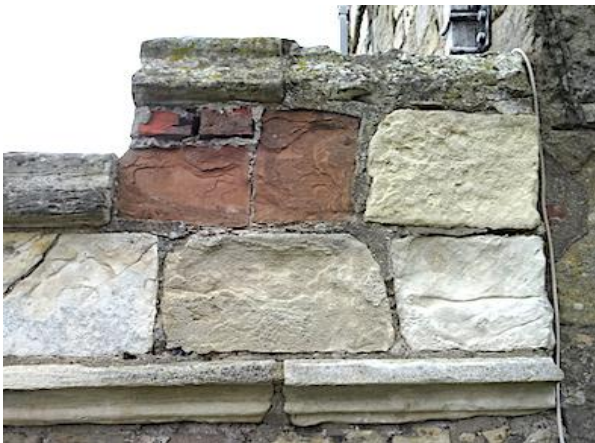
13. North Nave parapet wall next to Tower - open joints.
