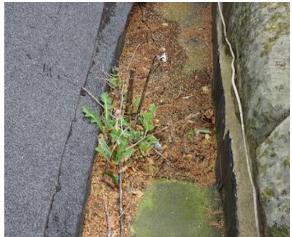
6. South Nave Aisle roof showing blocked gutter
