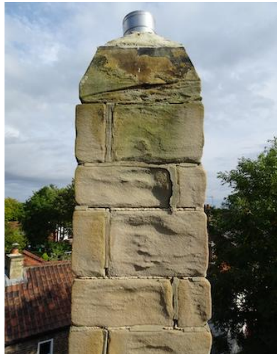
16. Boiler room chimney stack above Meeting Room - open joints
