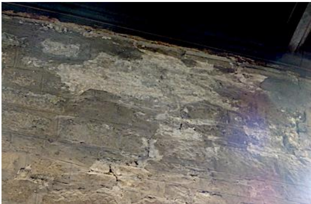
25. North Nave upper level – eroded stonework surfaces
