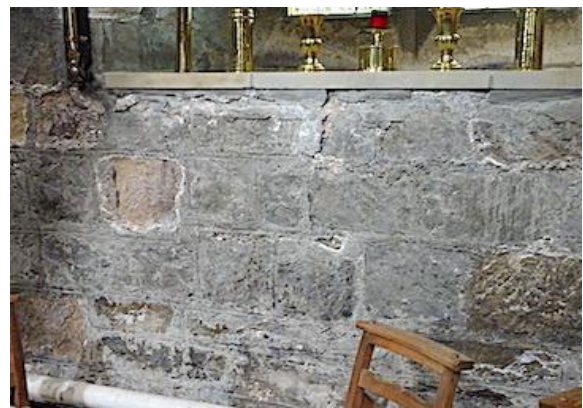
26. North Nave north wall – erosion and slats at low level
