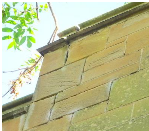
20. West wall coping of Meeting Room – open joints
