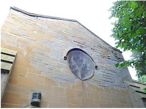
17. West gable of West Transept showing eroded stonework at top
