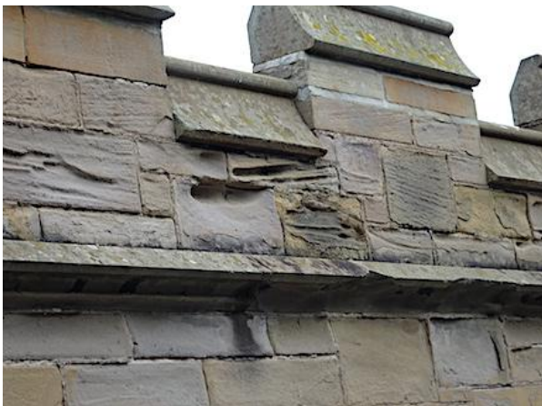
9. South parapet wall of Chancel showing eroded stonework.
