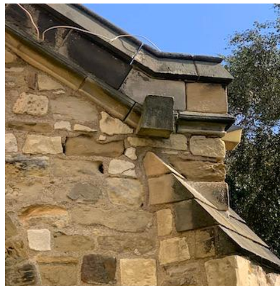
22. West face of South Aisle – open joints and eroded stones
