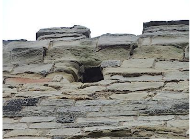
12. Tower parapet wall - deeply eroded stonework and open joints.
