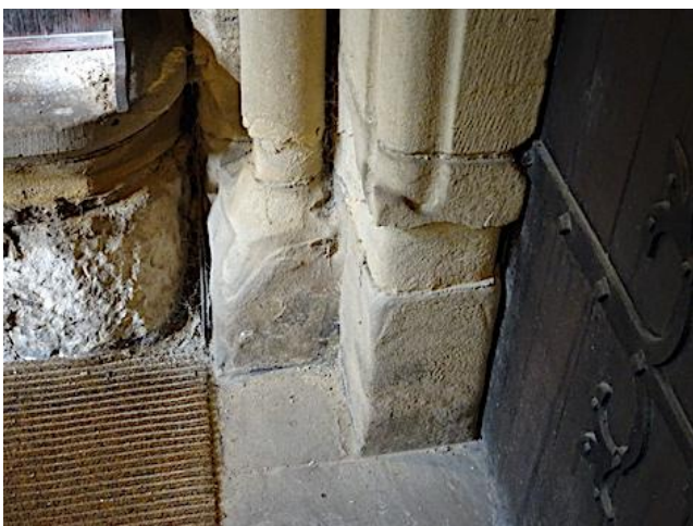
27. South Porch – eroding stone base and shafts of entrance archway
