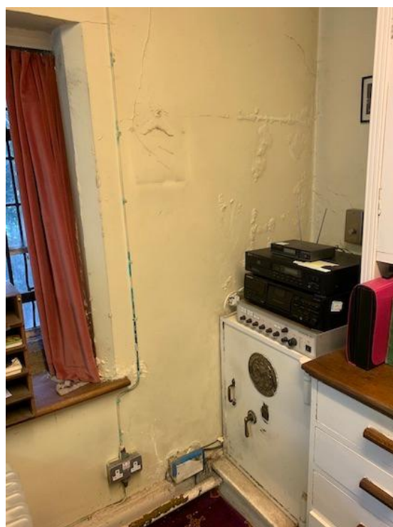
31. Vestry east wall south corner – numerous plaster defects
