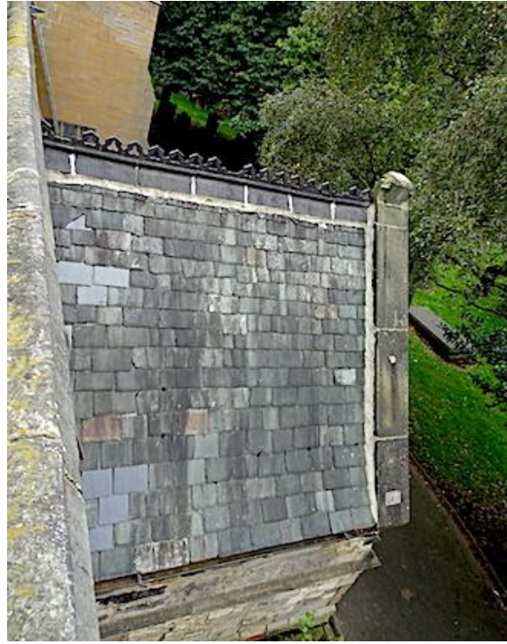
2. South Porch roof showing condition of slates
