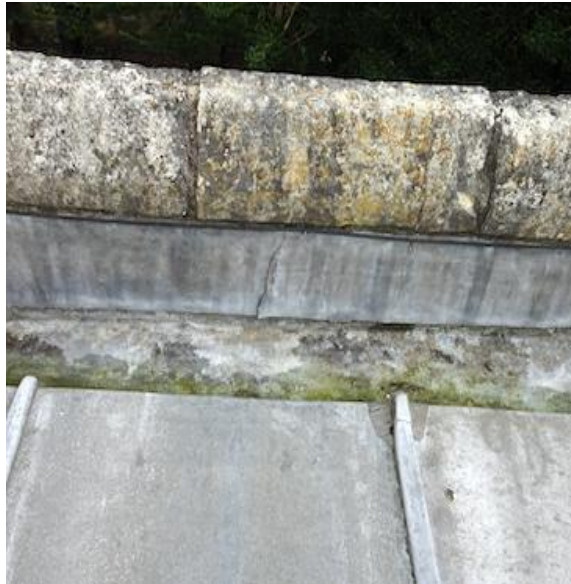
4. North Aisle roof showing open parapet joints & torn flashing
