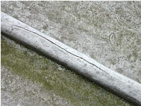
7. Typical split to top of lead rolls on North Aisle roof
