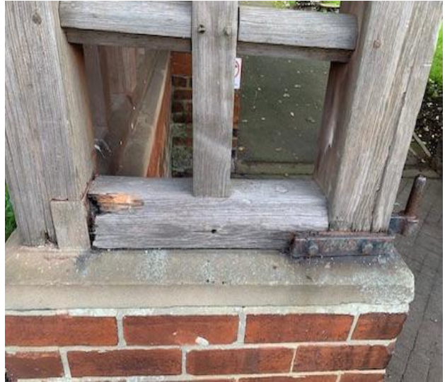
24. Lych Gate showing rotten soleplate timbers and rusty ironwork
