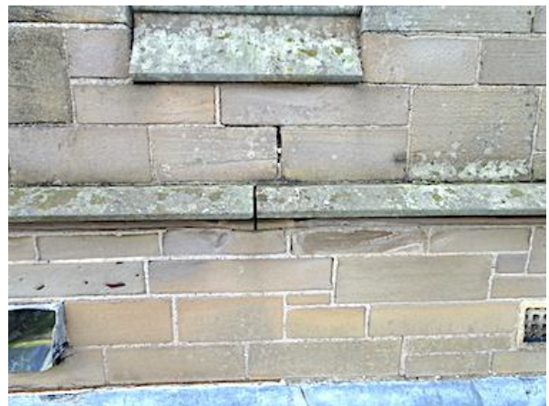
10. South parapet wall of Chancel showing movement in stonework.
