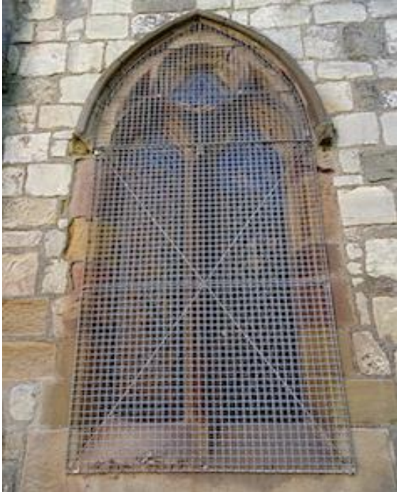
23. North Aisle window – eroded stone surrounds and tracery
