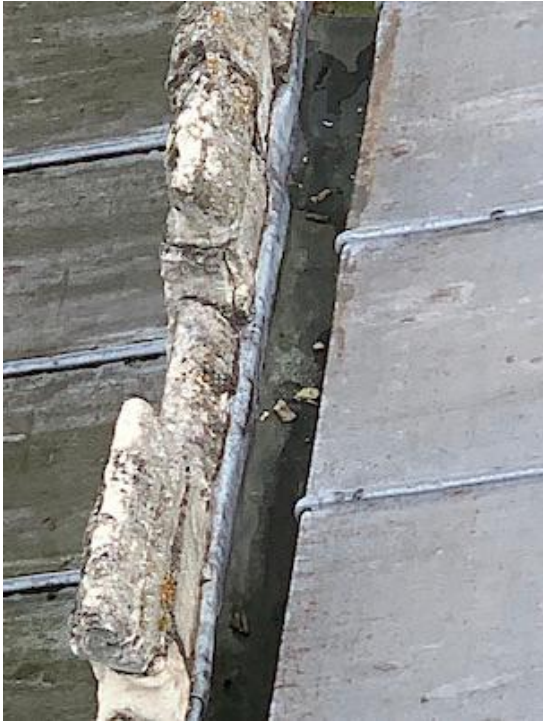
1. Nave roof south slope gutter – detached parapet stone.
