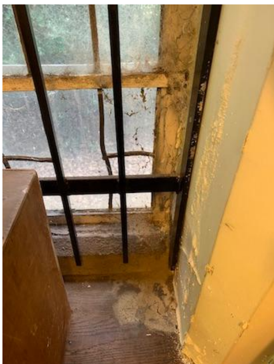
30. Vestry southeast window – buckled lead to panel
