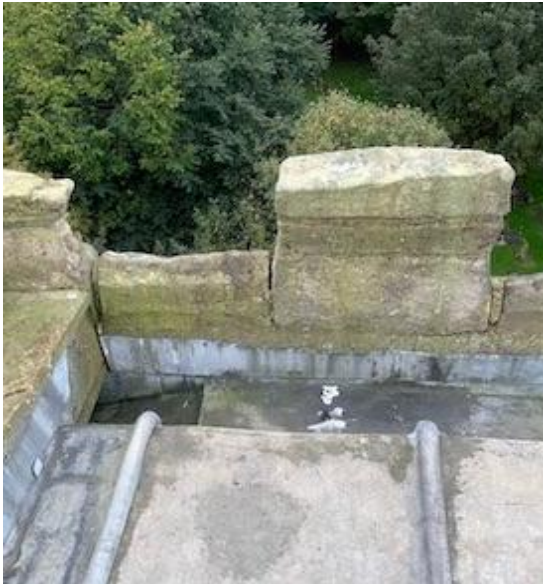
3. Tower roof showing open parapet joints
