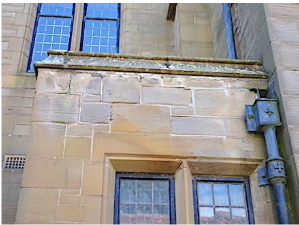
19. North face of North (Vestry) Entrance Lobby – poor pointing
