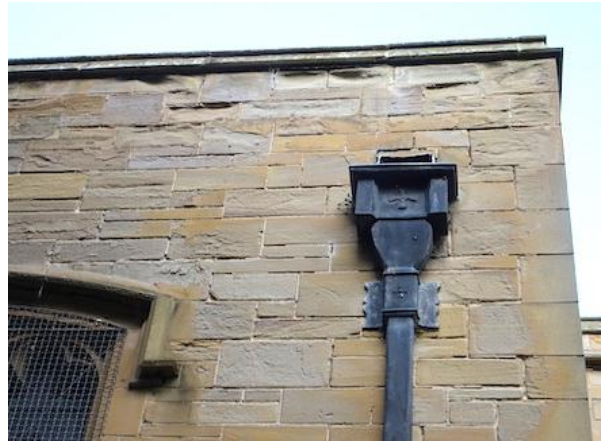
18. West end of south Chancel showing eroded stonework at top
