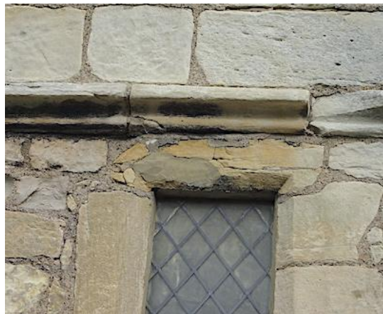
14. North Nave parapet wall next to Tower - open joints.
