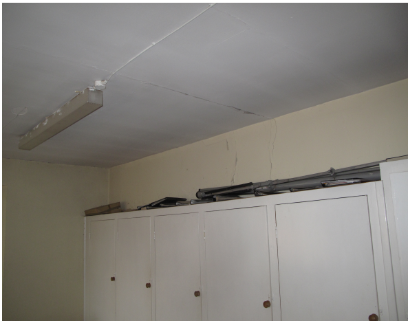
38 Meeting Room – cracks on east wall
