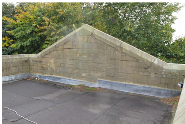
11 South Transept Roof – displaced stonework and open joints
