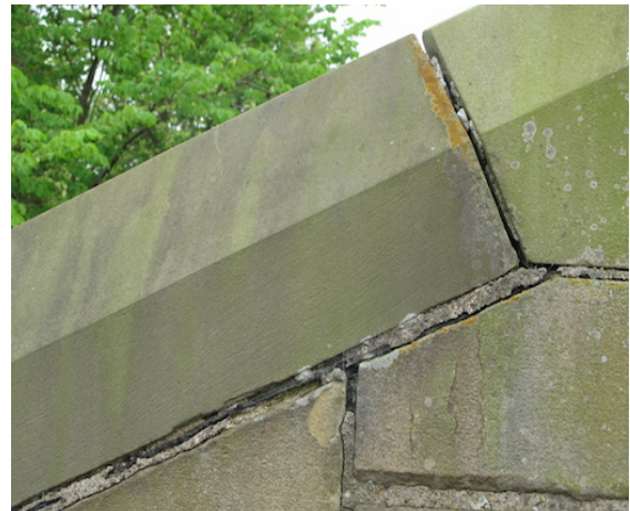
15 South Transept gable – displaced stonework / open joints
