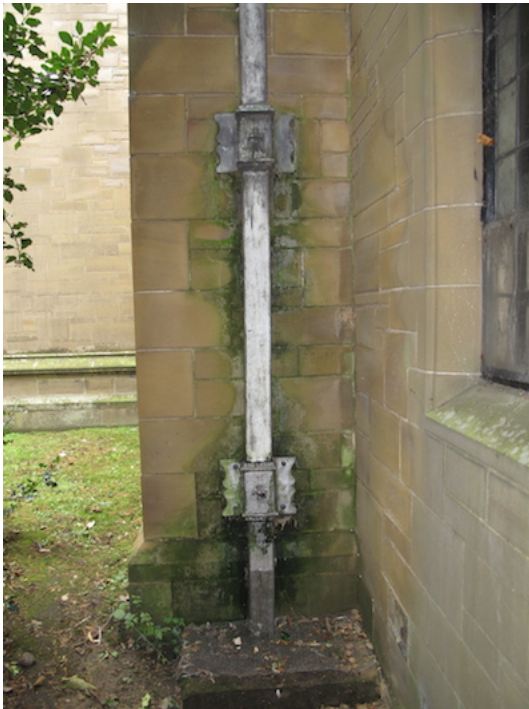
18 Vestry north side – overflowing rainwater pipe at east
