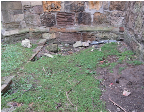
22 North Nave Aisle at west end – unprotected pipes
