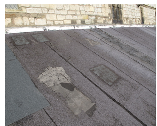
06 South Aisle roof – condition of felt coverings
