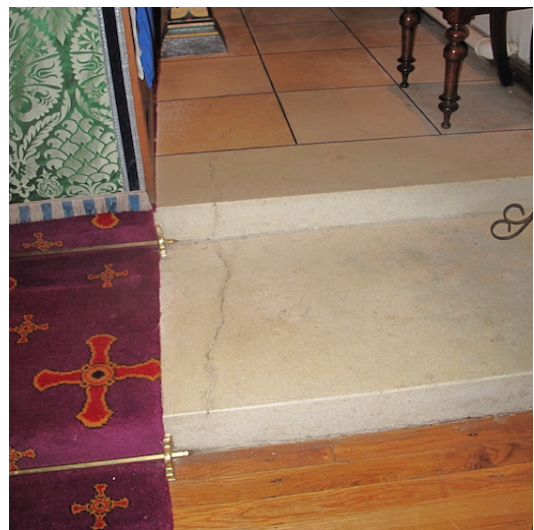
31 Sanctuary – crack in terrazzo floor
