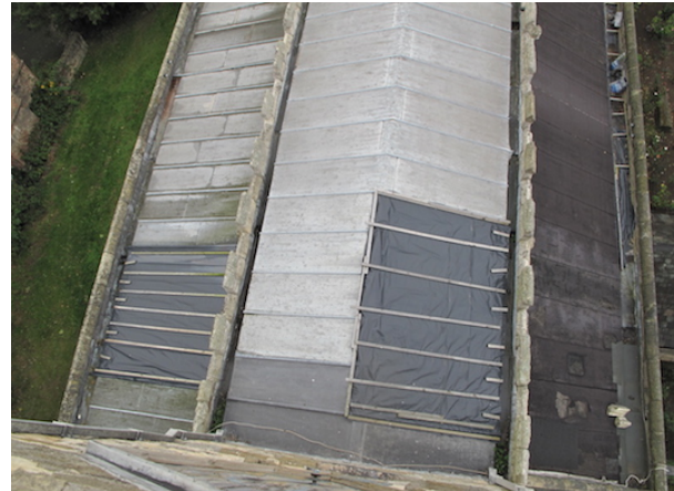
02 Nave roof at west end showing stolen areas of lead
