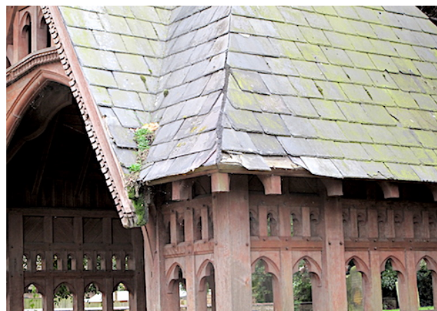
23 Lychgate – damaged roof at north east corner
