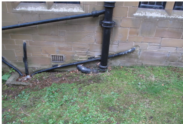
21 Vestry west wall – low ground level covering pipe junction
