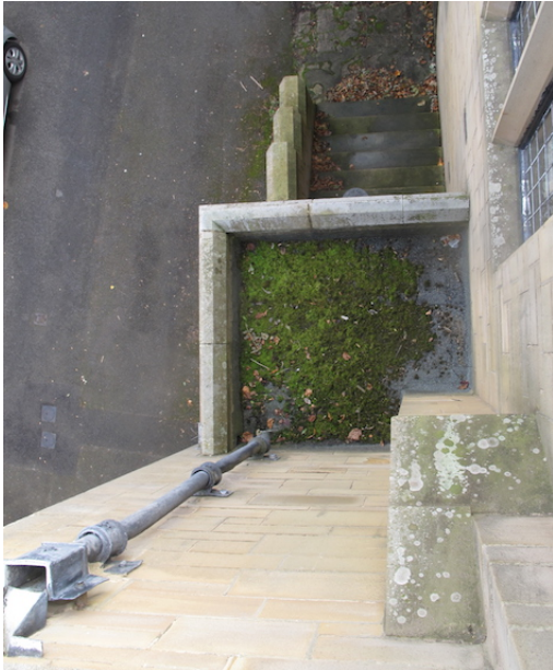
12 Vestry Porch Roof – moss covered
