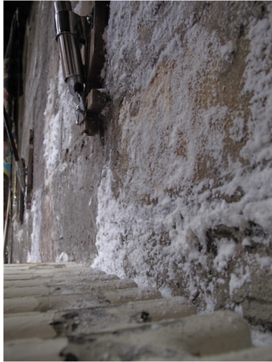
35 North Nave Aisle – salts above radiator, detail
