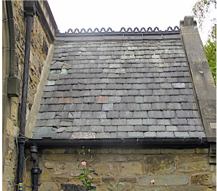
13 South Porch Roof – defective, slipped and missing slates
