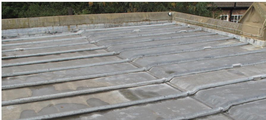
09 Meeting Room Roof – lead roll patches
