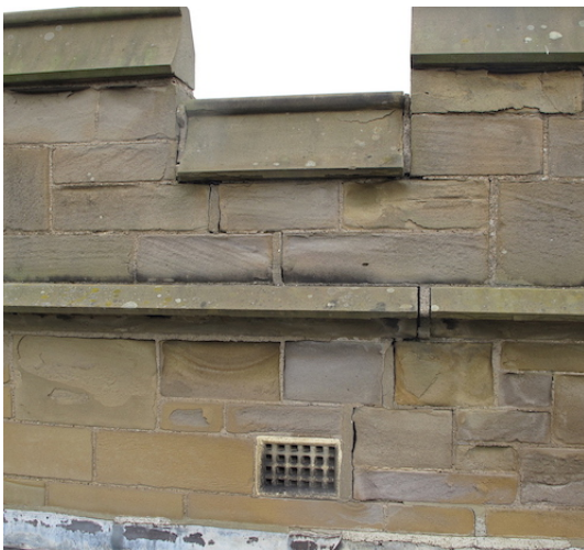
16 Chancel clerestory wall – structural movement
