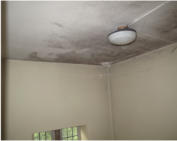
36 Meeting Room access stair void – damp signs on ceiling
