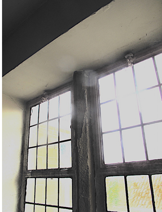
35 Meeting Room – eroding stone mullion
