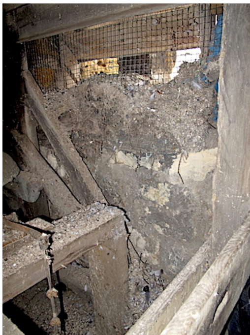
26 Belfry window opening covered in guano
