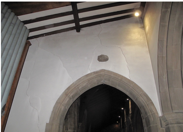
32 South nave Aisle west side – various cracks
