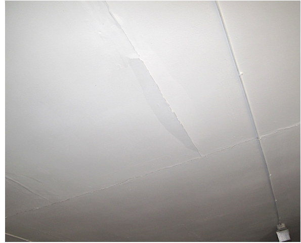
37 Meeting Room – disturbances in ceiling
