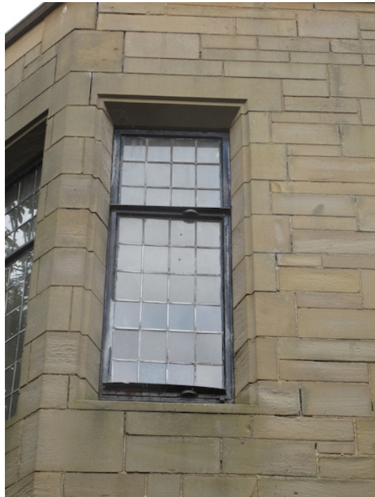
19 Vestry first floor – buckled steel window
