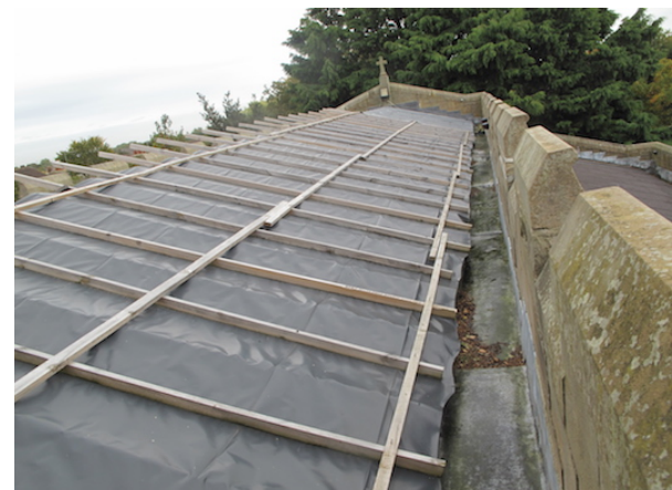
04 Chancel Roof south slope – showing stolen area of lead
