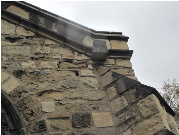
14 South Porch Roof – eroded stonework and open joints
