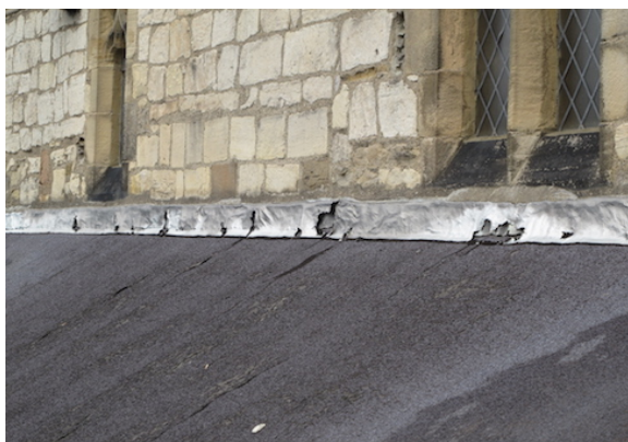
10 South nave Aisle Roof – defective flashings
