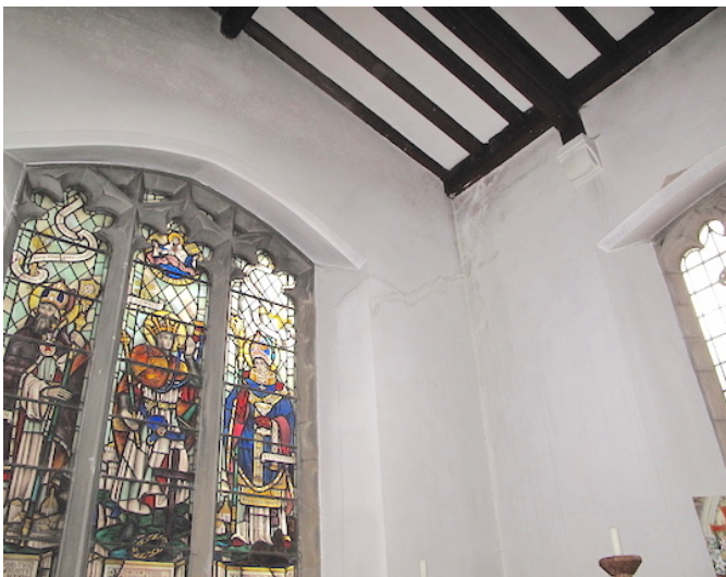
30 Lady Chapel – south east corner possible damp
