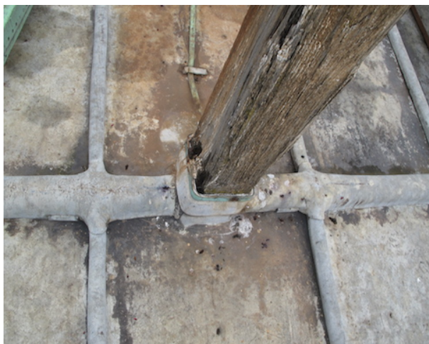
05 Tower Roof – rotten section of timber flagpole at base
