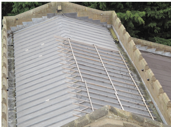
03 Chancel Roof – showing stolen area of lead
