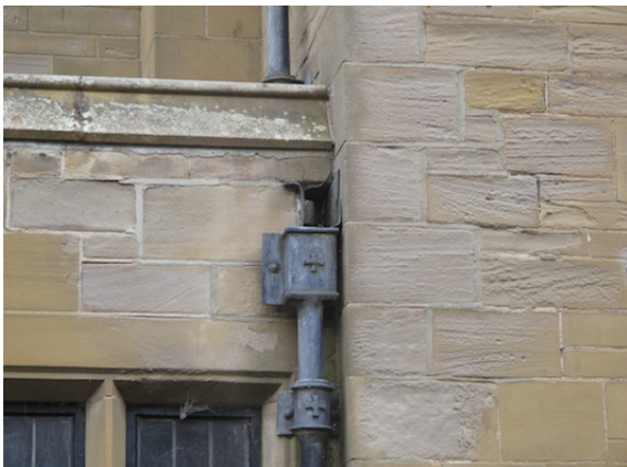
20 Vestry north porch side – overflowing hopper
