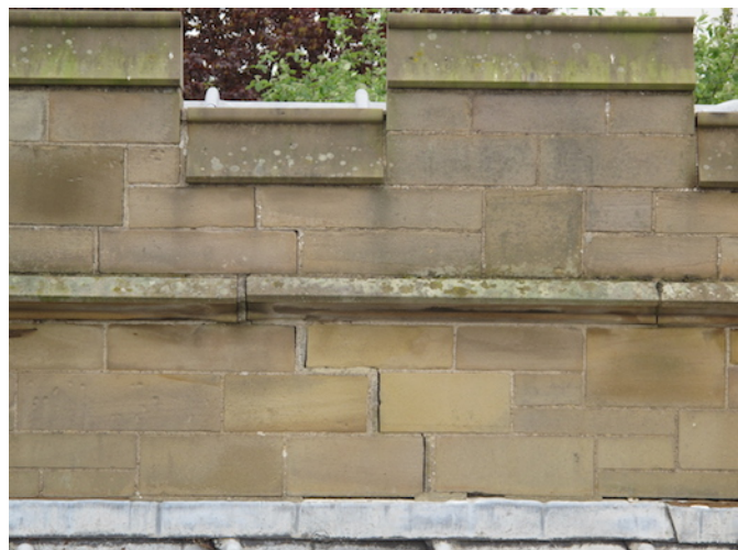
17 Chancel clerestory wall north side – structural movement
