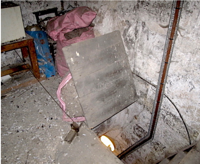
28 Clock Chamber – access point, no grab bars
