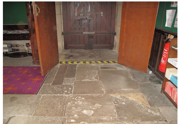
33 South Porch – damaged flags
