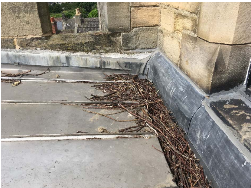
Photo 7 Jackdaw twigs blocking gutters below Tower.
