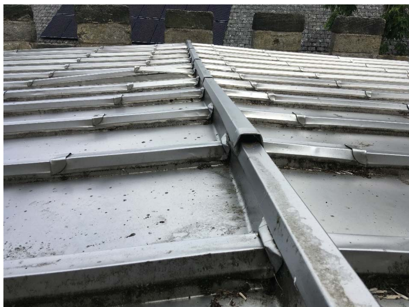
Photo 10 Close up of 2No. loose SS capping pieces.
