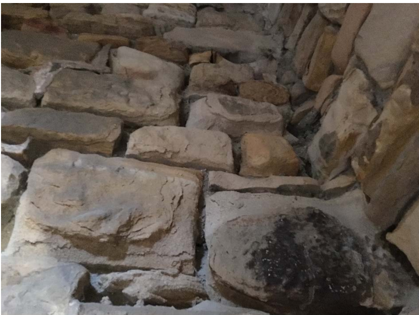
Photo 4 Eroded mortar and masonry within Belfry.
