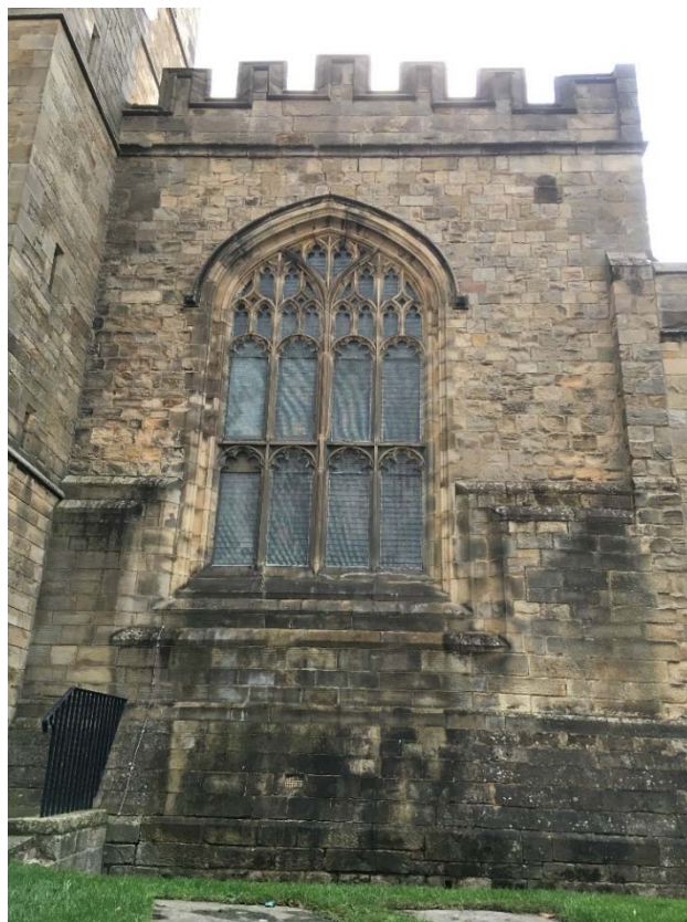
Photo 12 Nave west elevation with cracking and settlement north side.
