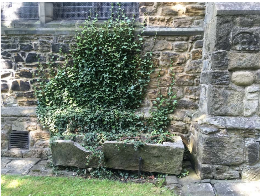
Photo 25 Ivy growth on South Transept
