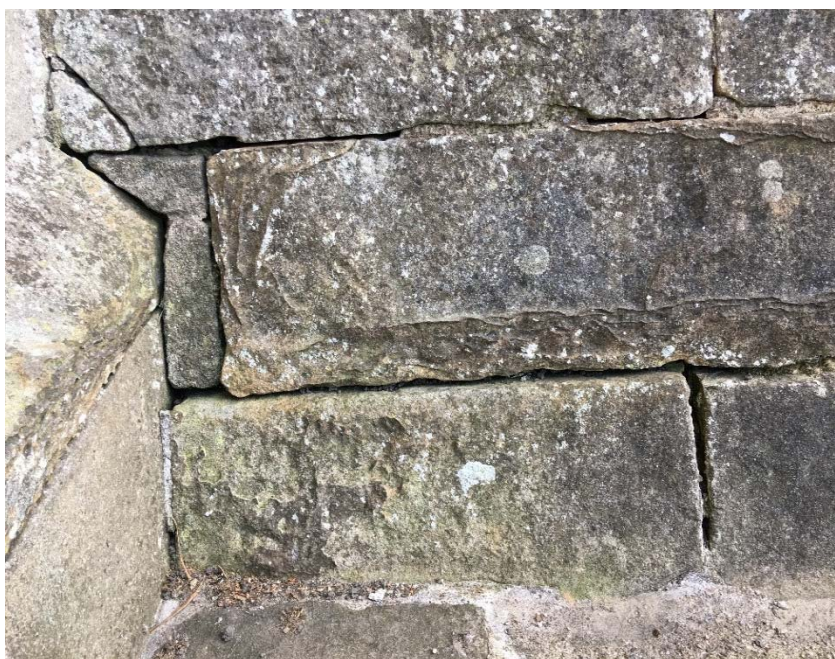
Photo 13 Missing pointing and loose stone below west window.
