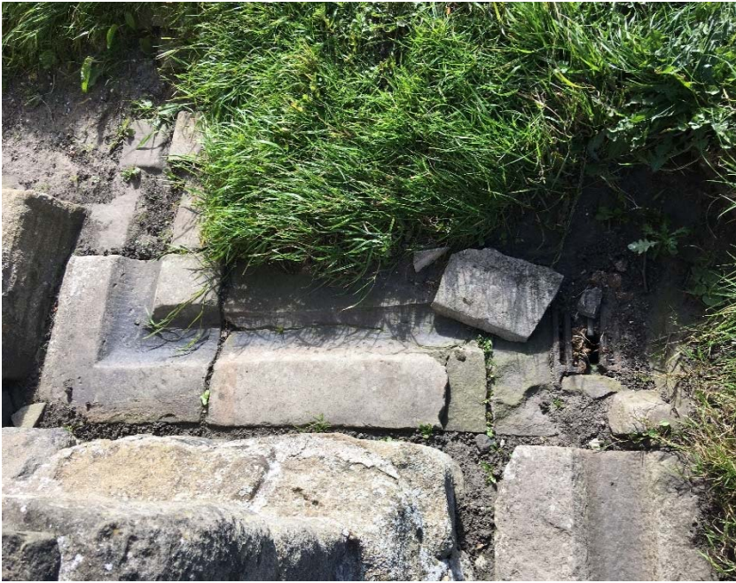
Photo 23 Broken and uneven stone channel drains.
