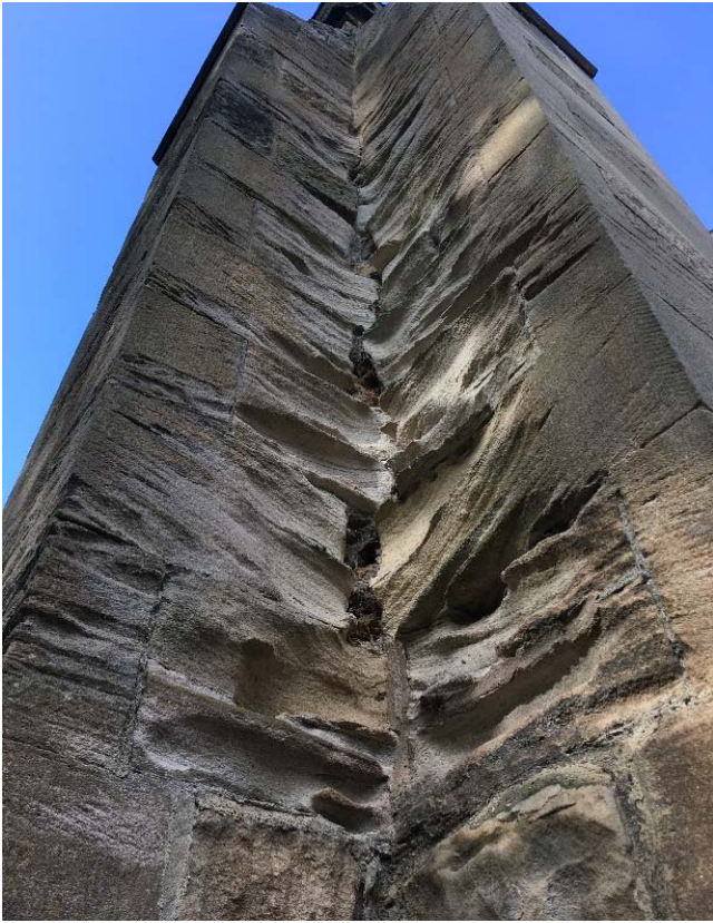
Photo 14 East buttress on South Transept is severely eroded.
