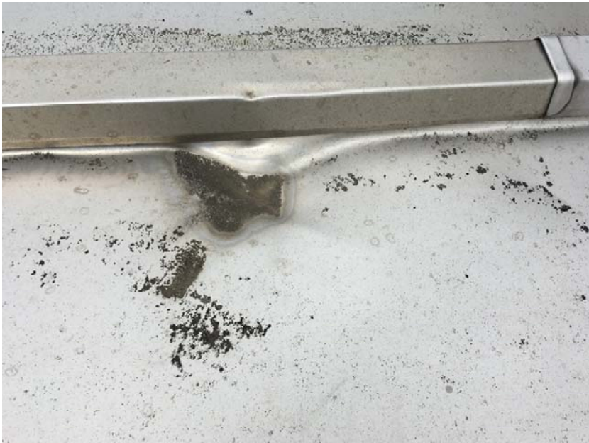
Photo 6 Indent damage on SS sheets above Nave.
