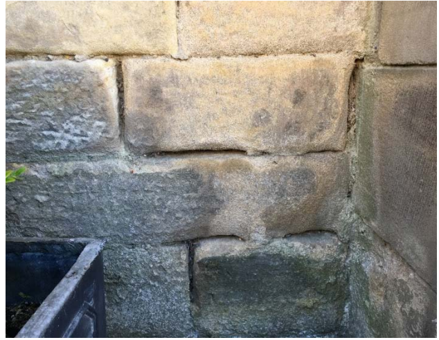
Photo 15 Missing pointing on north side of Tower.
