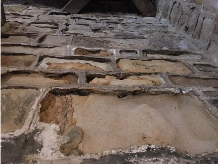
Photo 5 Eroded masonry behind cement pointing in Belfry
