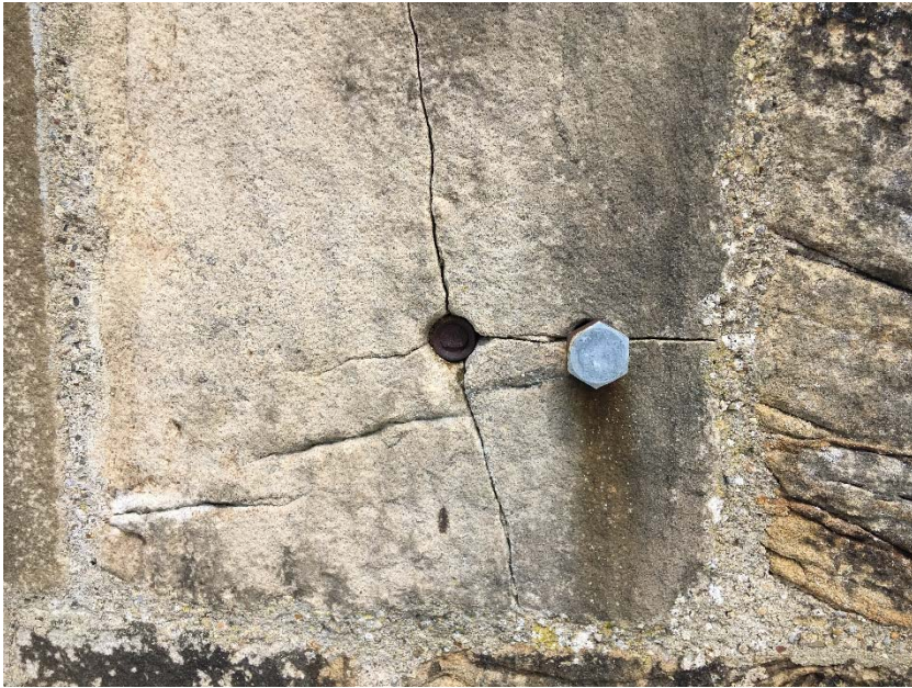
Photo 17 Corroding scaffold plugs are cracking masonry.
