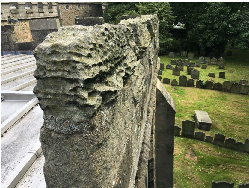
Photo 18 Severely eroded merlon on South Transept
