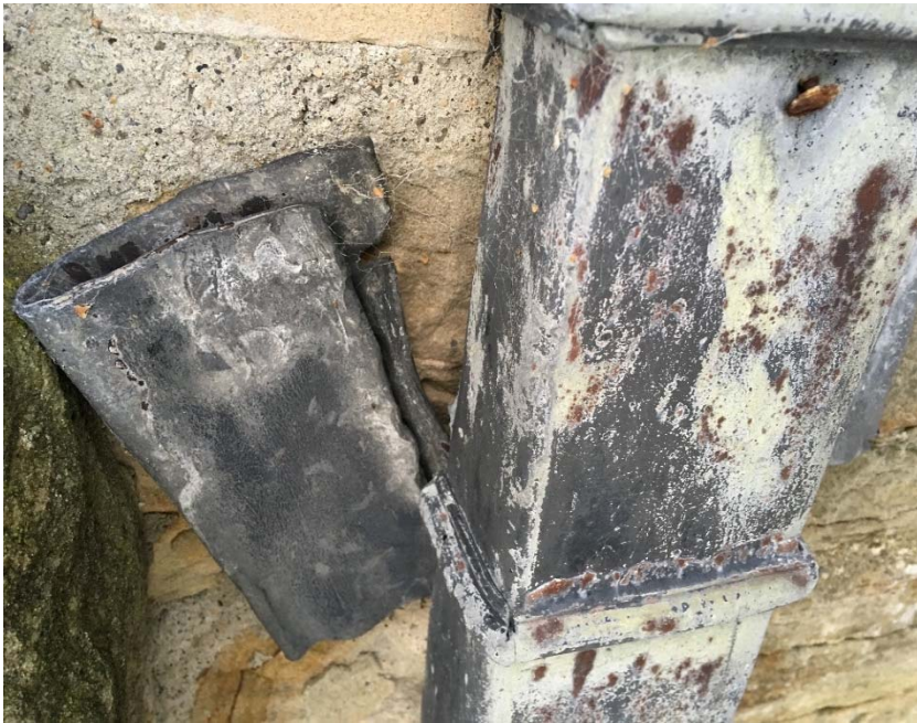
Photo 21 Torn and holed lead RWP on south clerestory.
