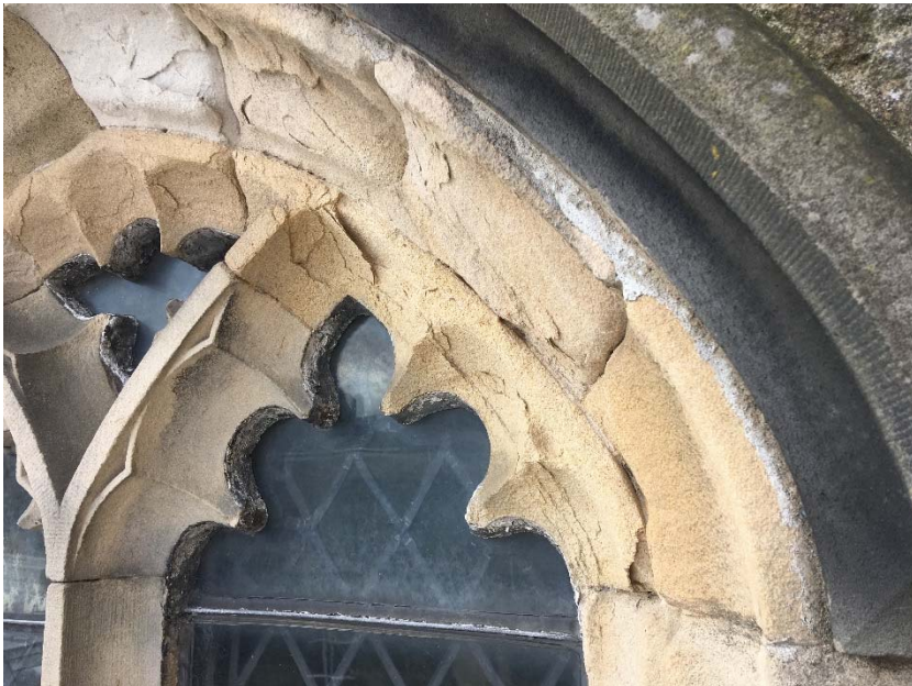
Photo 16 Eroded tracery on Nave south clerestory.
