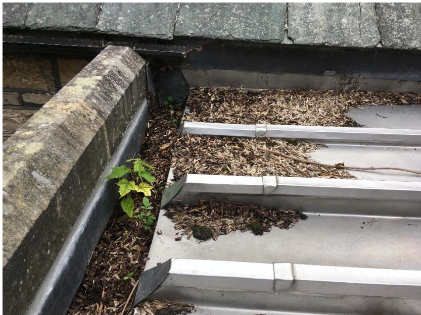
Photo 8 Ash keys and plant growth above North Chapel.
