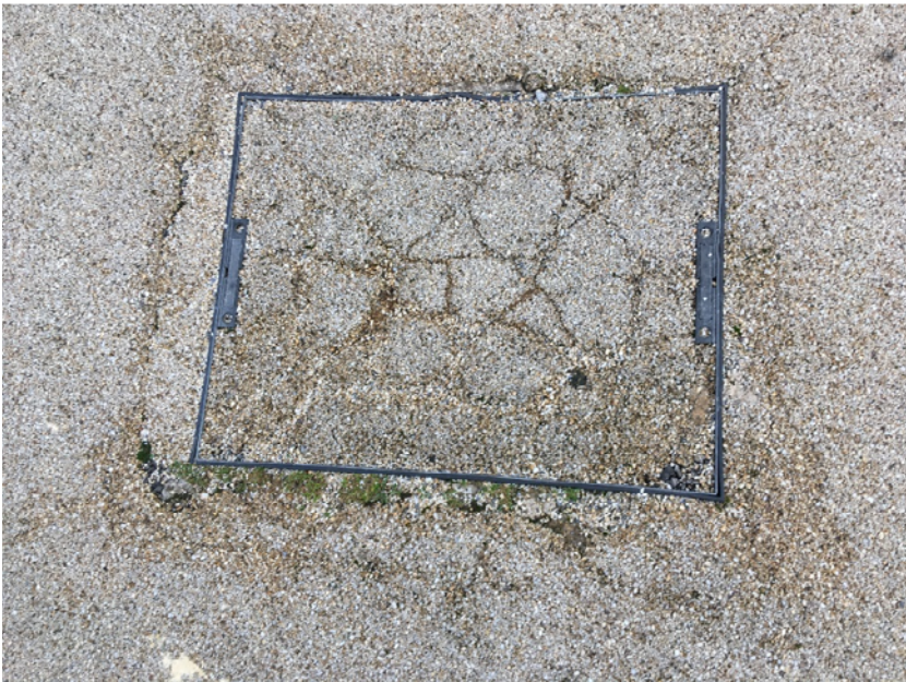
Photo 24 Cracked resin surfacing on car park.
