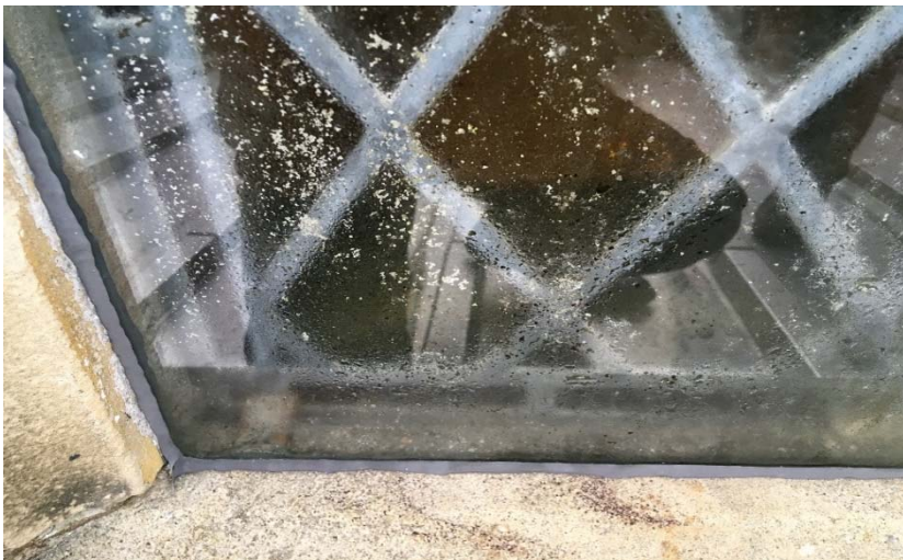
Photo 22 Silicone sealed external glazing is trapping moisture.
