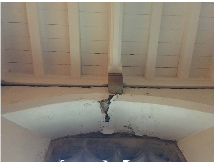
Photo 28 Water ingress above North Chapel.
